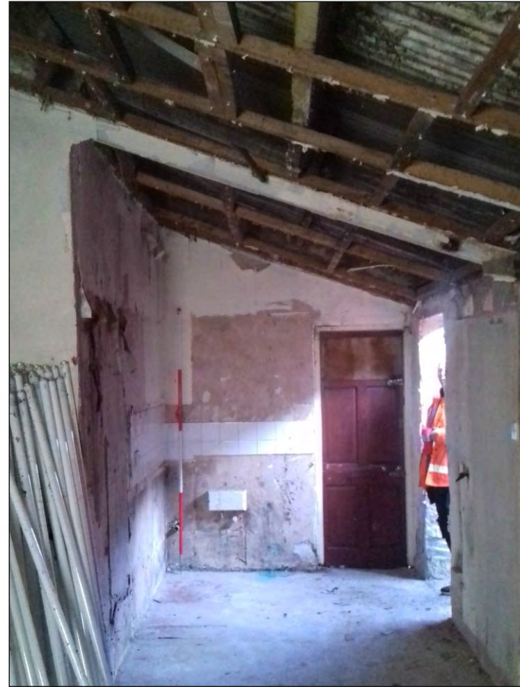
Pl. 7 General view of rear elevation of No. 80a Ebrington Street. 2m scale. Looking north.
