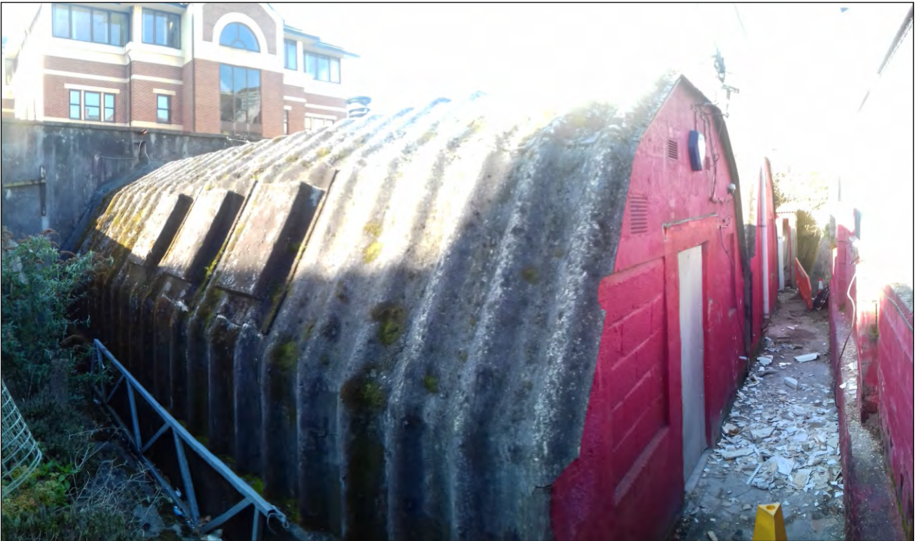
Pl. 2 General view of rear elevation of 80-82 Ebrington Street clearly showing the Handcraft Hut design. Looking southwest.
