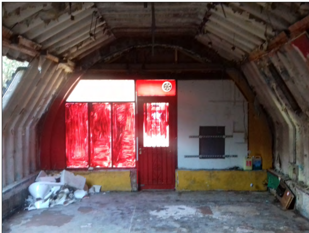
Pl. 5 General view of front elevation of No. 80 Ebrington Street. 2m scale. Looking south.
