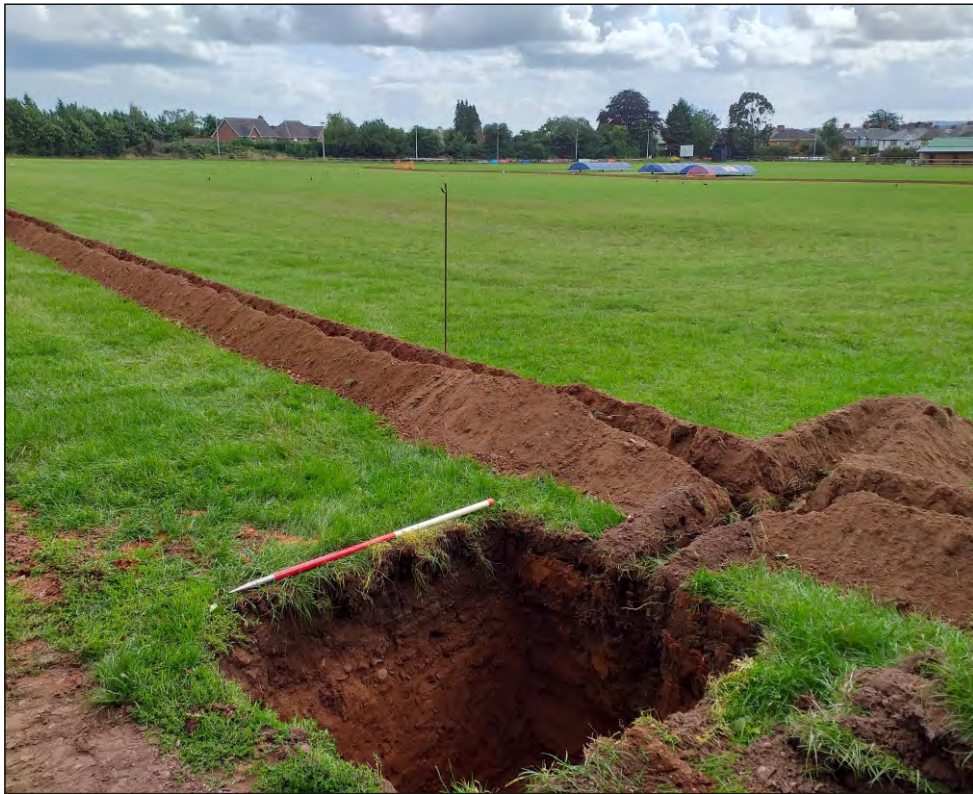
Pl. 1 General view of cable trench with Pit 4 in foreground. 1m scale. Looking south.
