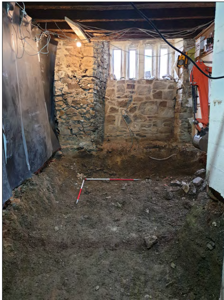
Pl. 2 General view of Room G04 showing reduced level. 1m scales. Looking northwest.
