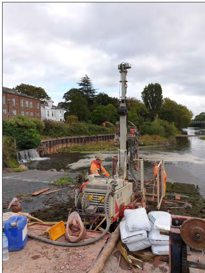
Pl. 2 General view of the rotary rig positioned on Trews Weir, excavating borehole 2. Looking southeast.
