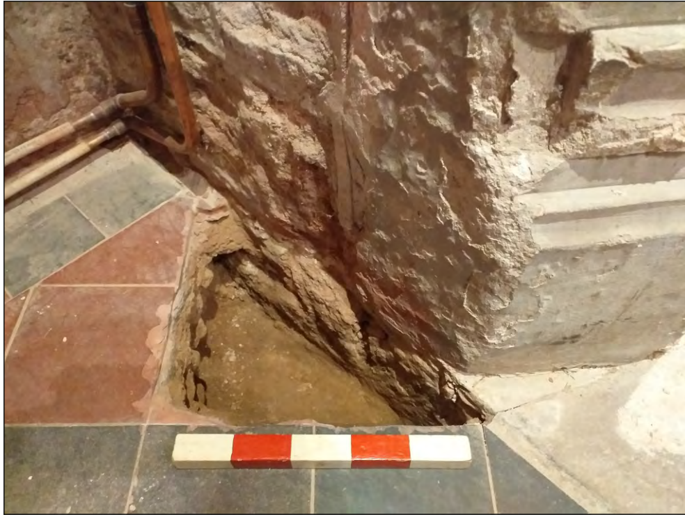
Pl. 1 General view of Trench 1 showing projecting footing (103) of north wall of north aisle. 0.25m scale. Looking southeast.
