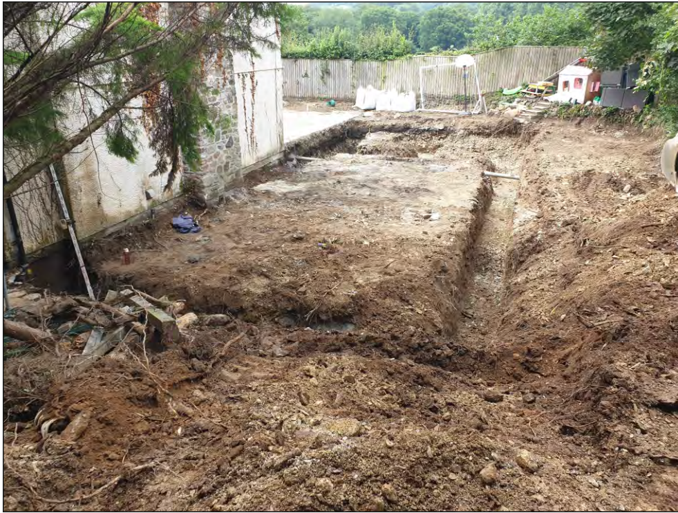
Pl. 1 General view of the foundations showing the possible mining waste stone. Looking north.
