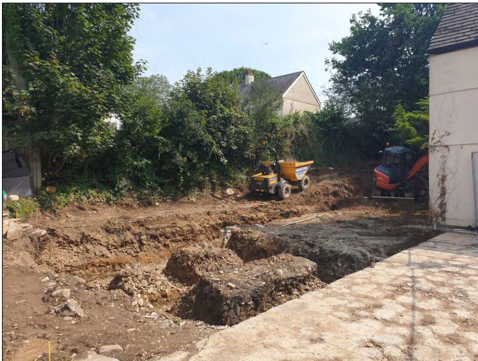
Pl. 2 General view of the foundations showing the possible mining waste stone. Looking south.
