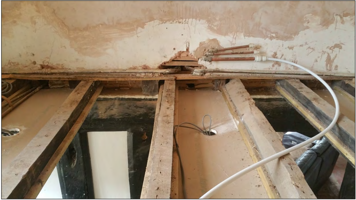
Pl. 22 Close-up showing 19th century floor joists resting on thin timber fillet above passage head-beam. Looking south.
