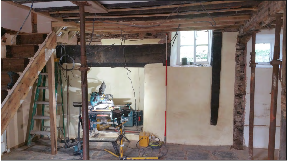
Pl. 11 General view of west elevation of former hall showing lateral fireplace and later window. 2m scale. Looking west.
