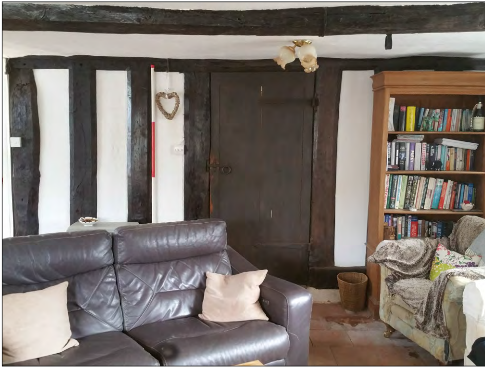
Pl. 5 General view of south elevation of passage screen showing replaced muntin. 2m scale. Looking north
