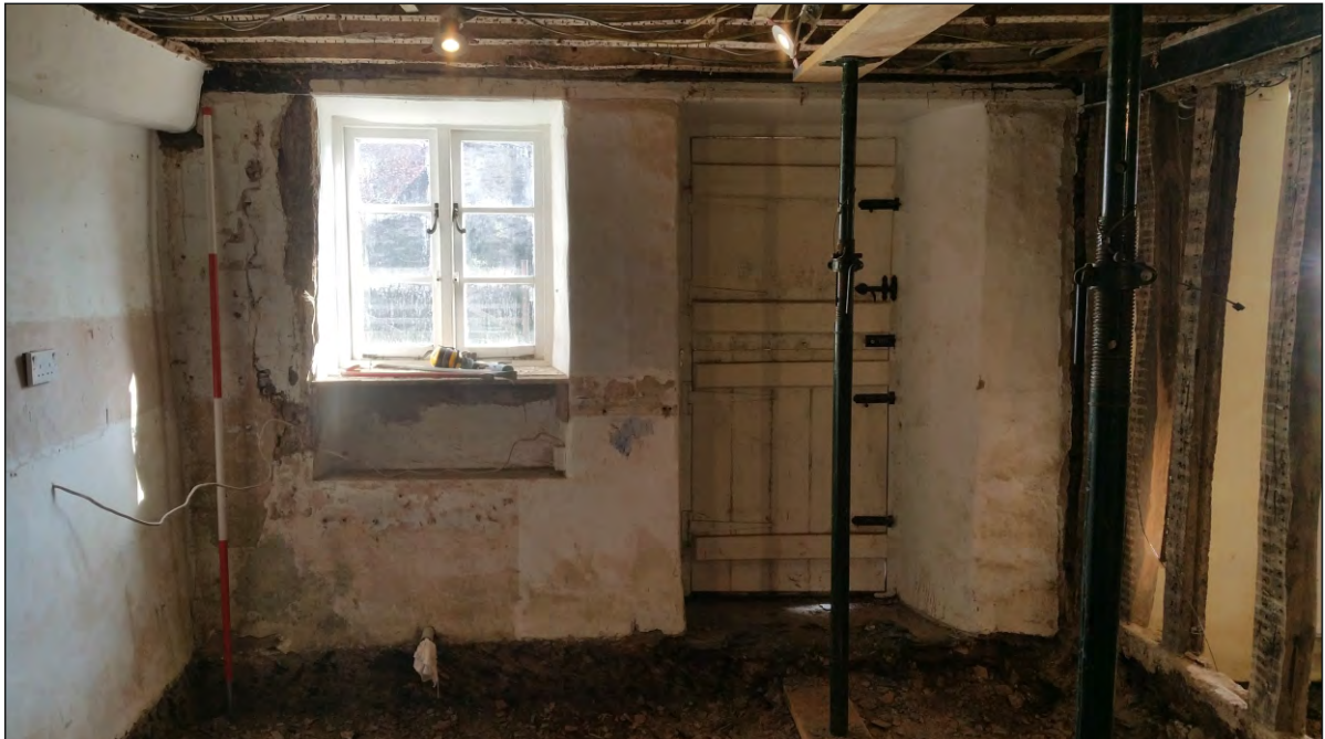
Pl. 12 General view of east elevation of former hall showing later window and doorway. 2m scale. Looking east.
