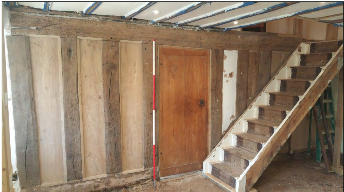
Pl. 4 General view of the plank-and-muntin screen showing the replaced planks and the construction of the floor of the hall in relation to the earlier screen. 2m scale. Looking southwest.
