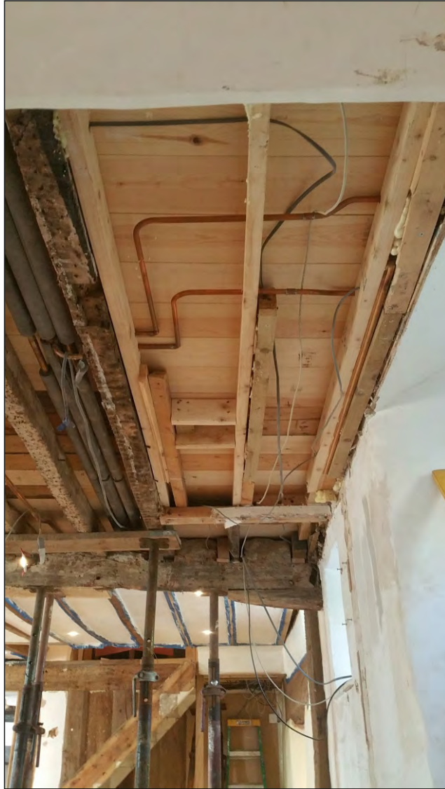
Pl. 17 General view of first floor ceiling in the kitchen showing location of former staircase. Looking south.
