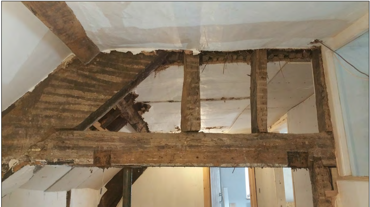
Pl. 23 Close-up of secondary brace showing lap joints for later partition. Looking south.
