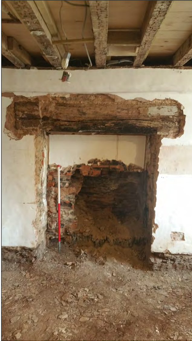
Pl. 15 General view of fireplace in north elevation of former inner room. 1m scale. Looking north.
