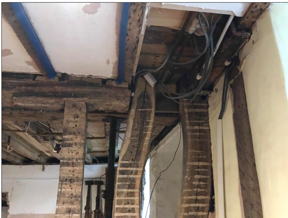
Pl. 14 Close-up of east end of screen showing 19th century 'repairs'. Looking north.
