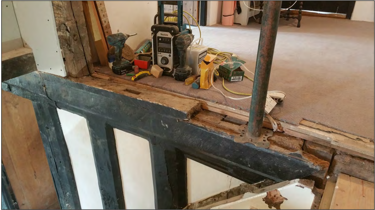
Pl. 19 General view of passage head-beam showing arrangement of earlier floors and partitions. Looking southeast.
