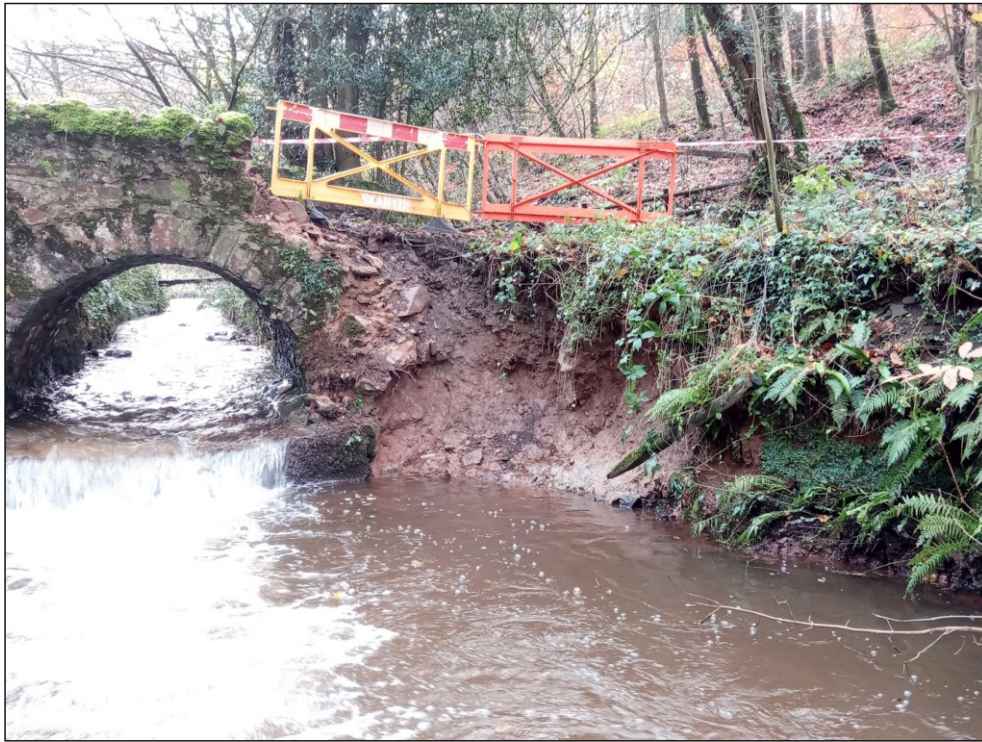
Pl. 1 General view of damaged west wing wall. Looking south.
