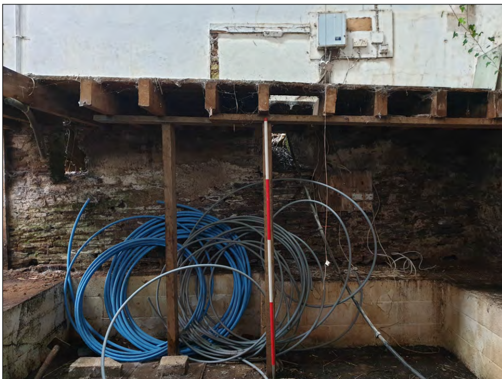
Fig. 12 General view of northern ground-floor bay showing two slit windows with splayed jambs in west elevation. 2m scale. Looking west.
