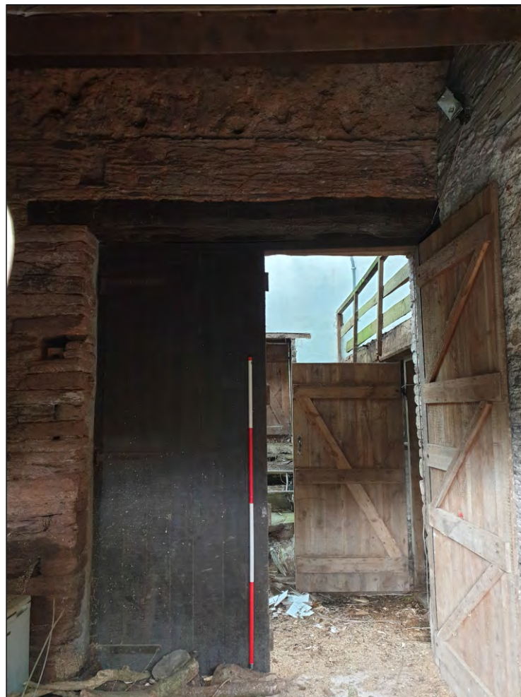
Pl. 8 General view of double door in east elevation showing cob walling above the original stone rubble. 2m scale. Looking southwest.
