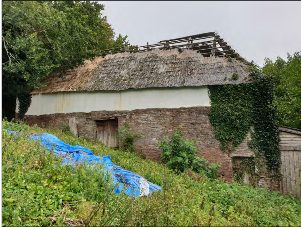
Pl. 7 General view of the west elevation showing the original roof height. Looking northeast.
