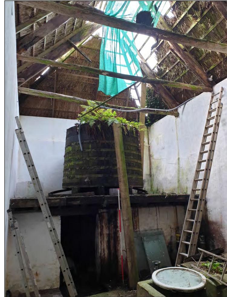
Fig. 10 General view of south end showing mid-late 19th century ground-floor partition with modern opening and heavily rebuilt floor structure. 2m scale. Looking south.
