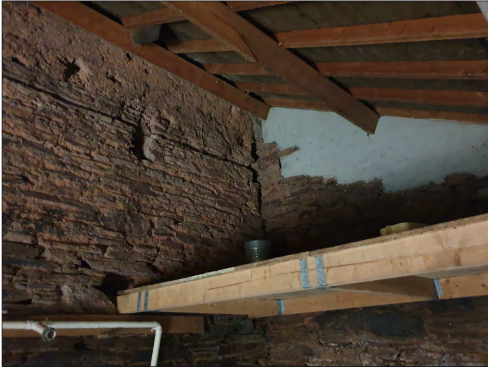
Pl. 3 General view of earlier roofline of extension below cob extension of barn and original height of north end wall. Looking northwest.
