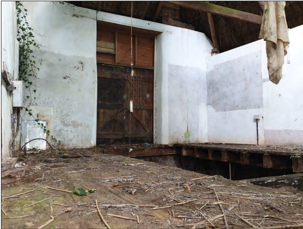
Fig. 15 General view of first floor showing former height of wall with extended double door in north elevation. Looking north.
