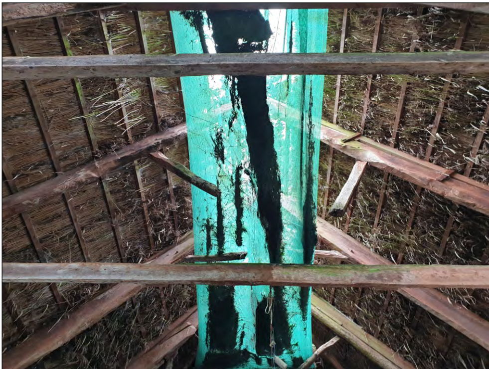
Fig. 16 General view of roof structure showing trusses with pegged collars, modern tie beams and thatching battens. Looking north.
