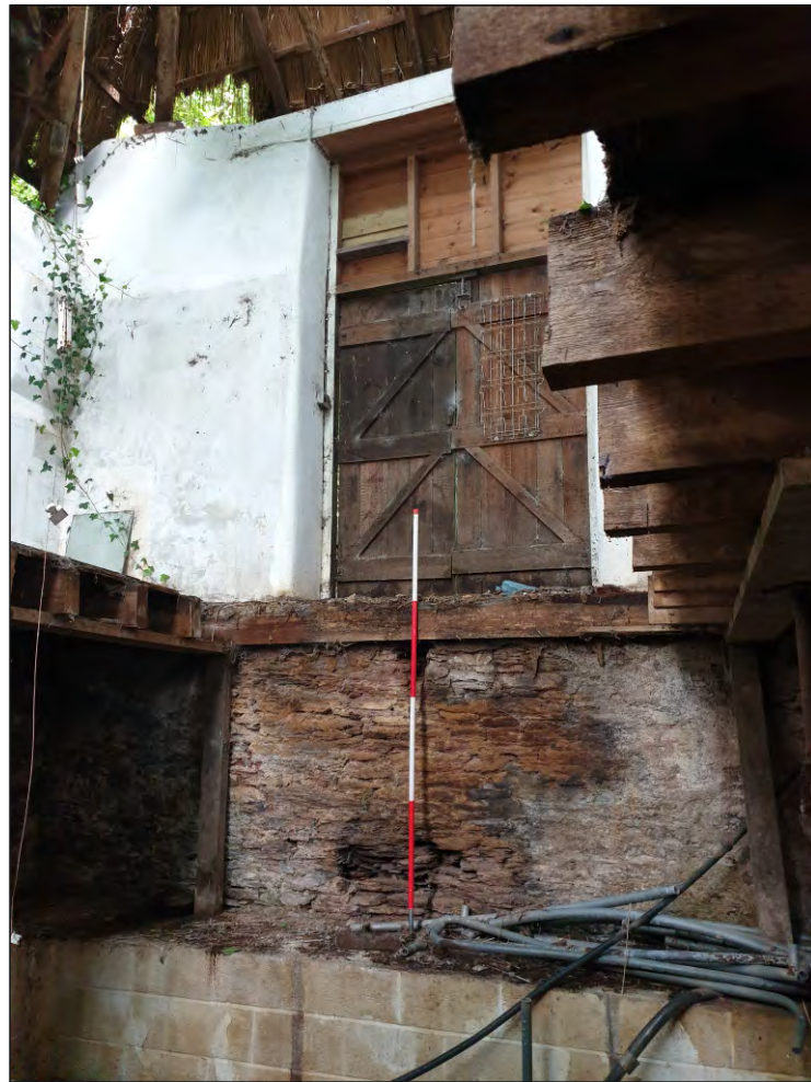
Pl. 14 General view of north bay showing extensive modern truncation of ground- and first floor. 2m scale. Looking northwest.
