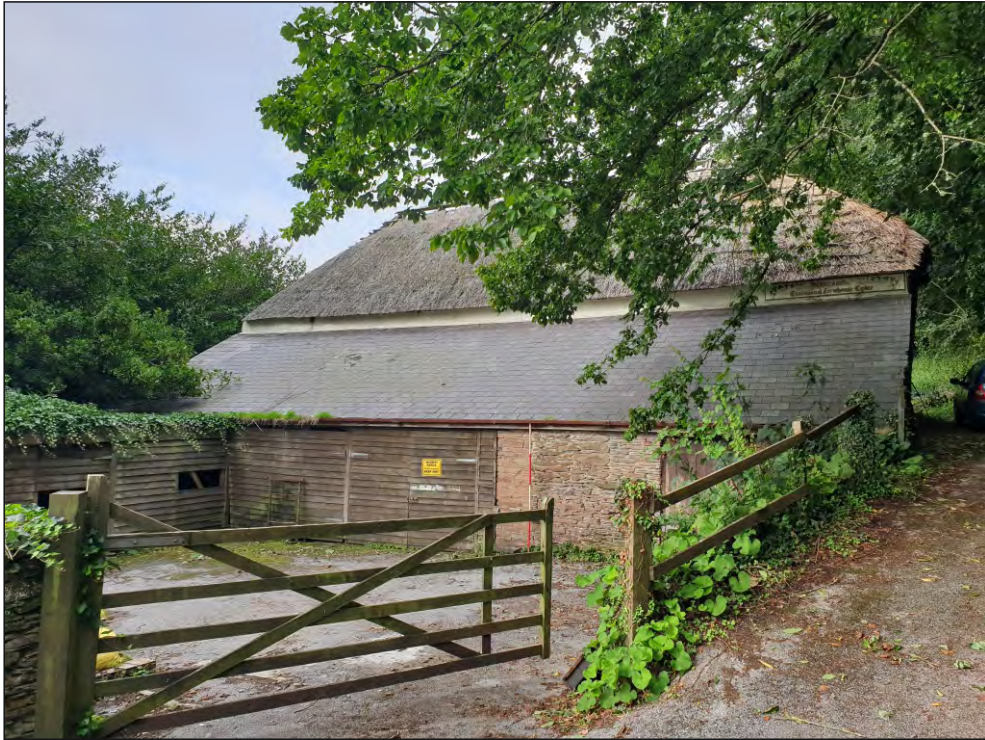
Pl. 1 General view of east elevation showing 19th and 20th century lean-to extensions. 2m scale. Looking west.
