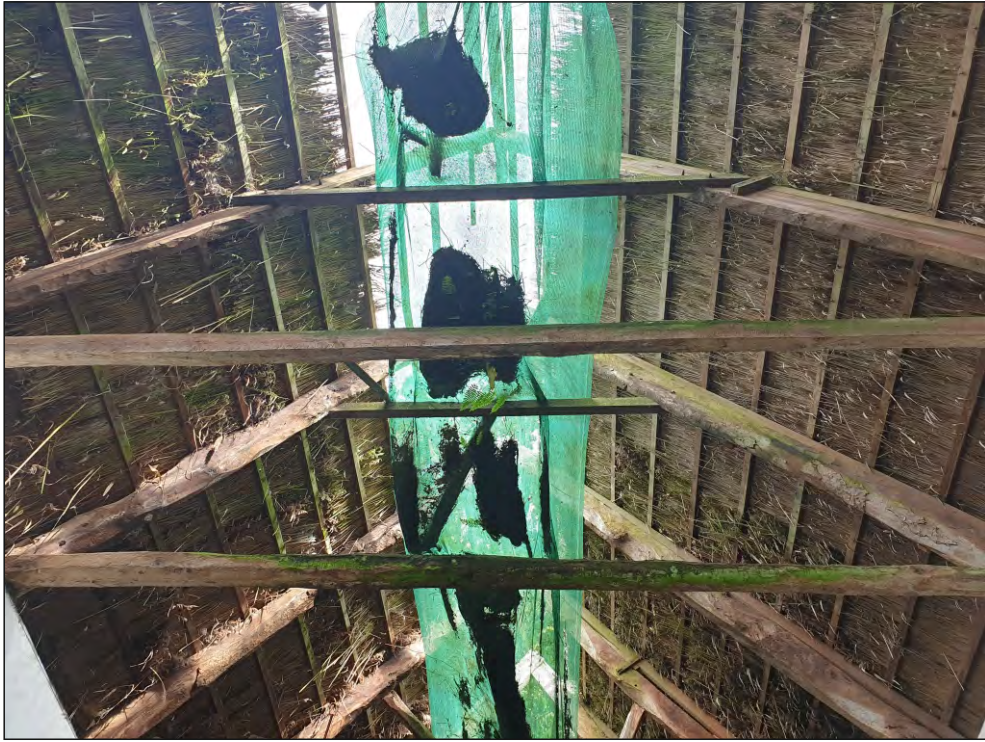
Pl. 17 General view of roof structure showing trusses with bolted modern collars and original pegged tie beams. Looking south.
