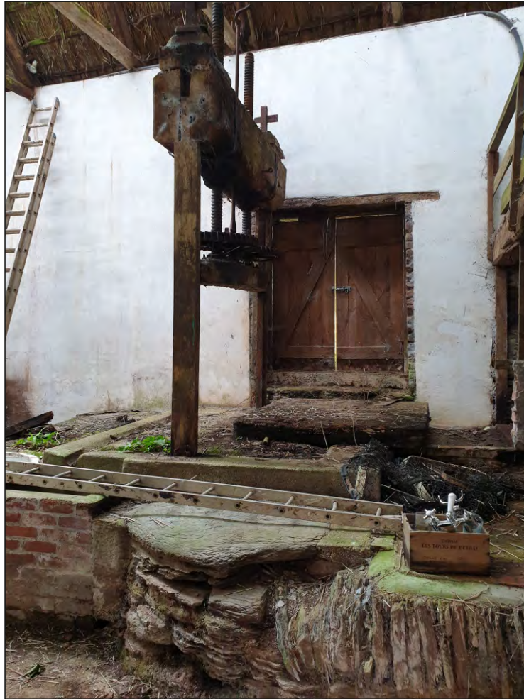
Fig. 9 General view of double door in west elevation with partly rebuilt stone platform in foreground. Looking southwest.
