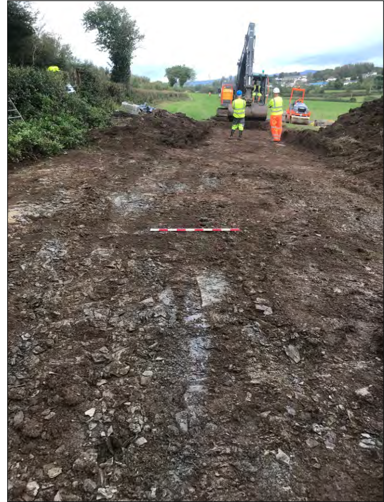
Pl. 2 General view of access road and new soakaway site excavations. 1m scale. Looking northwest.
