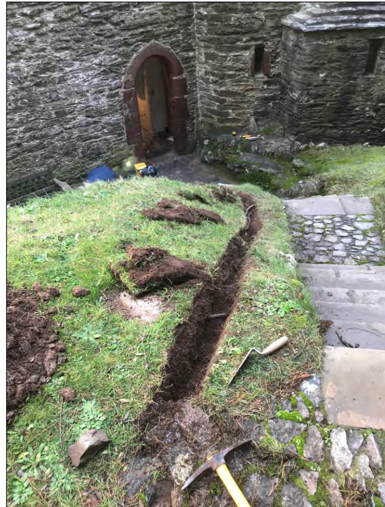
Pl. 2 General view of trenching towards Kingswear Castle showing depth of deposits. Looking southwest.
