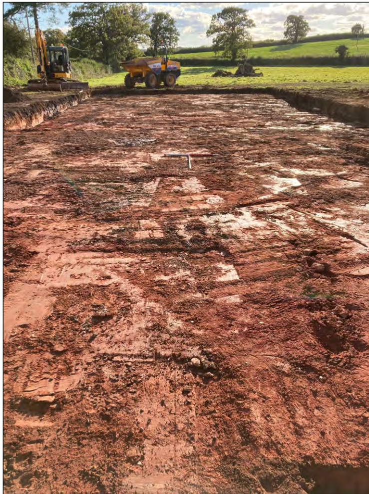
Pl. 3 General view of the soil strip for the access road and southern garage. Looking south.
