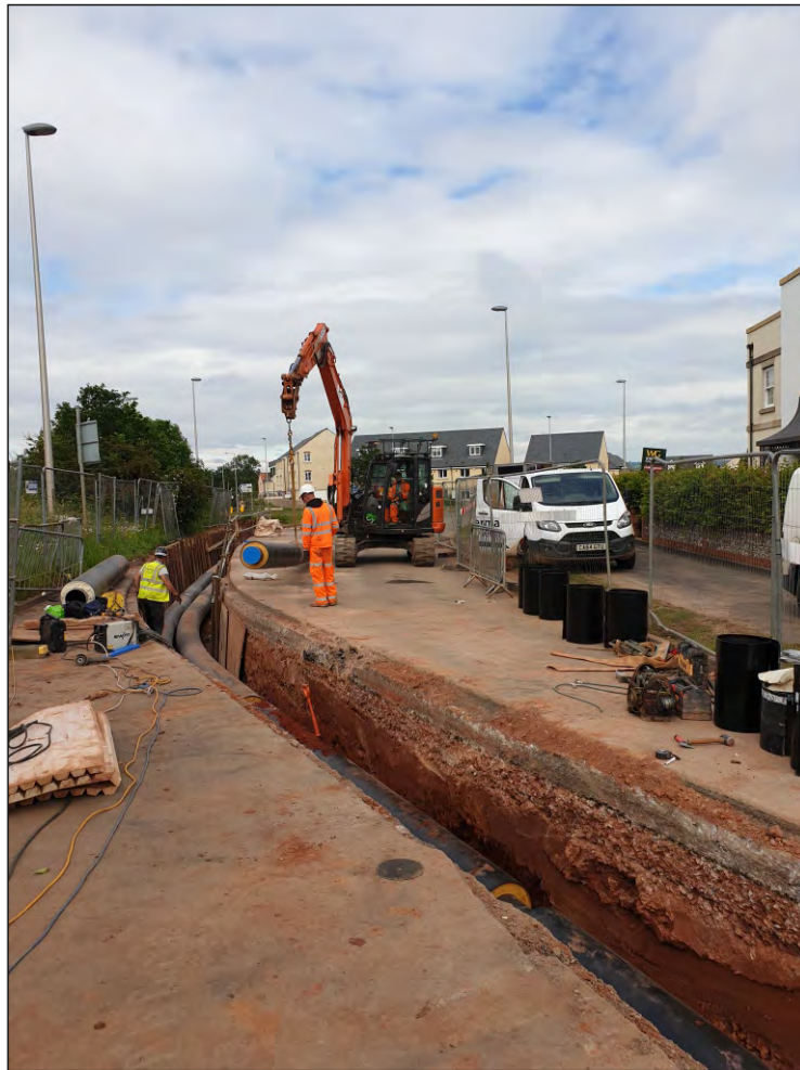
Pl. 7 General view of trenching route through B3174 London Road. 2m scale. Looking west.
