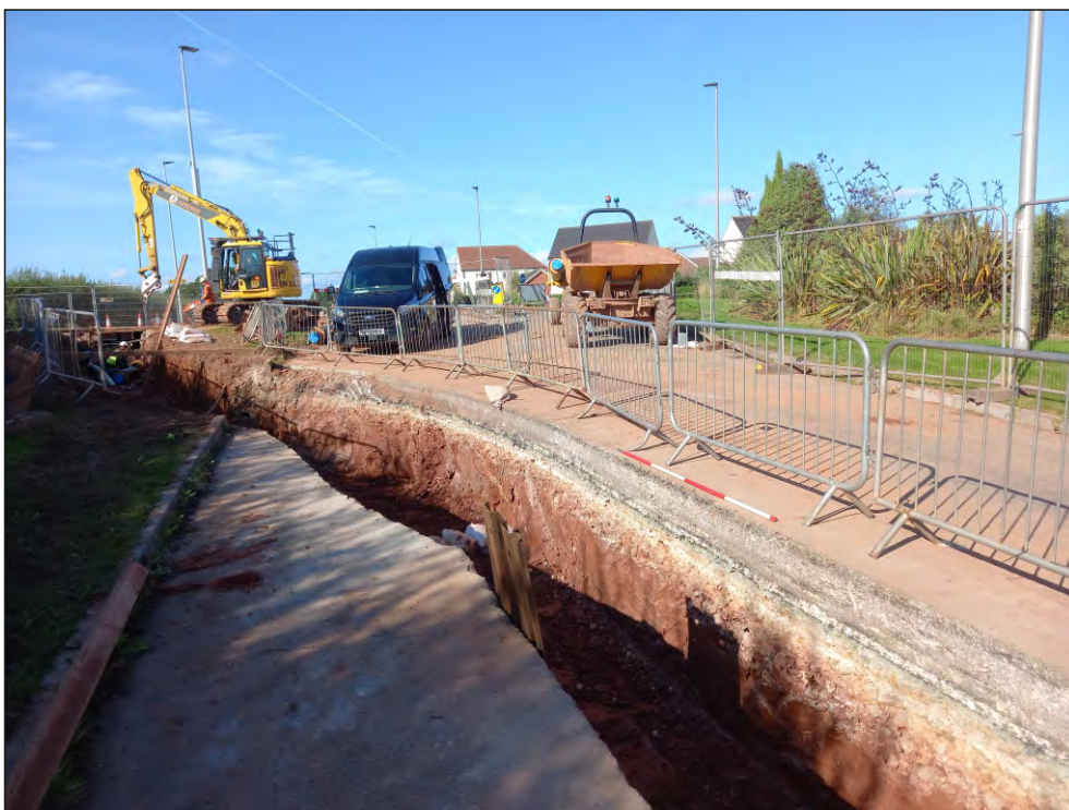
Pl. 10 General view of trenching route through B3174 London Road. 2m scale. Looking northwest.
