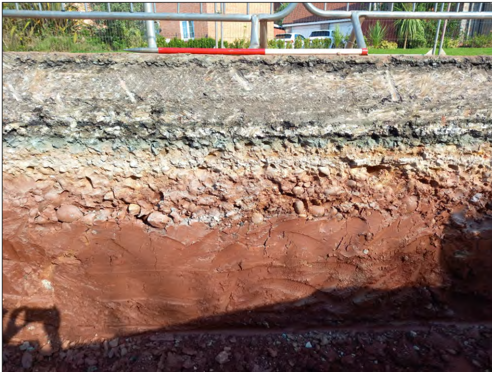
Pl. 12 Close-up showing typical deposit sequence of modern road make-up. 1m scale. Looking northwest.
