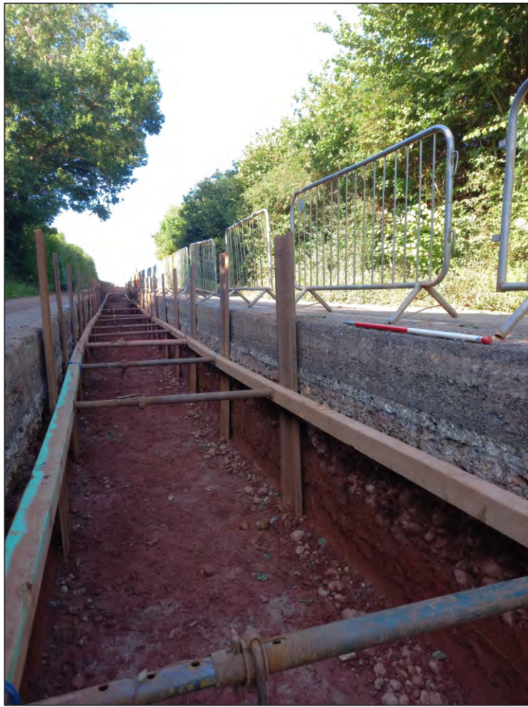
Pl. 13 General view of trenching route through B3174 London Road. 1m scale. Looking west.
