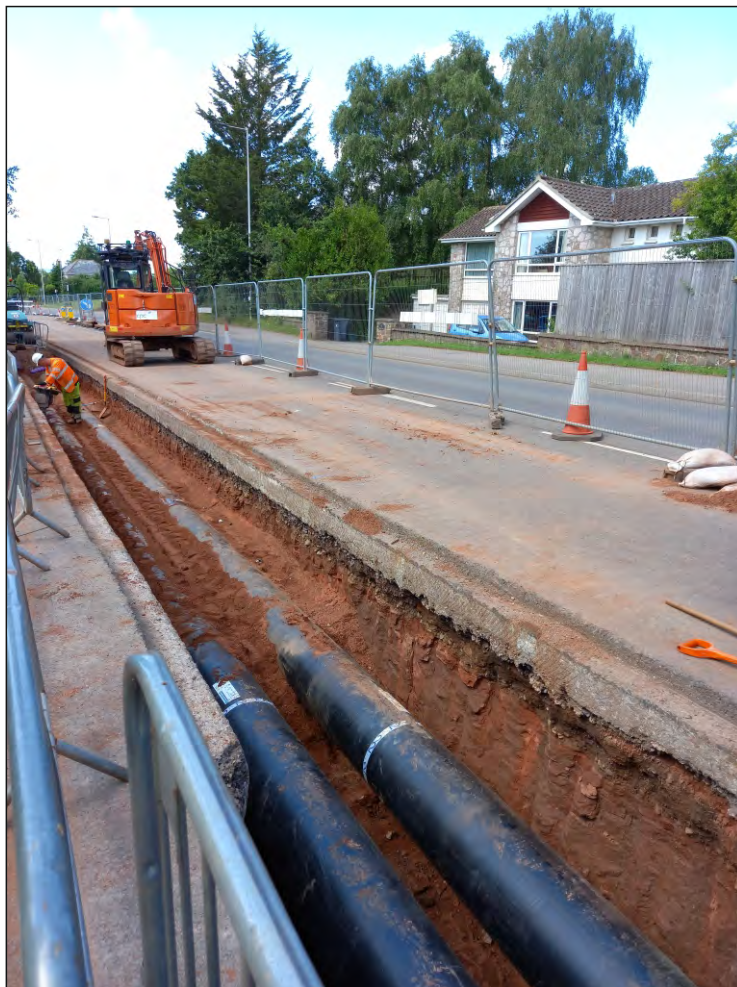
Pl. 5 General view of trenching route through B3174 London Road. 2m scale. Looking southwest.
