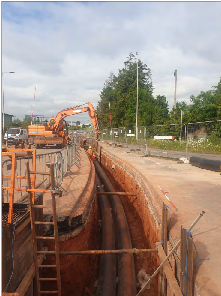
Pl. 1 General view of trenching route through B3174 London Road. 2m scale. Looking southwest.
