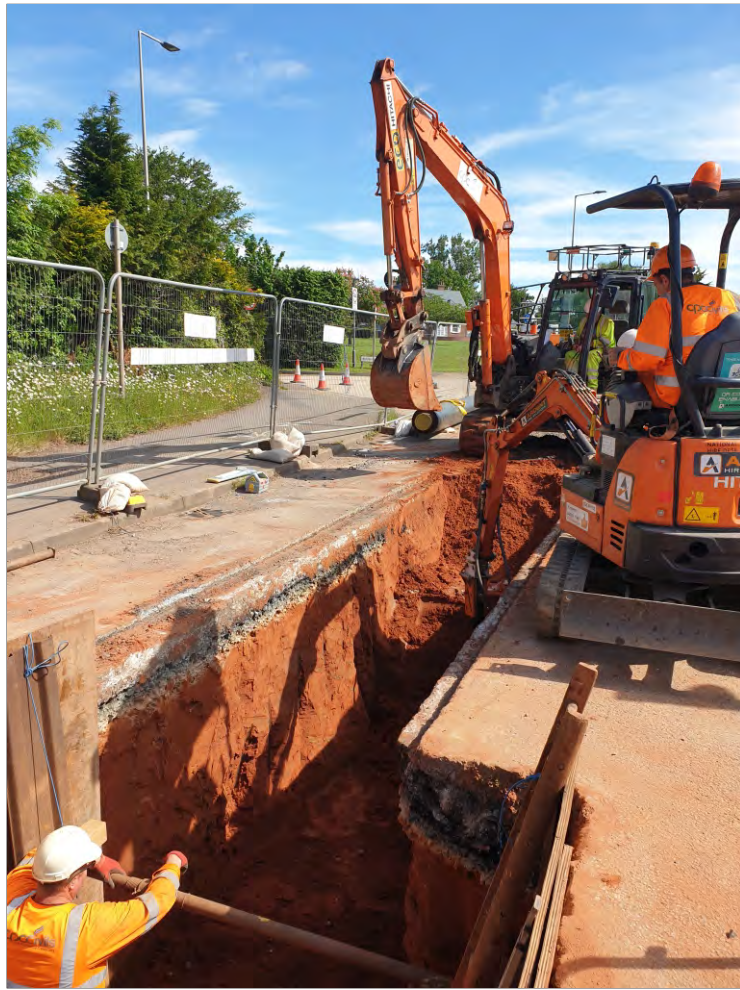
Pl. 3 General view of trenching route through B3174 London Road. 2m scale. Looking northeast.
