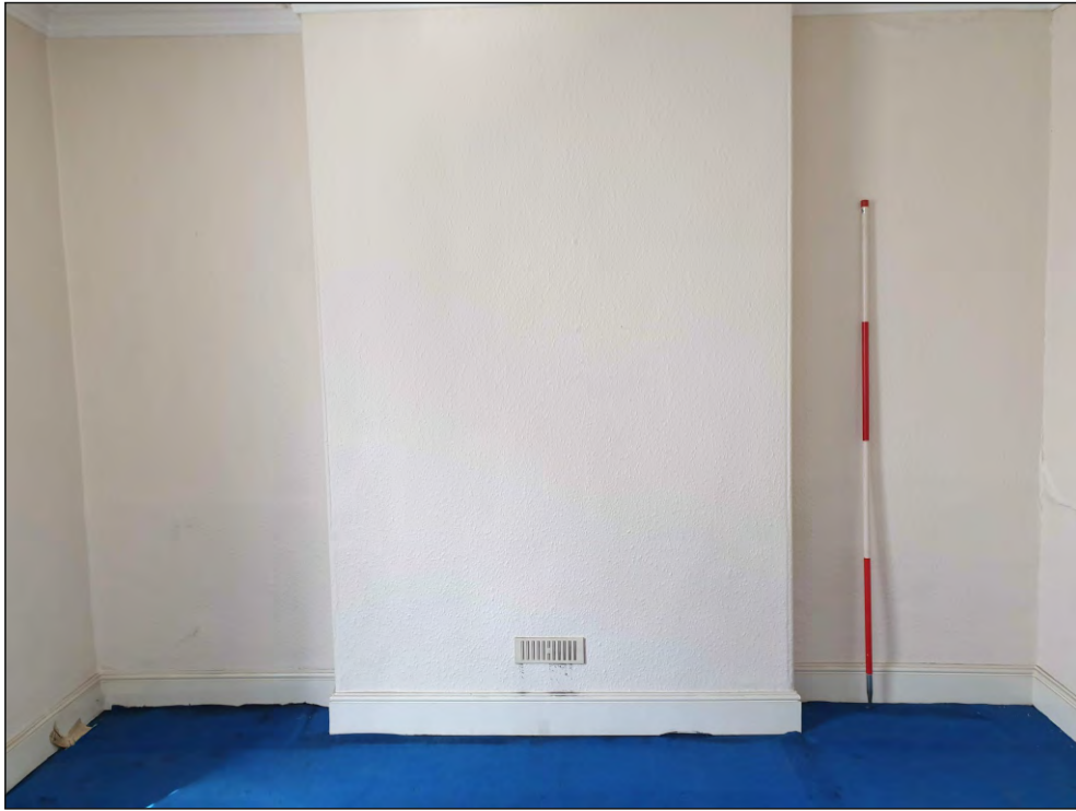
Pl. 21 General view of F03 showing position of former mid-19th century fireplace. 2m scale. Looking west.
