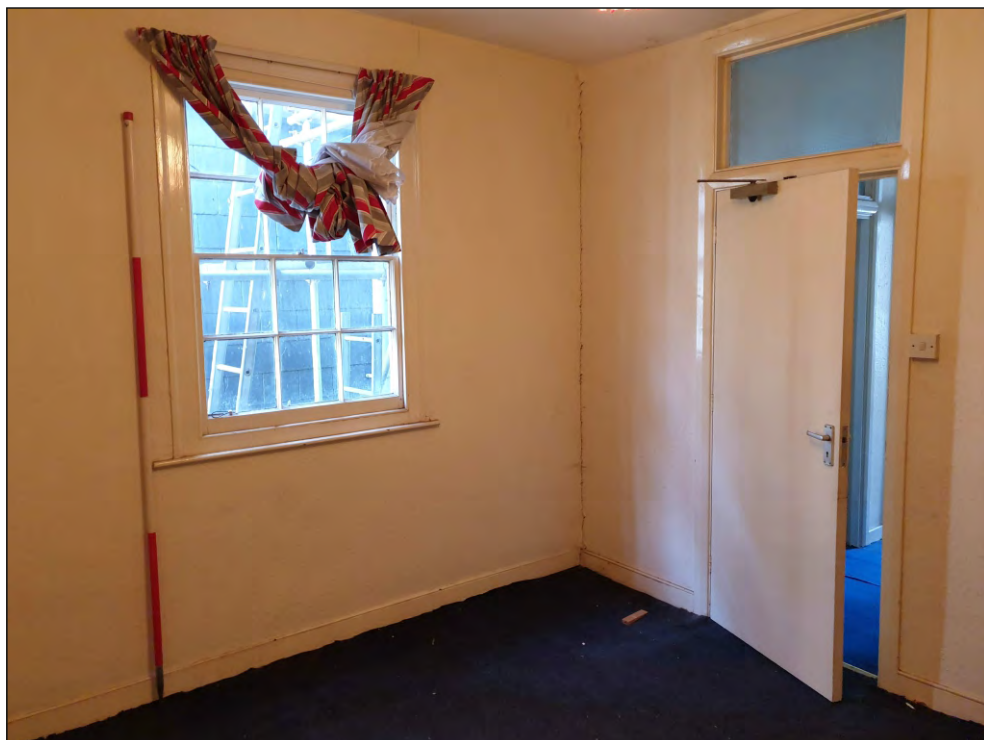
Pl. 30 General view of S04 showing original mid-19th century sash window in east elevation and modern doorway and door. 2m scale. Looking southeast.
