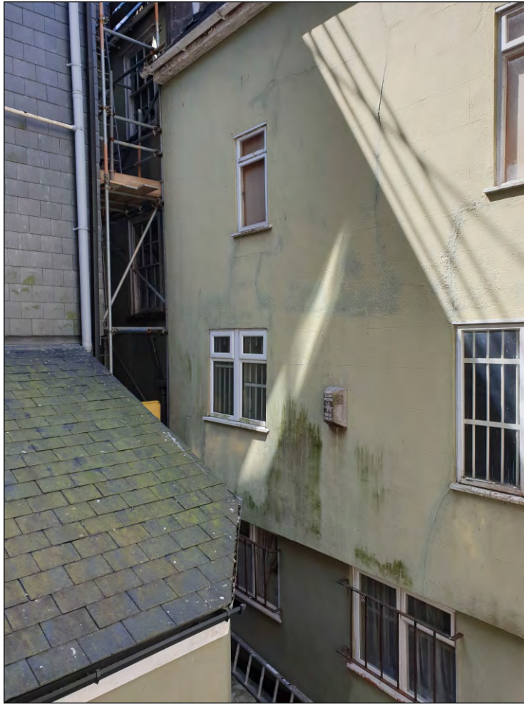
Pl. 41 General view of rear extension showing projecting upper storeys and modern windows. Looking southwest.
