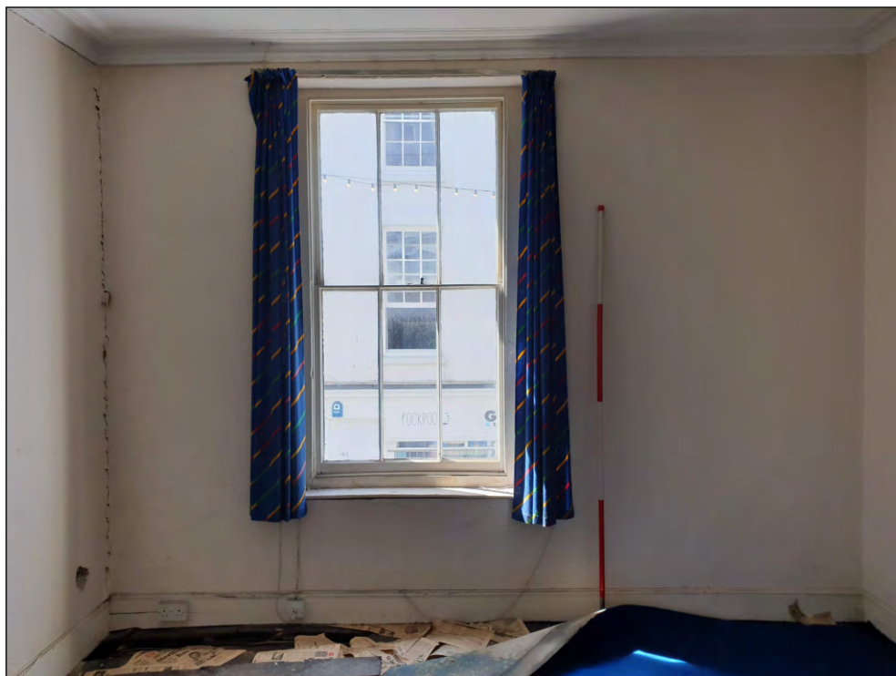
Pl. 20 General view of mid-19th century hornless sash window in F03. 2m scale. Looking south.
