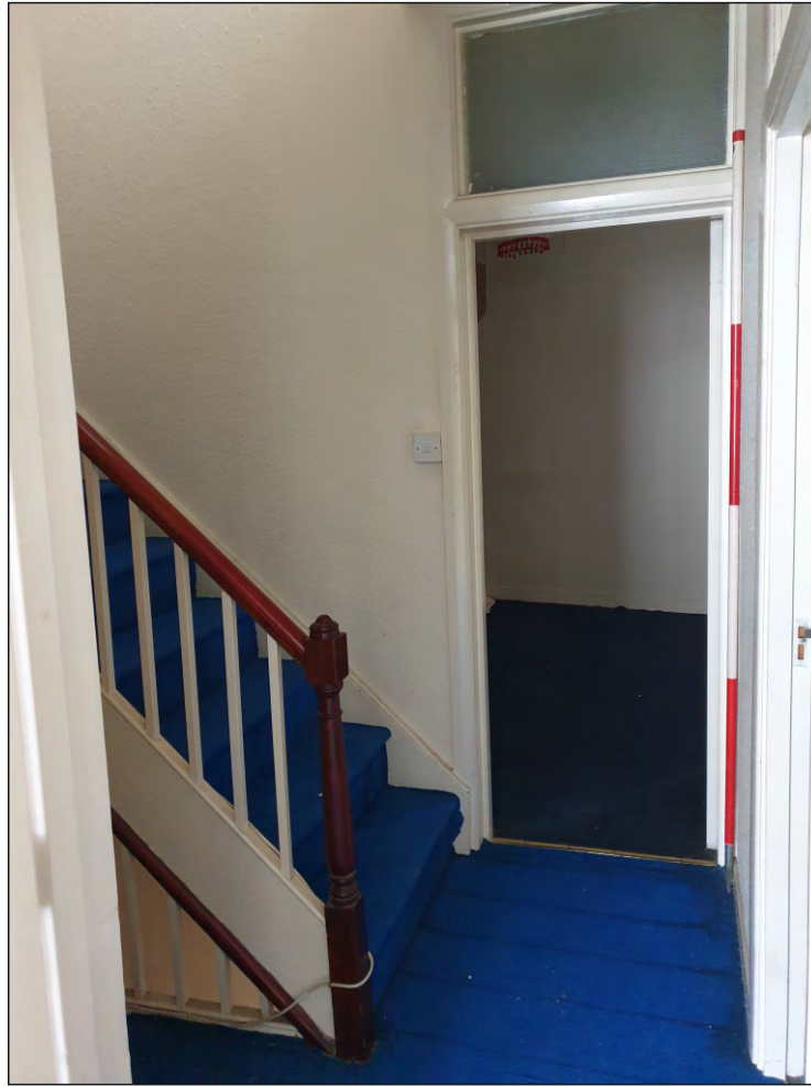
Pl. 29 General view of mid-19th century staircase and modern doorway into S04. 2m scale. Looking north.
