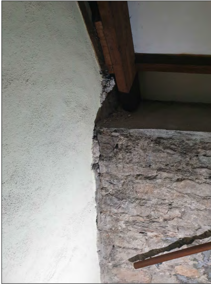
Pl. 49 Close-up showing a small gap between the north elevation of the central block and the rear range showing the former is a later rebuild. Looking southwest.
