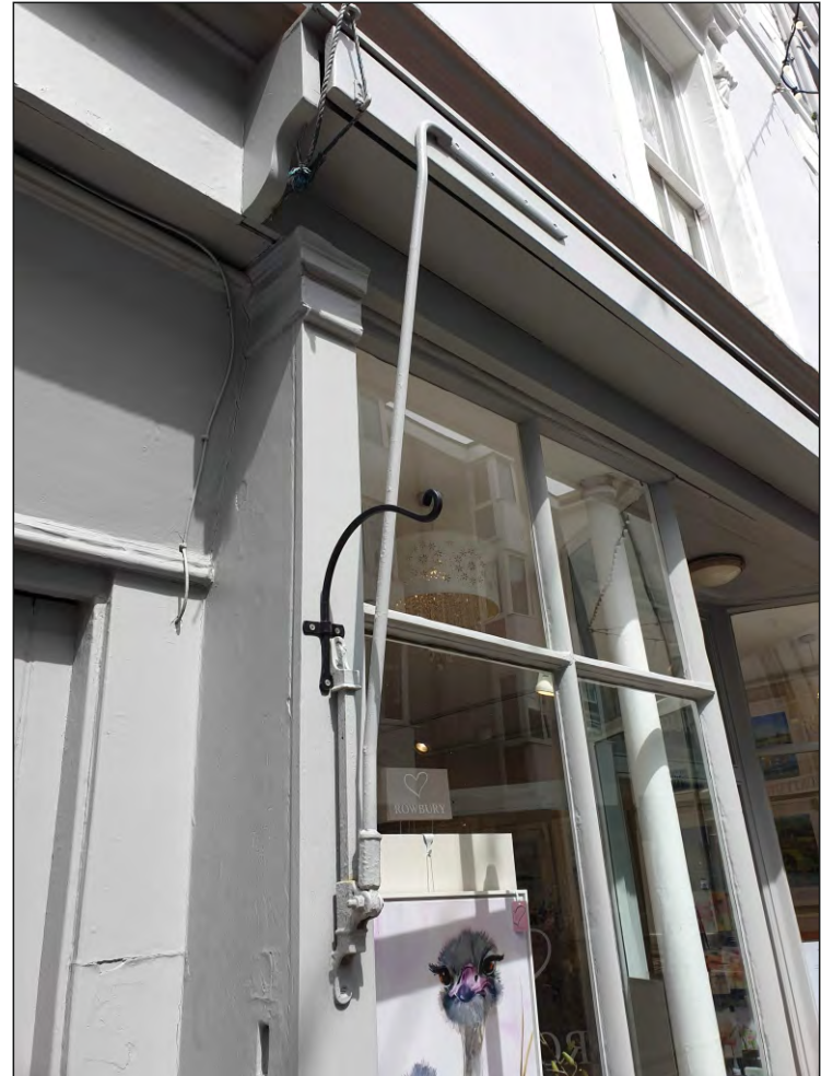
Pl. 4 Close-up of original awning mechanism and wooden container at No. 26. Looking northeast.
