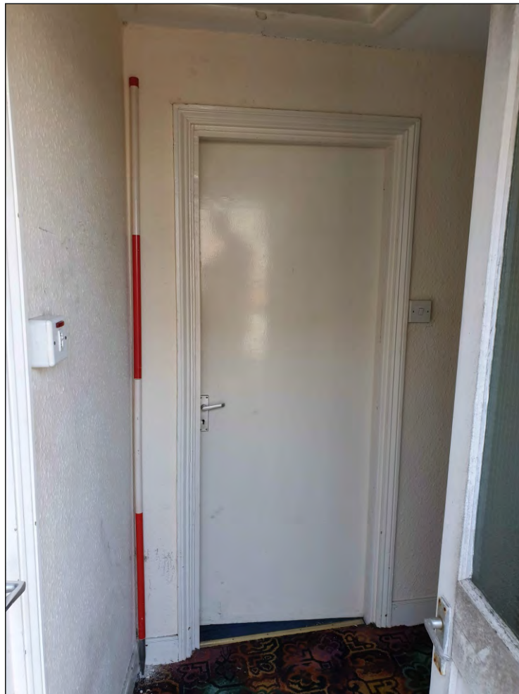
Pl. 34 General view of original mid-19th century doorframe and modern door into T02. 2m scale. Looking south.
