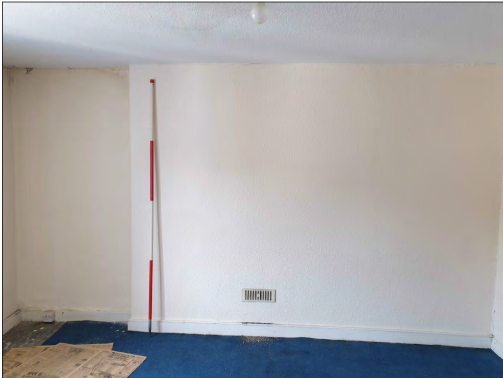
Pl. 36 General view of T02 showing position of former mid-19th century fireplace. 2m scale. Looking west.
