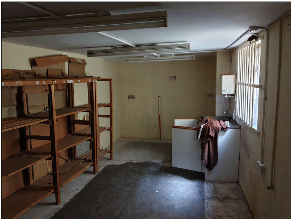
Pl. 42 General view of G04 showing modern partition at the rear and modern windows in the east elevation. 1m scale. Looking north.
