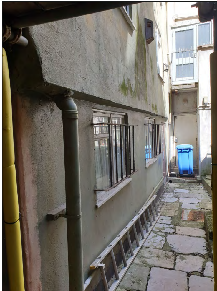
Pl. 40 General view of rear extension showing projecting upper storeys and modern ground floor windows. Looking northwest.
