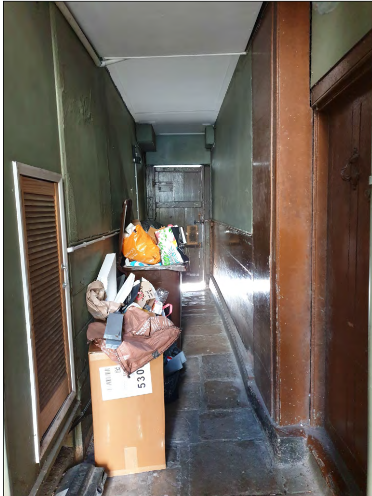
Pl. 13 General view of passage showing set-back mid-19th century doorway to original entrance hall and staircase in G01. Looking south.
