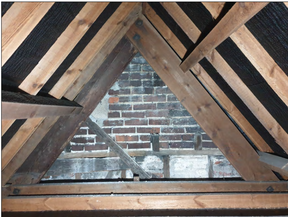
Pl. 50 General view of the roof structure showing original 17th century truss (left), 19th century replacement truss and purlins (right) and modern common rafters. In the background is the north elevation of the mid-19th century infill. Looking south.
