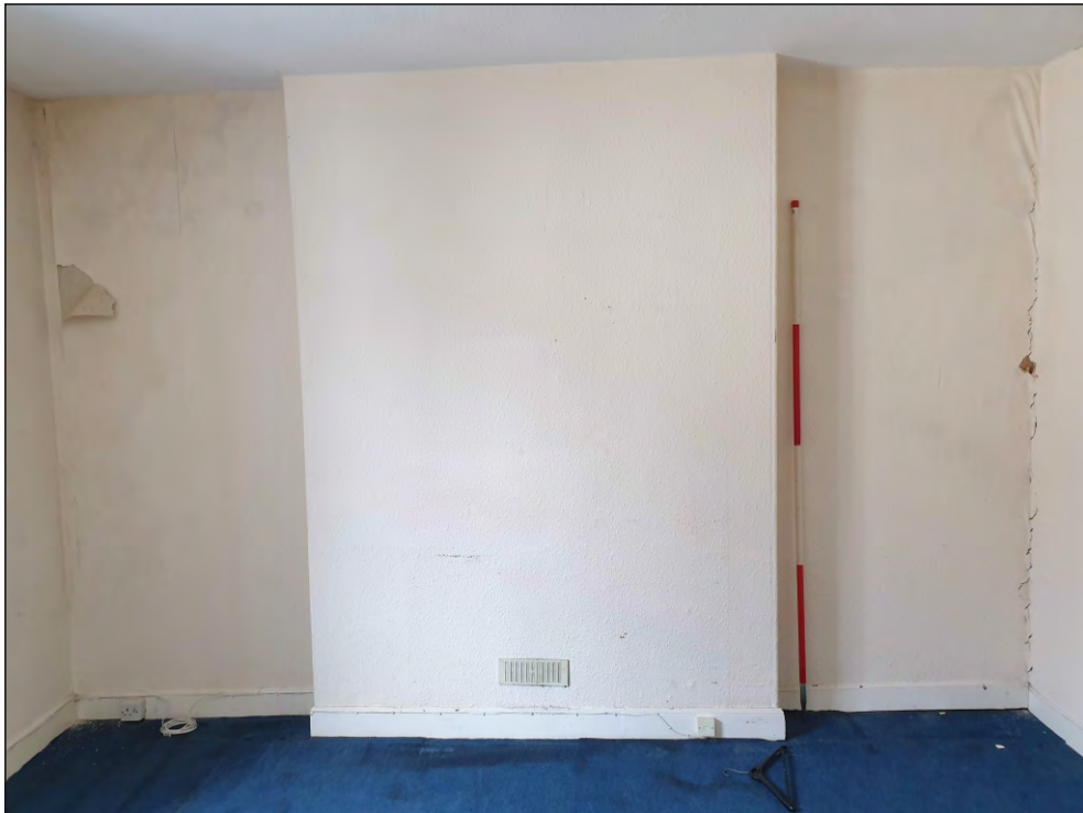
Pl. 28 General view of S03 showing position of former mid-19th century fireplace. 2m scale. Looking west.
