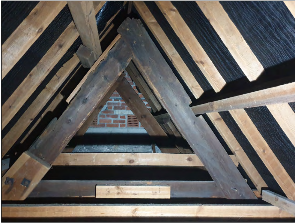
Pl. 51 General view of the roof structure showing original 17th century trusses (foreground) and 19th century replacement trusses (background) and purlins, and modern common rafters. Looking north.
