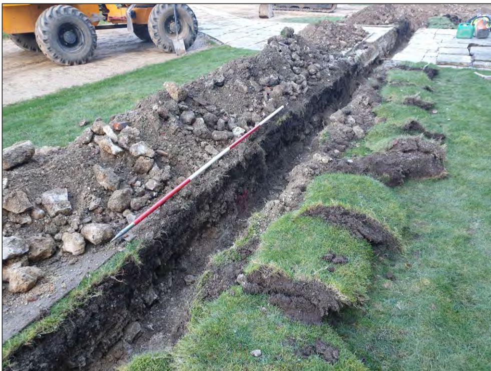
Pl. 8 General view of the trench showing extensive 18th century disturbance (104) underneath the landscaping. 2m scale. Looking northeast.
