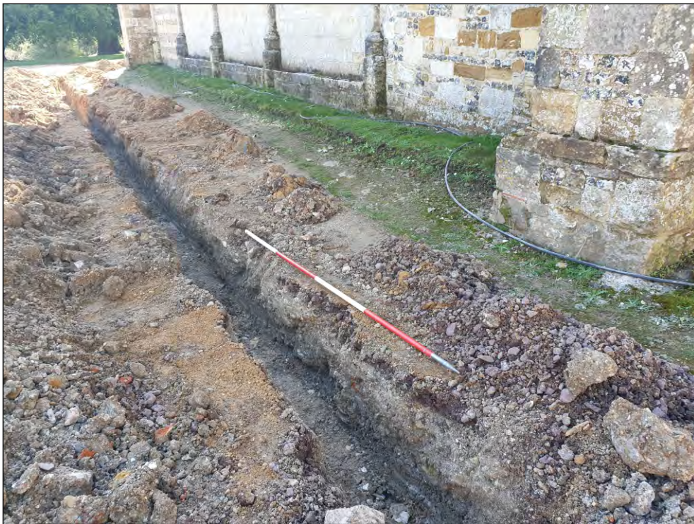
Pl. 6 General view of electric trench across east end of abbey church showing backfill of 2017 trench. 2m scale. Looking southwest.
