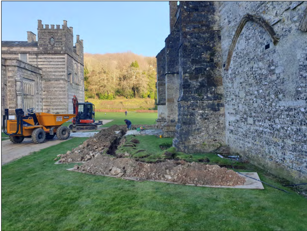
Pl. 7 General view of electric trench on north side of abbey church with the position of the former sacristy in the foreground. 2m scale. Looking east.
