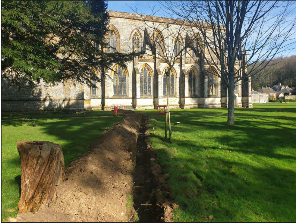
Pl. 1 General view of water trench to south of abbey. 2m scale. Looking northeast.
