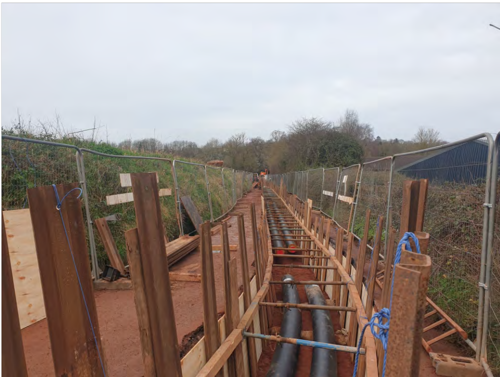
Pl. 4 General view of trenching route leading to Pinhoe Target Shooting Club. Looking northwest.
