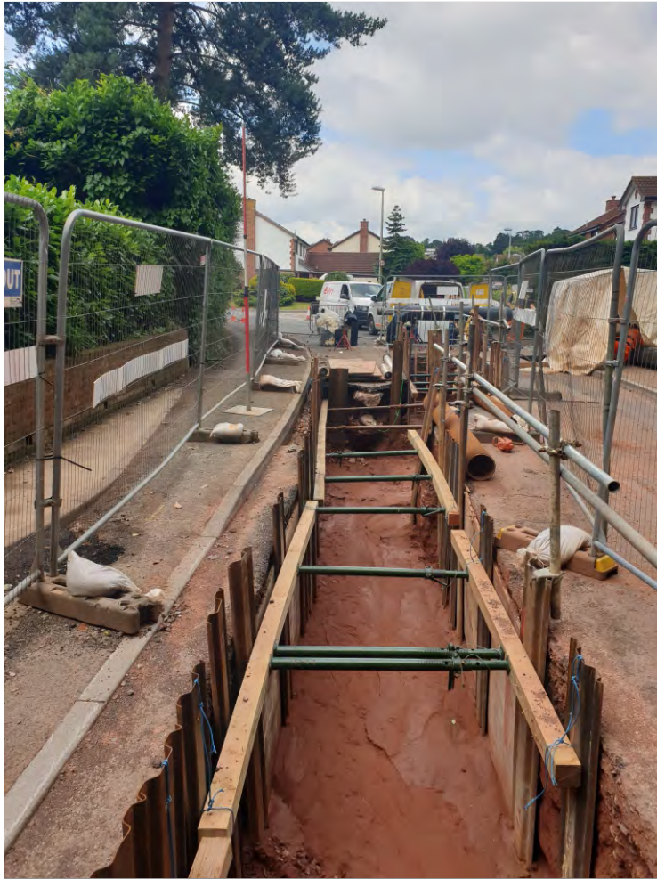
Pl. 1 General view of trenching route at north end of Langaton Lane. Looking northwest.
