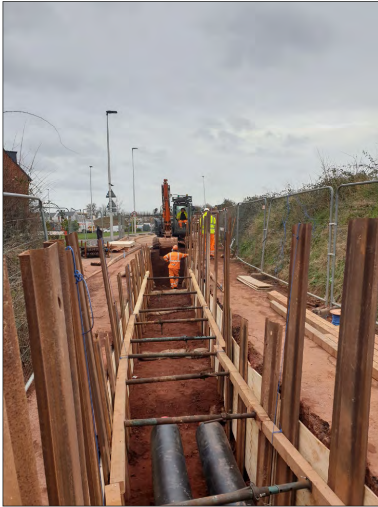
Pl. 9 General view of trenching route at south end of Langaton Lane looking towards Tithebarn Way. Looking south.
