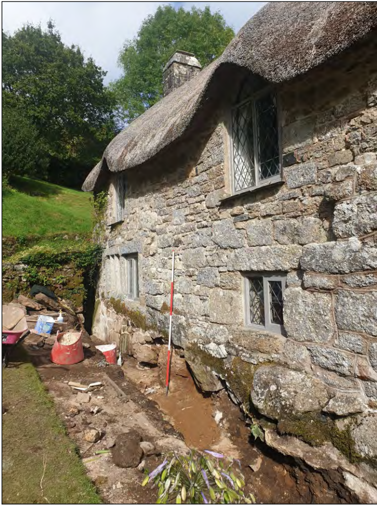
Pl. 1 General view of west elevation showing base of wall above gowan and granite bedrock protrusions. 2m scale. Looking northeast.
