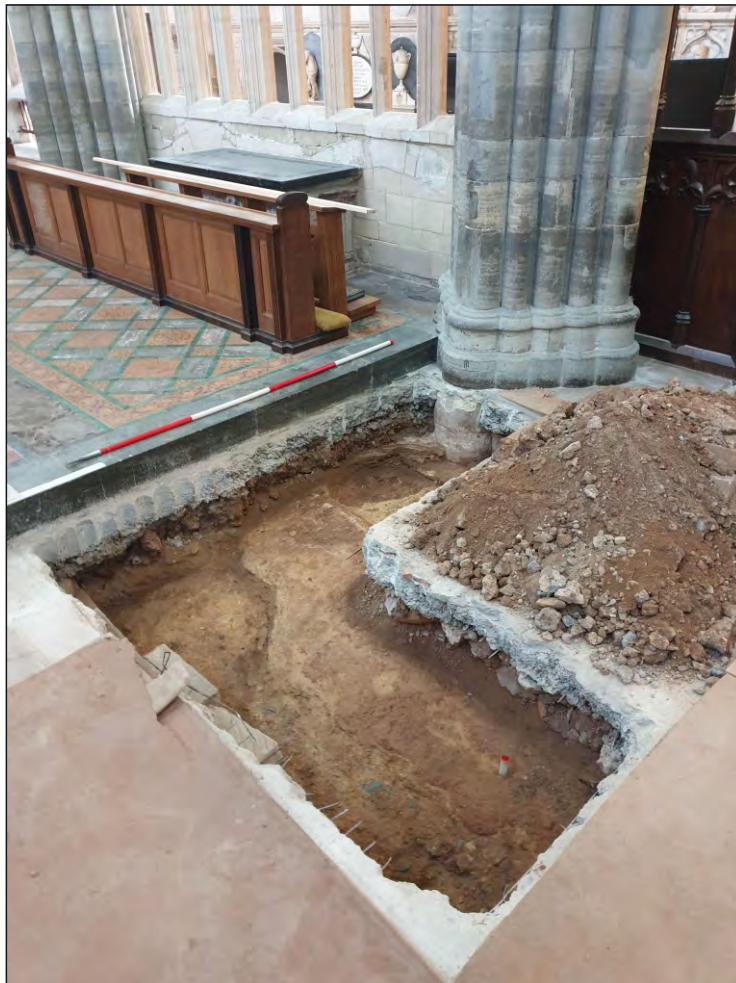
Pl. 18 General view of Trench 8 showing stone working and mortar deposits associated with the reconstruction of the east end in the late 13th and early 14th century truncated by the late 19th and 1960s flooring. 2m scale. Looking southeast.
