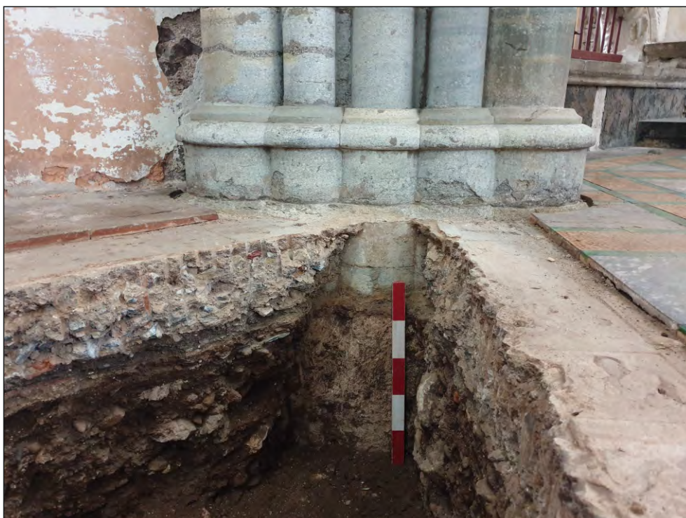
Pl. 12 Close-up of pier (419) and pier foundation (421) showing the original level of the 18th and late 13th century floors. 0.5m scale. Looking northeast.
