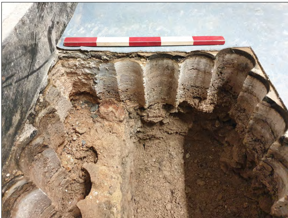
Pl. 26 Section through Trench 9 showing depth of concrete (900), south wall of vestry (903) and infill above vaulting (902). 0.5m scale. Looking west.
