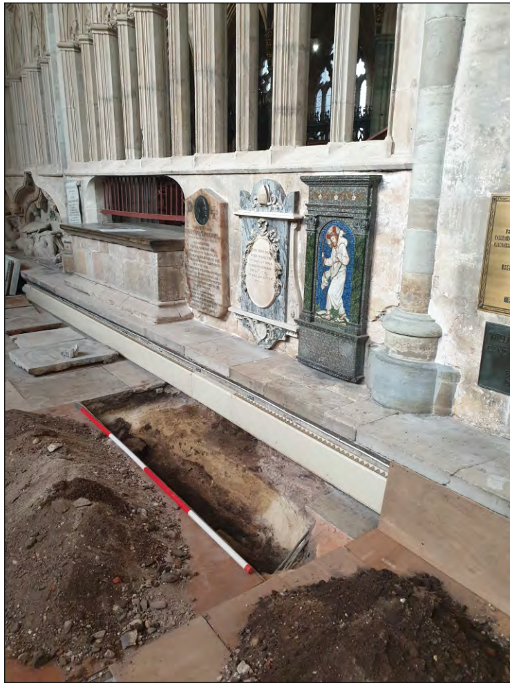
Pl. 9 General view of Trench 3 showing the stepped foundation for the choir screen and bench (303). 2m scale, Looking northwest.
