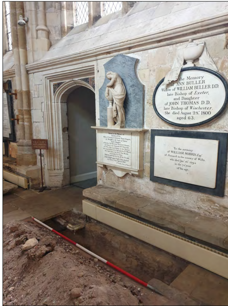
Pl. 7 General view of Trench 2 showing the stepped foundation for the south wall and bench (204). 2m scale, Looking southeast.
