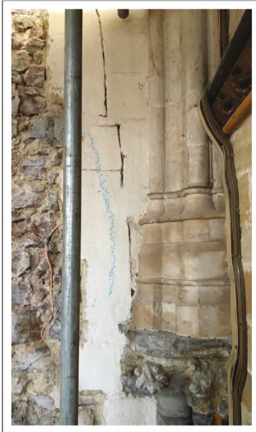
Fig. 4d. Chapter House, west wall: building break above 13th-century capital on north side providing evidence for early vault ( photo: J. Allan ).
