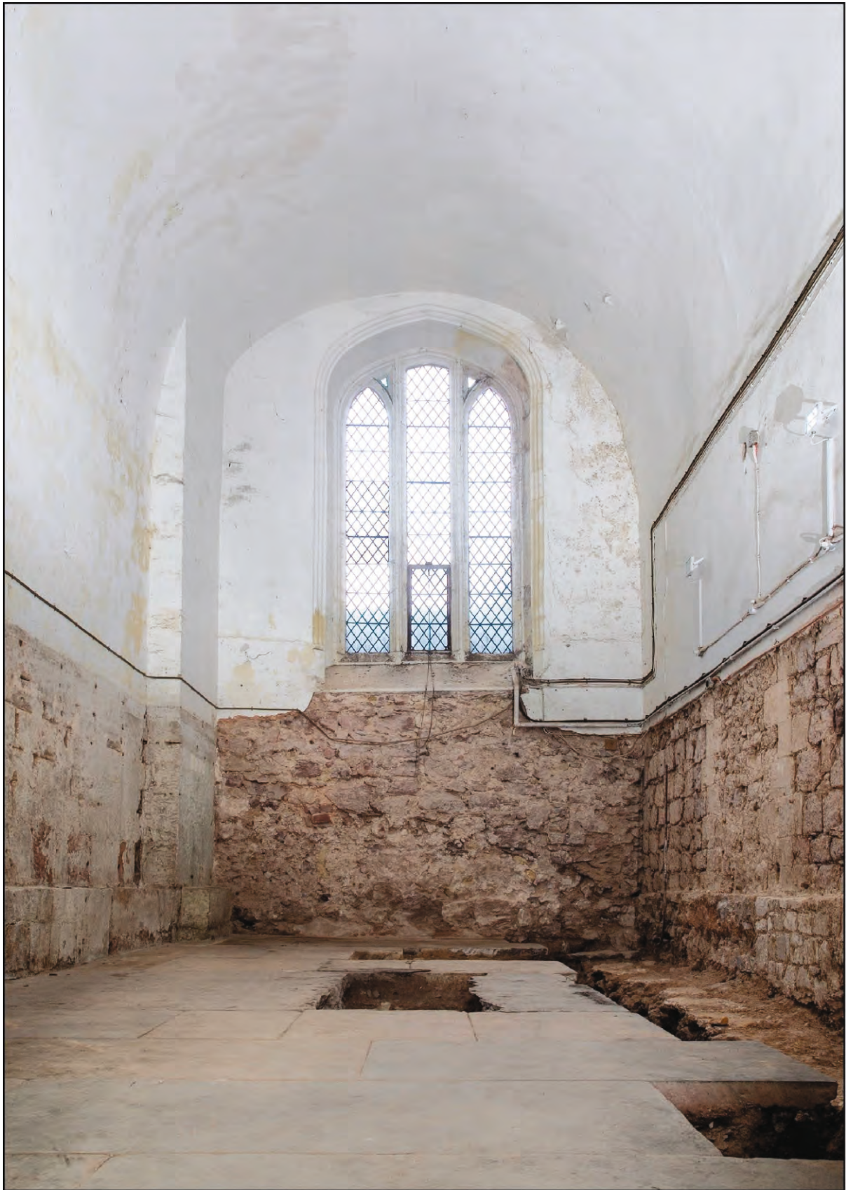
Fig. 11. The Chapel of the Holy Spirit looking east after excavation and removal of cement from the walls, 25 March 2021 ( photo: Gary Young ).
