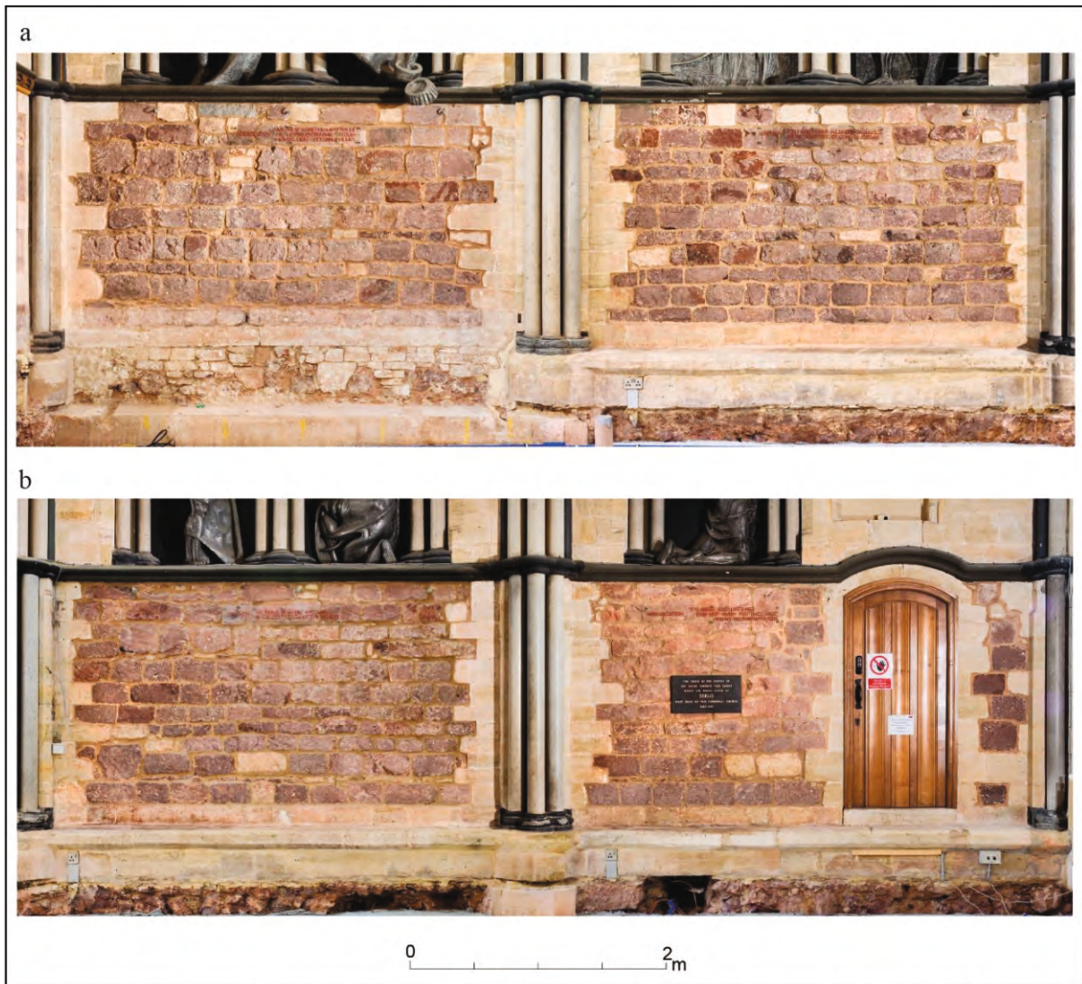
Fig. 6a-b. The Chapter House: internal face of the south wall, March 2021. (a) Bays 1 and 2. (b) Bays 3 and 4. The plain masonry was replastered subsequently (photos: Gary Young).
