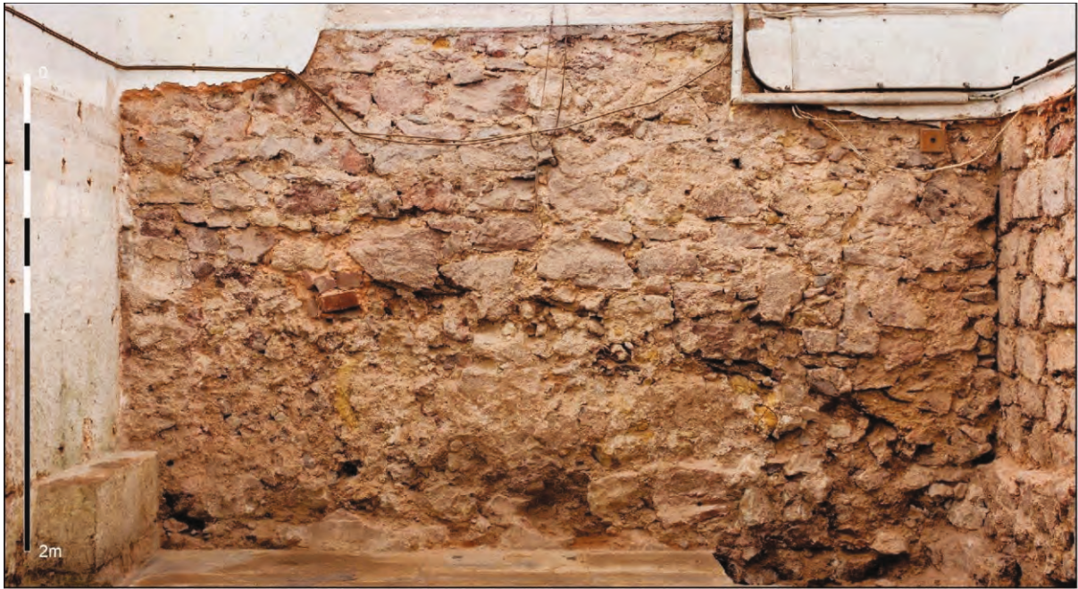
Fig. 15. The Chapel of the Holy Spirit: rectified photographic record of the east wall after removal of cement render ( photo: Gary Young, 8 Feb. 2021 ).
