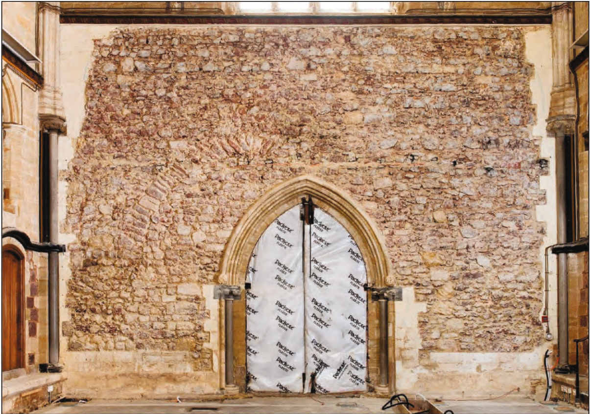
Fig. 4a. The Chapter House: internal face of the west wall after removal of modern render, 1 April 2021 (photo: Gary Young).
