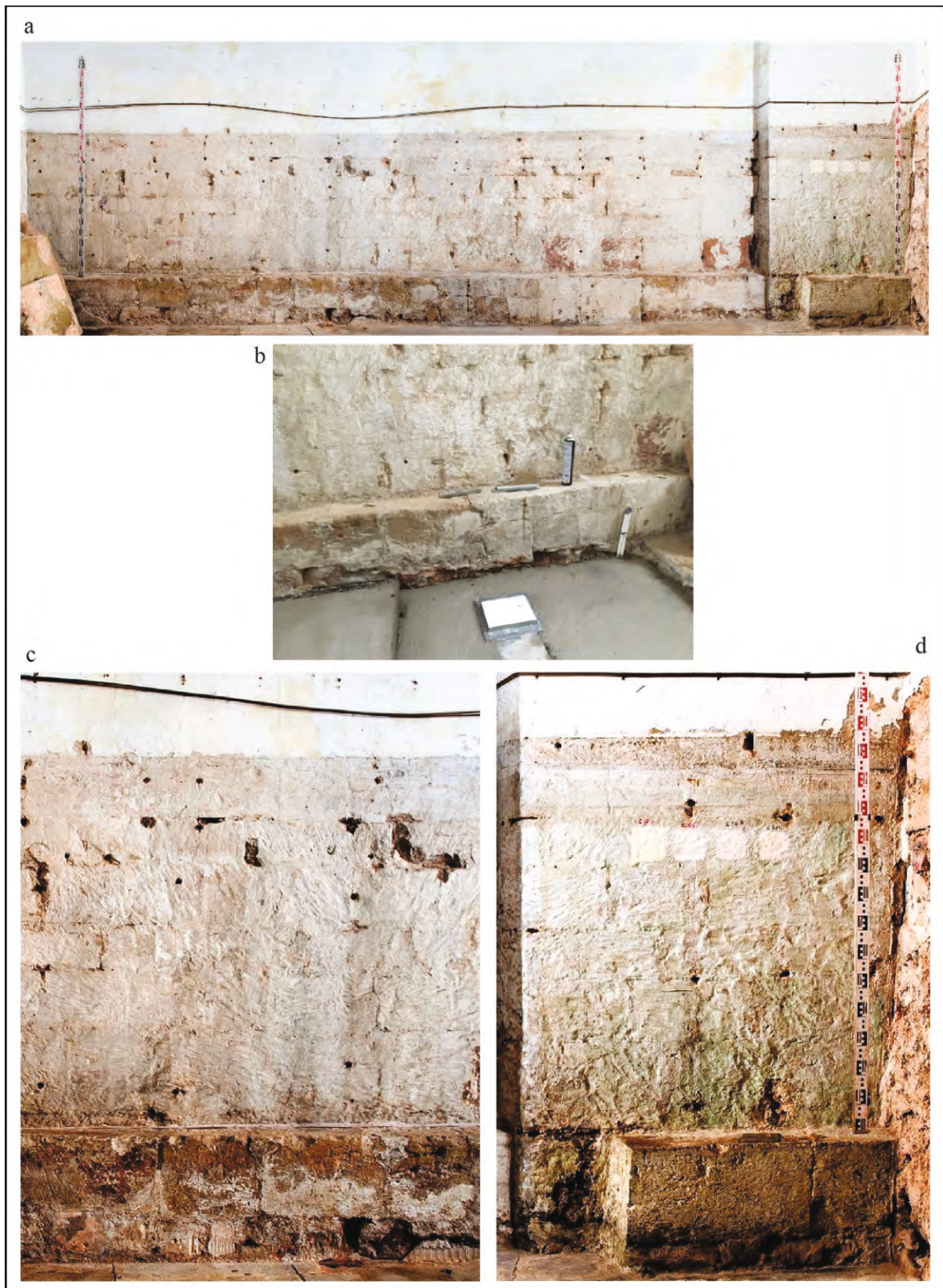
Fig. 12. The Chapel of the Holy Spirit: the north wall (external face of the south tower). (a) Photogrammetric record. (b) Footing exposed by lifting of paving slabs. (c–d) Details showing rough dressing, indicating that the face has been cut back (photo: a, c–d Gary Young, 8 Feb. 2021; (b) J. Allan, 9 March 2021 ).
