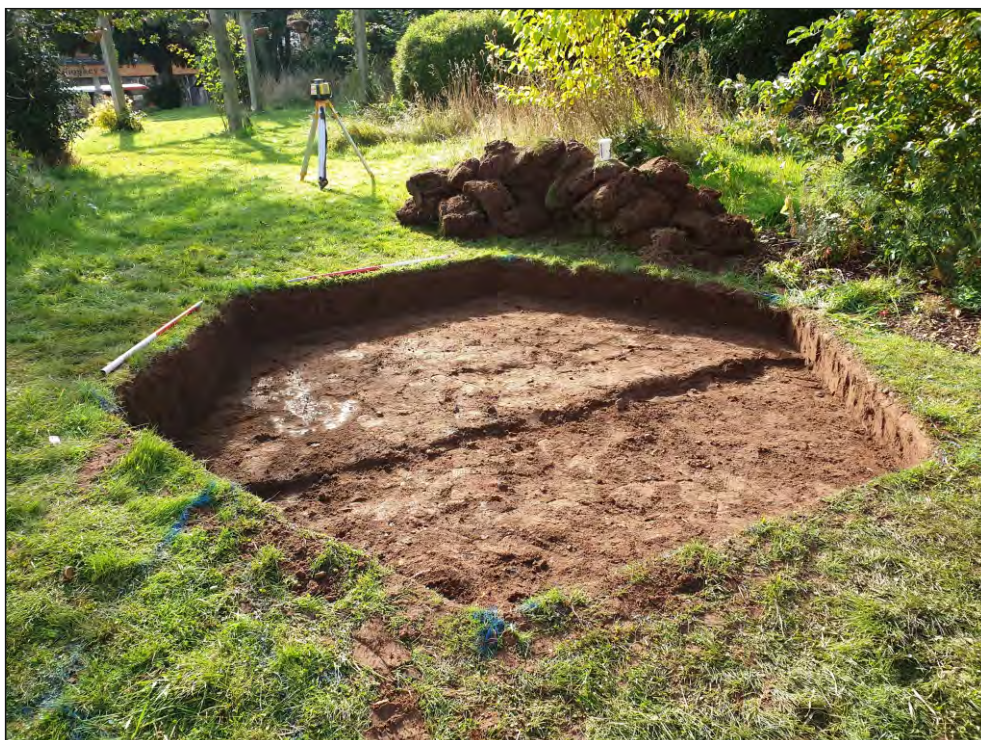
Pl. 2 General view of the new bell tower base. 1m scales. Looking southwest.
