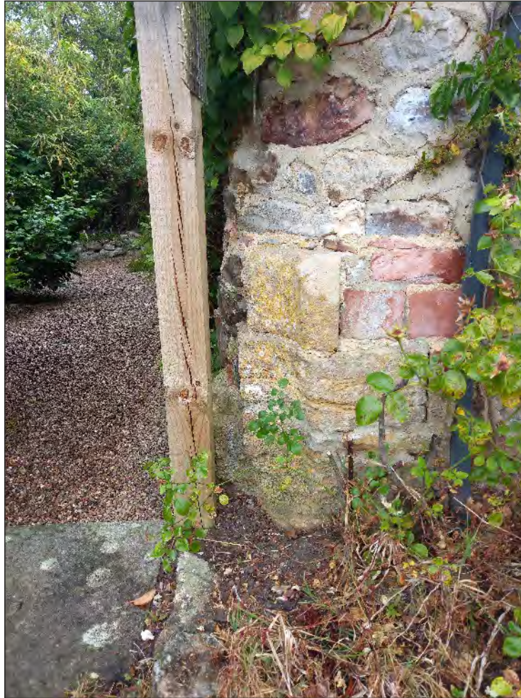
Pl. 3 Close-up of the surviving southern jamb of the former monastic gatehouse incorporated within Abbey Cottage. Looking east.
