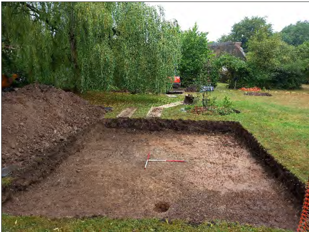
Pl. 6 General view of the new drainage field (Trench 2) showing depth of deposit sequence above natural subsoil. 1m scales. Looking northwest.
