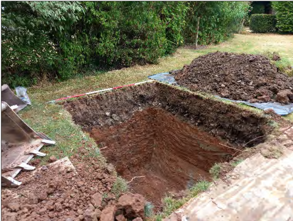
Pl. 4 General view of the new septic tank location (Trench 1). 2m scale. Looking northwest.
