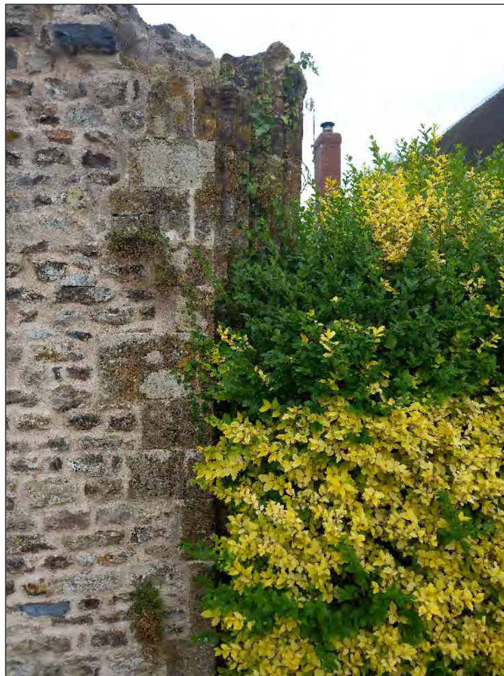
Pl. 2 Close up of the northern jamb of the former monastic gatehouse. Looking east.
