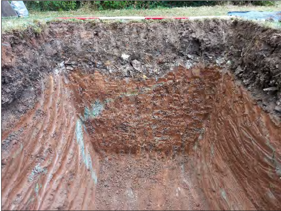
Pl. 5 Section through the new septic tank trench showing deposit sequence. 2m scale. Looking west.
