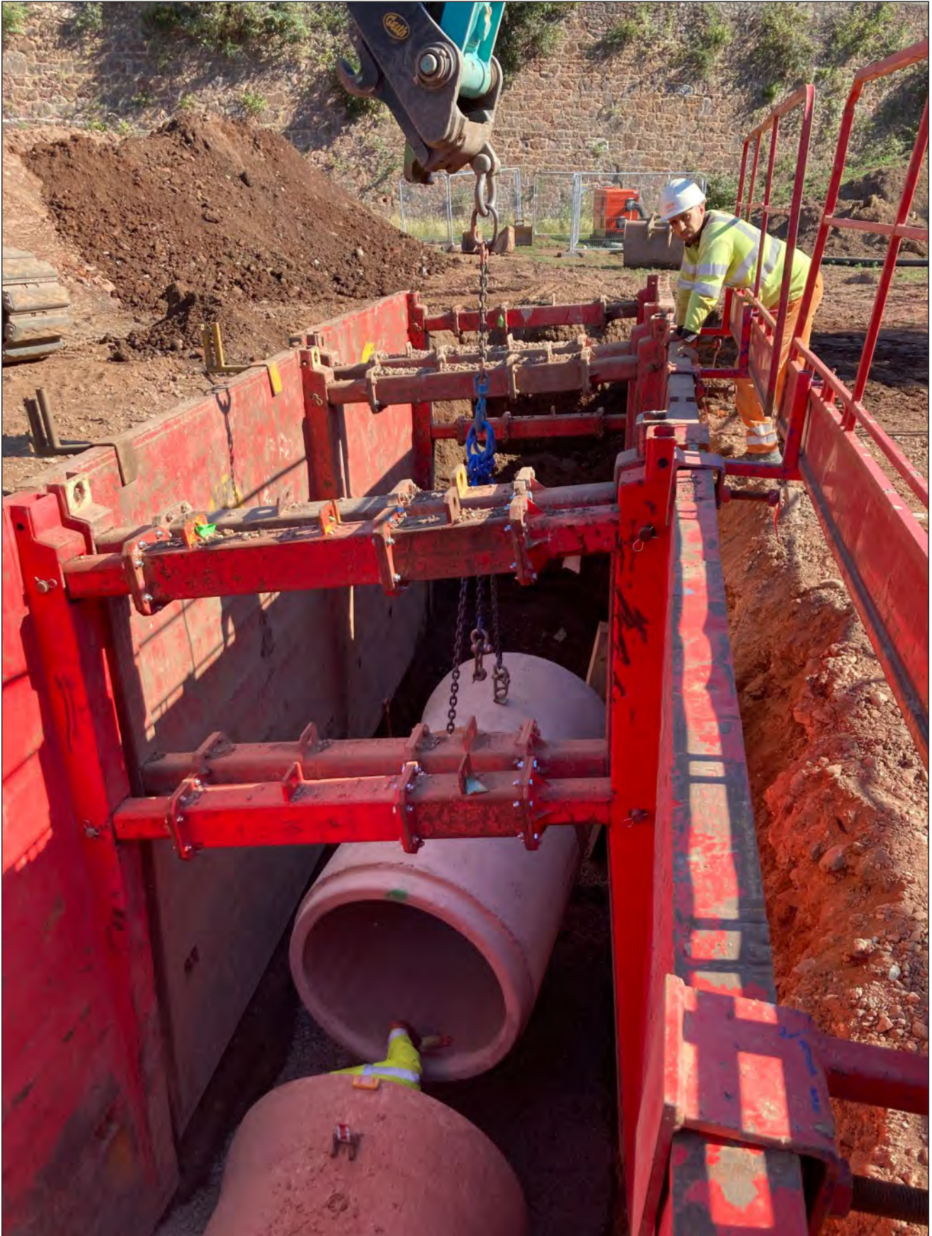
Pl. 4 General view of the pipe trench looking towards the Magdalene Street Viaduct. Looking northeast.
