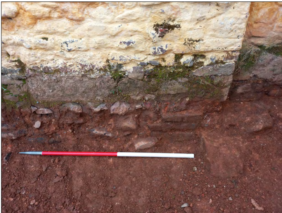
Pl. 12 Close-up showing remains of the original late 15th-early 16th century foundations (far right) and the later c.1800 rebuilding and refacing (left and centre) of the former interior elevation of the west range. 1m scale. Looking west.
