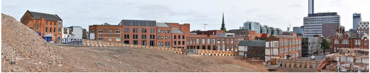
Harper's Hill site (south of Northwood Street); panoramic view looking south-east following demolition of majority of buildings showing significant drop away of ground level from Northwood Street (left) to Newhall Street / Graham Street (right); photographed 21.09.2021.
