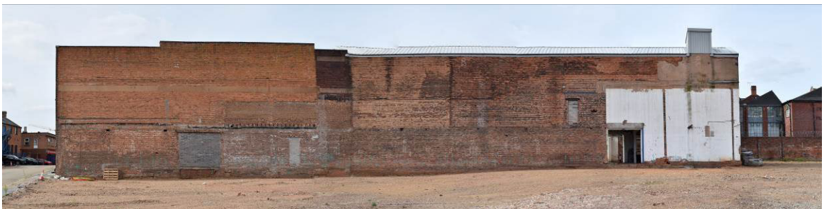
Eastern flanking wall of Building 7a/b, as observed following demolition of adjacent ranges (20.09.21); note horizontal change in brickwork at first-floor level to central section of range (7b), assumed related to early layout (see cross-section above).
