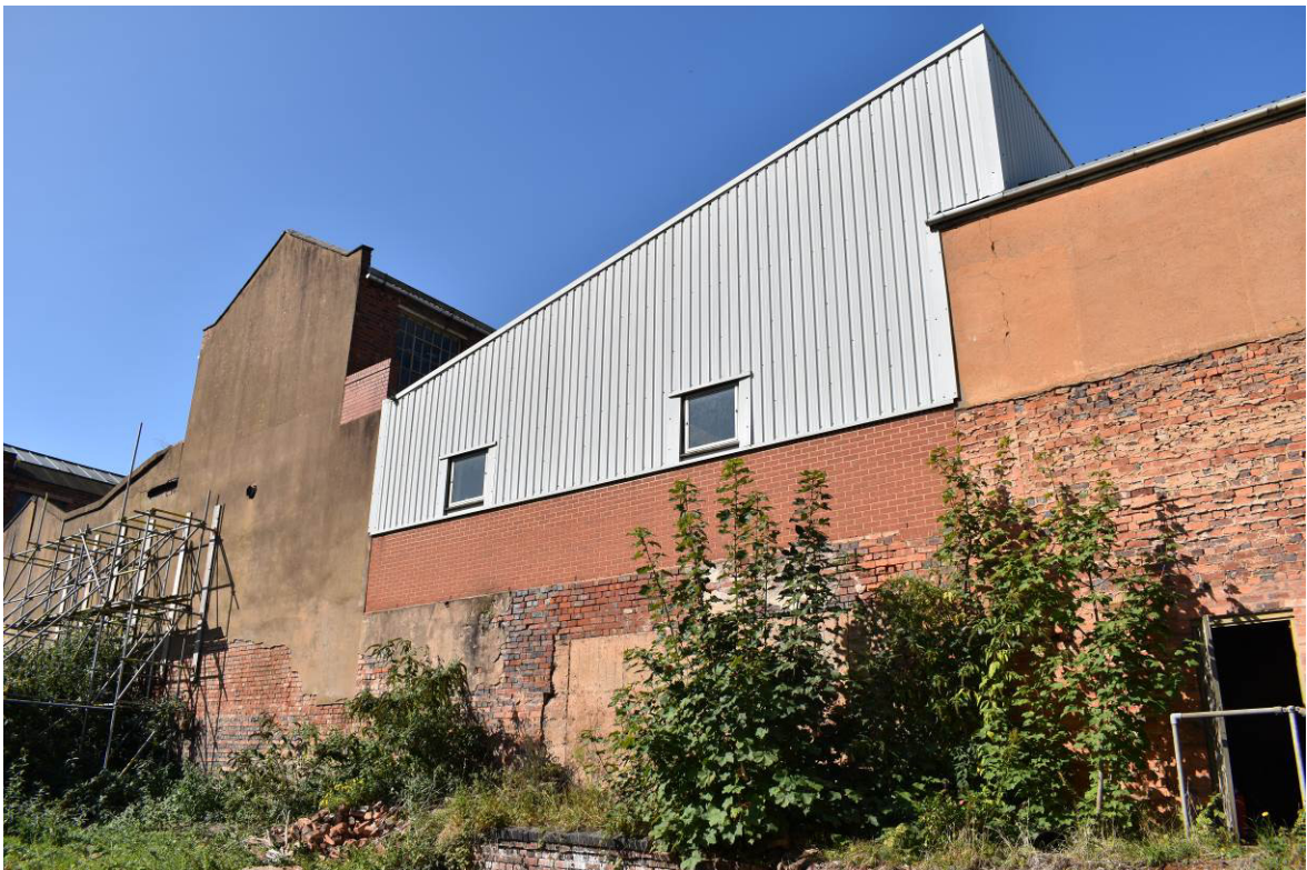
Plate 249: Building 12b; south elevation to yard adjacent to Bldg. 15 (incorporating early fabric at ground level).
