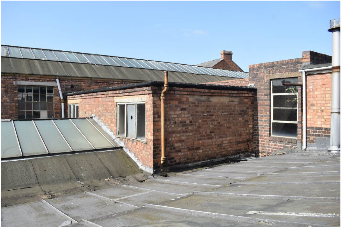
Plate 315: Building 13e; first floor level as seen from first floor of Bldg. 13a, looking north-west (Stair F to right).
