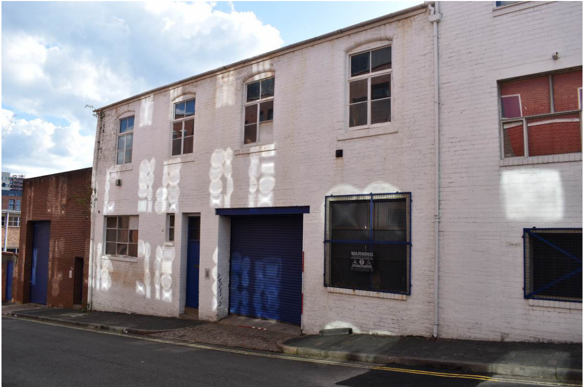
Plate 155: Building 10b (No. 11 James Street); east elevation to James Street. (NB. window to right of roller door set within original doorway opening – transverse entry bay indicated here on Piggott-Smith, 1855).
