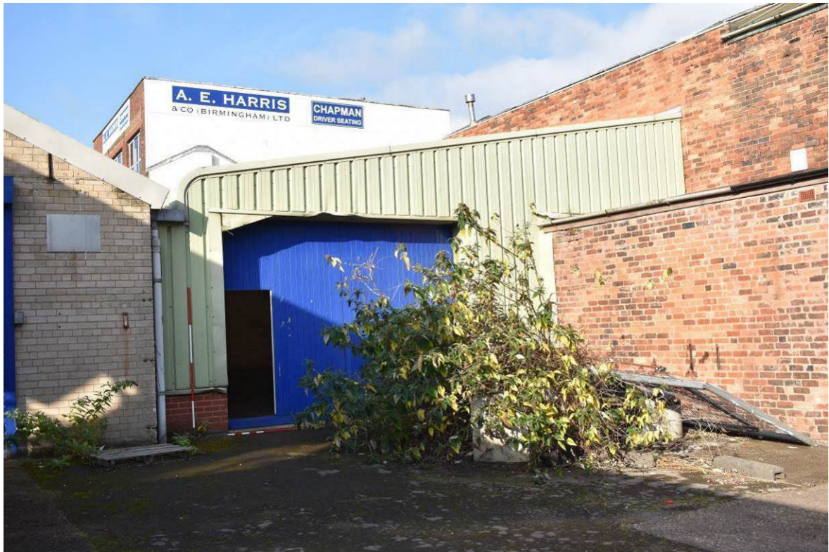
Plate 221: Building 11d; east elevation to yard (Bldg. 11c to left; 11a/e to right and Bldg.12 to background).
