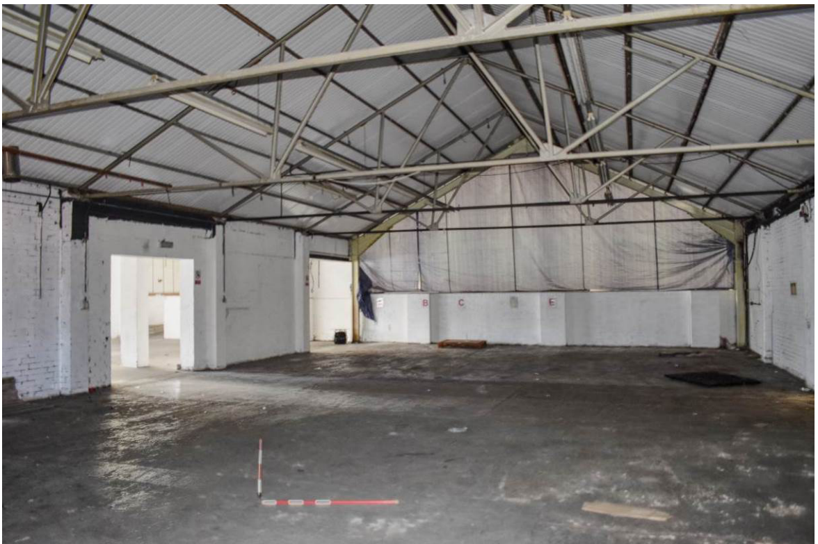
Plate 216: Building 11c: interior looking west; doors to left open to range 11b.
