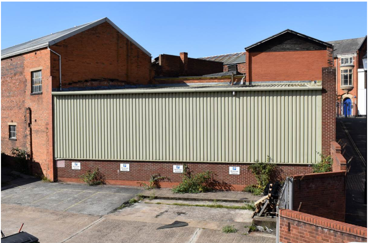
Plate 183: Building 10d, south elevation as seen from Bldg. 15a, looking north (James Street to right) with rebuilt gable end of truncated range 10b beyond. NB. scar of curved roof to east elevation of 11b (left).
