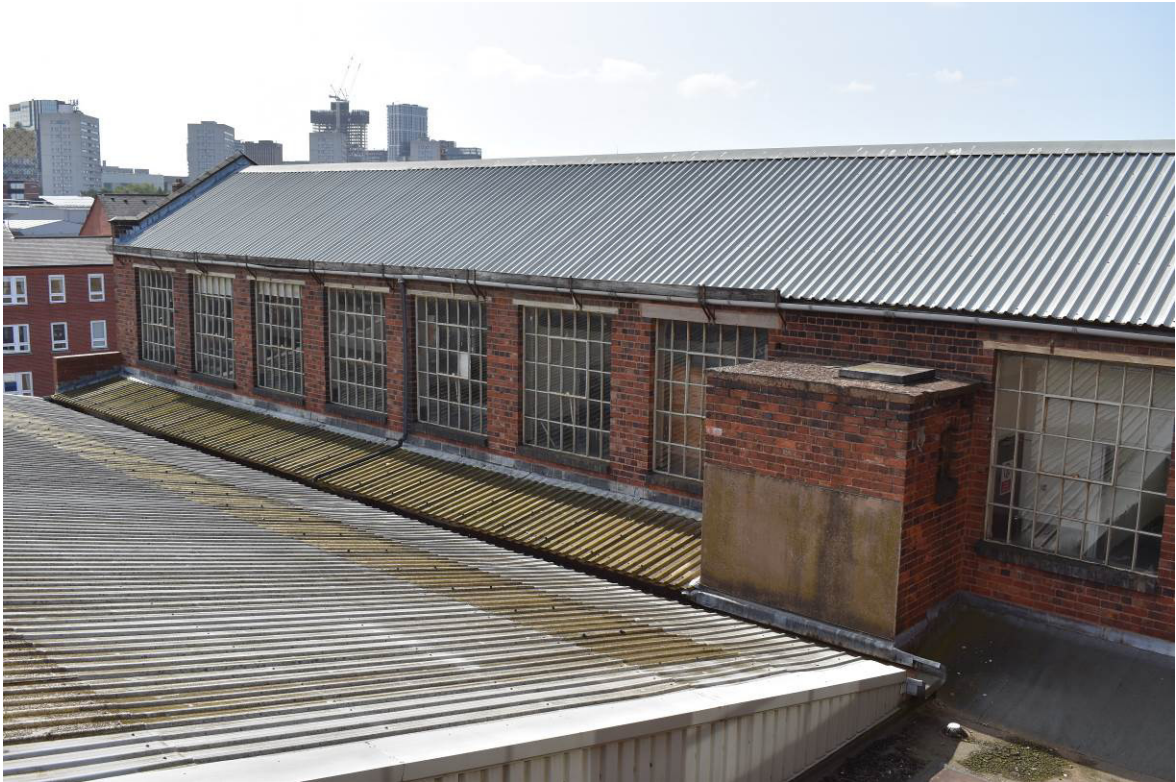
Plate 270: Building 13a; first-floor east elevation looking south-west, with ground-floor skylight and projecting turret.
