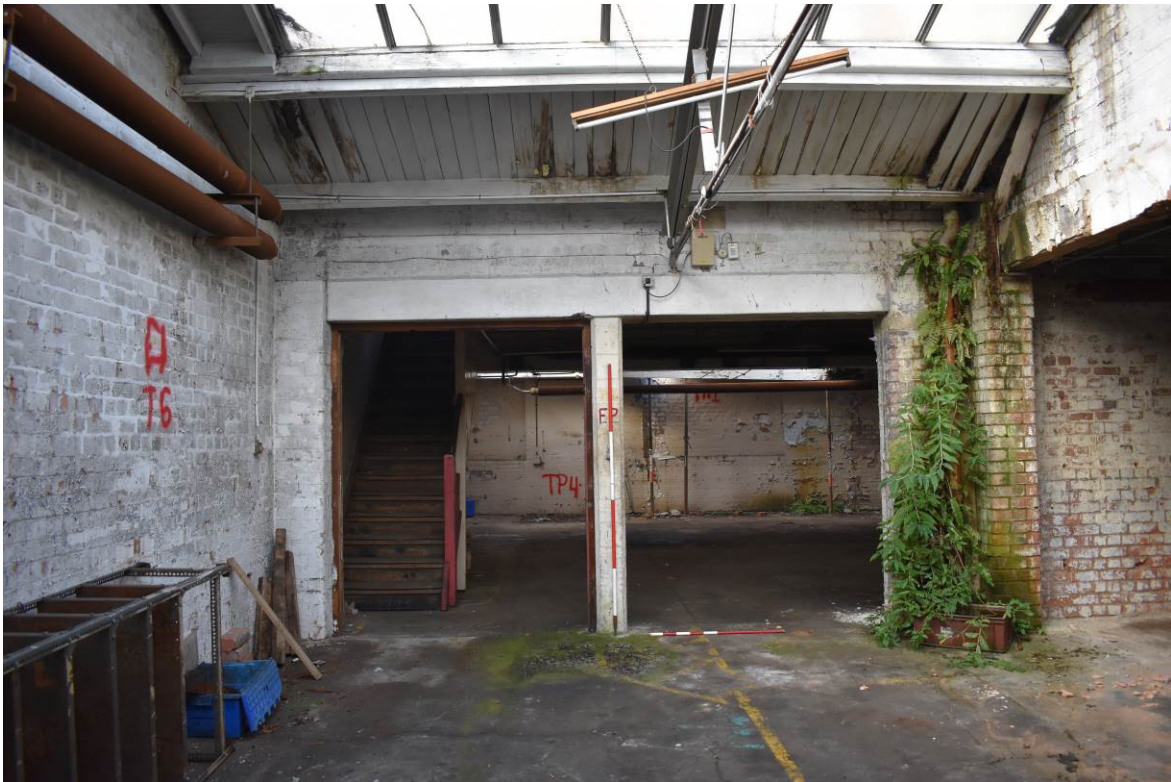
Plate 317: Covered yard 13f looking west, with primary open bays onto shopping range 13d.
