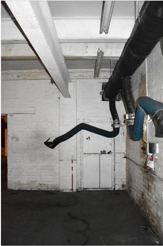
Plate 100: Longitudinal RSJ to east side of [G6], reflecting location of skylight marked on original plans.
