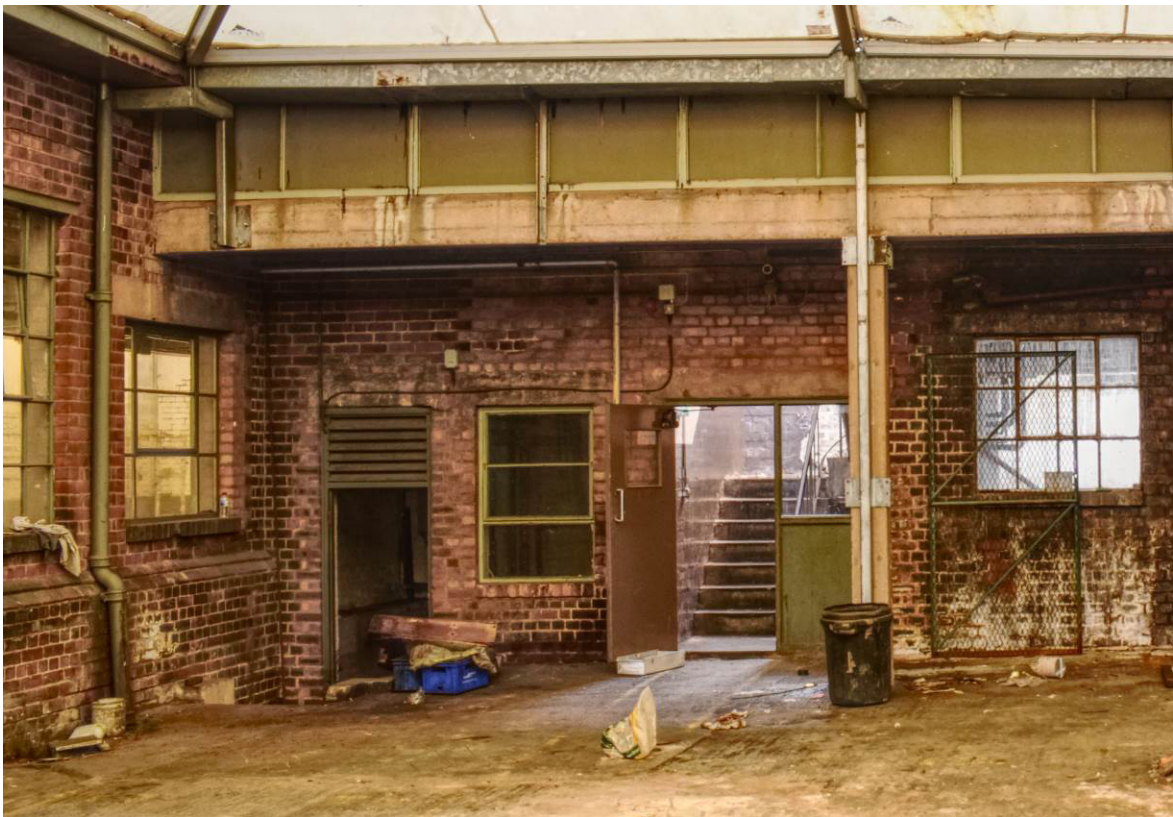
Plate 320: Boiler room 13h (left) and base of stairwell F (centre) as seen from covered yard 13j, looking south.
