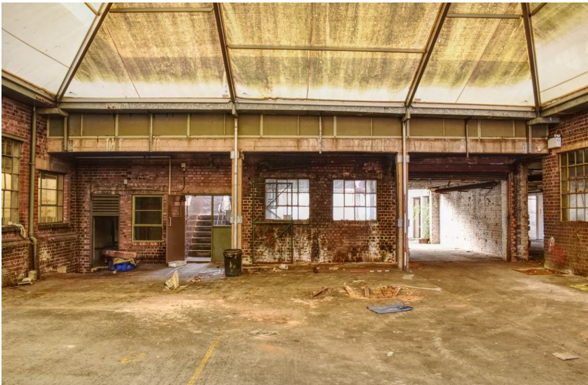
Plate 312: Building 13e (centre/right of image); ground floor as seen from covered yard 13j (NB. 13h and Stair F to left).
