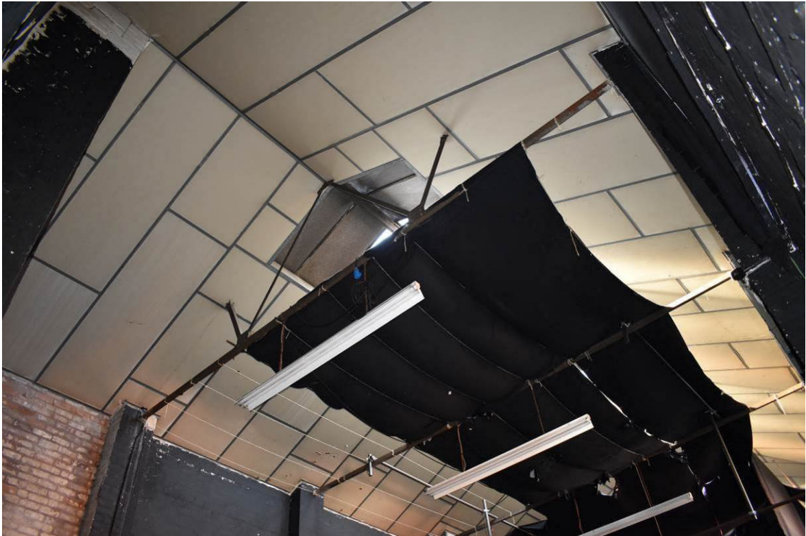
Plate 198: Building 11a: steel 'W' pattern Fink roof trusses introduced over lowered range in 1933.
