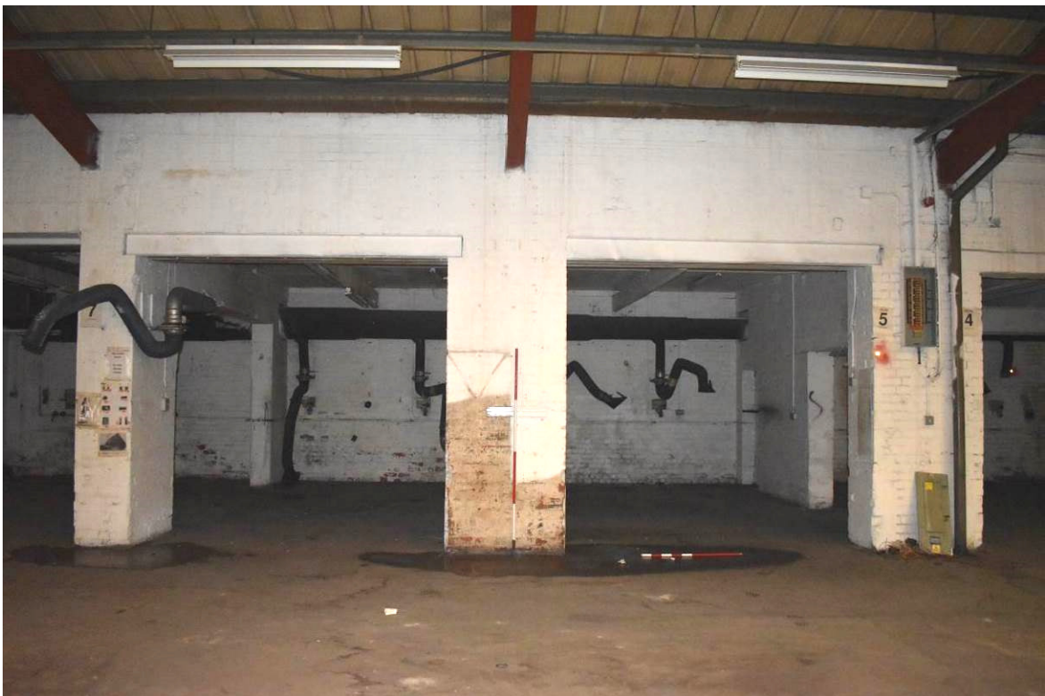
Plate 101: Building 7b; west elevation, Bays 9/10 to yard (with seg. brick arches above inserted concrete lintels).
