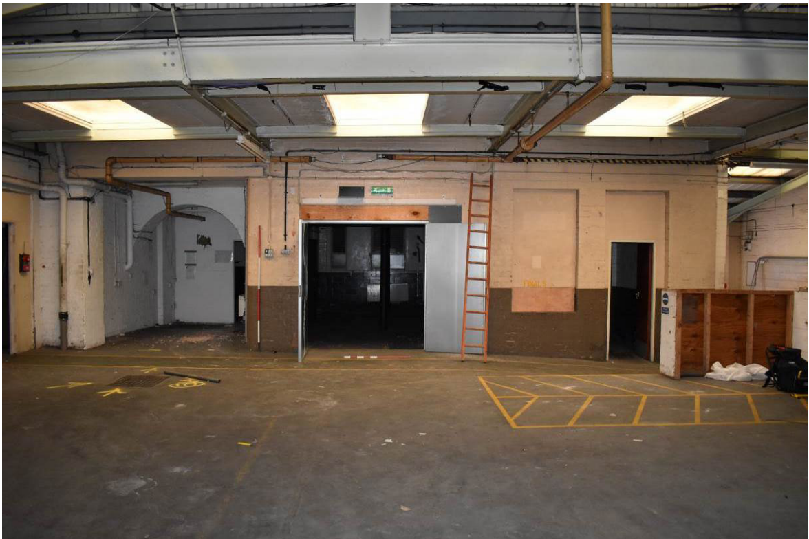
Plate 233: Building 12a: ground floor rear (south) elevation, visible within rear range; cart entry to left.
