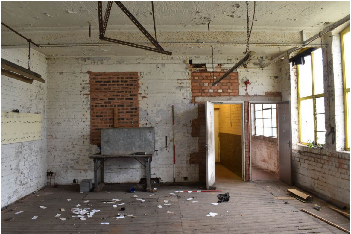
Plate 111: Building 7b, 1F; blocked windows to transverse wall at south side of Bay 7 (original, 1903 gable end).
