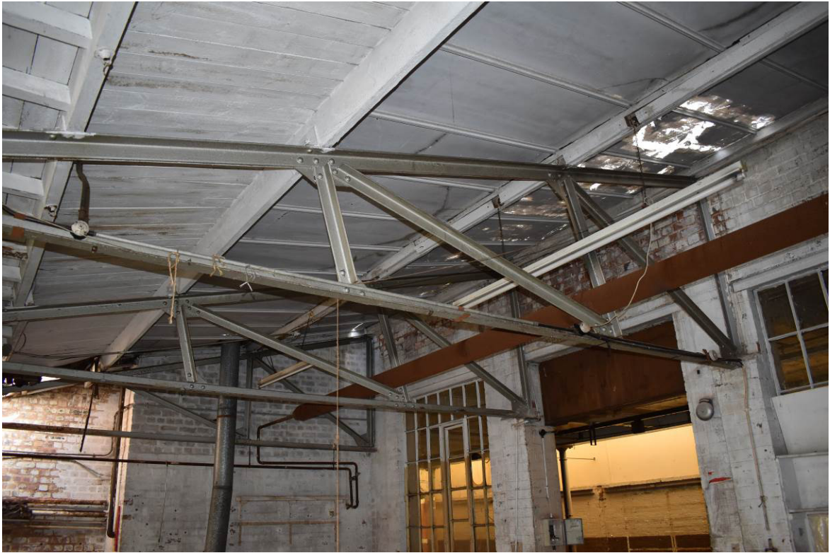
Plate 319: Steel ½-truss roof structure over covered yard 13g flanking shopping range 13a (to right).
