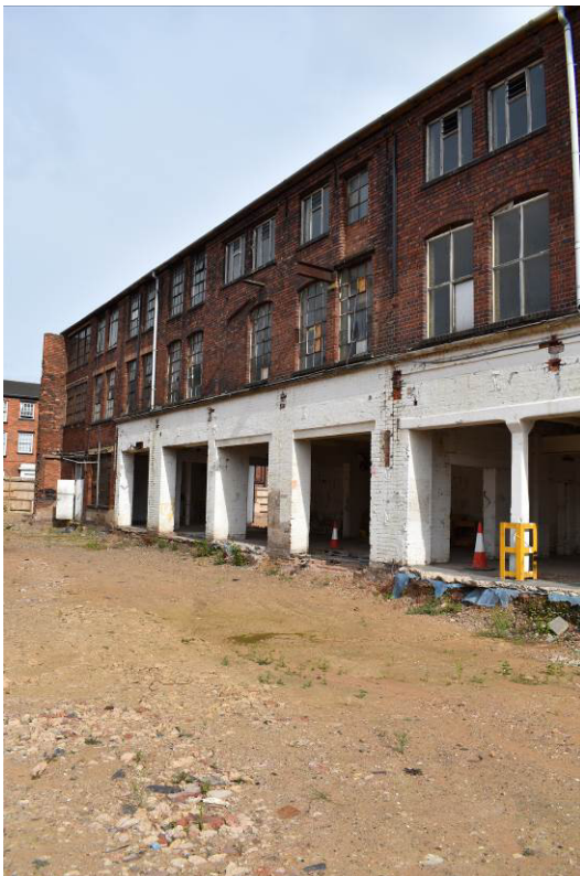
Plate 91: West elevation of Bldg. 7b after removal of covered yard 8 , looking north.
