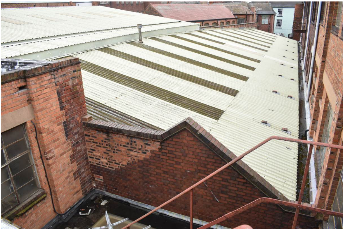
Plate 123: Roof of covered yard 8 looking north from roof of street frontage range 7a. Note brick gable of precursor covered yard to foreground.
