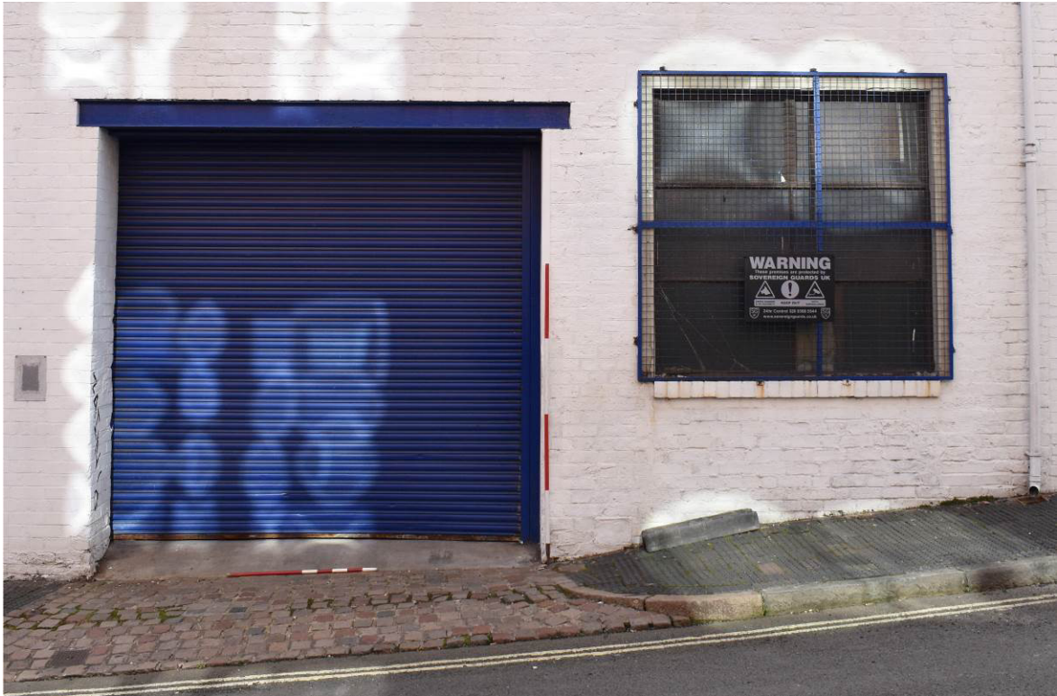
Plate 158: Bldg. 10b, James Street façade; roller door and adjacent, former cart entry, modified to house window.
