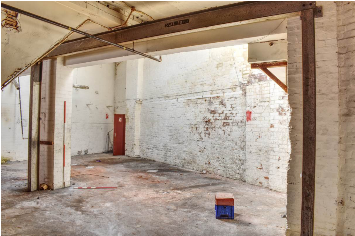
Plate 164: West side of 10b open to covered yard 10c at basement level (openings formed in 1928).
