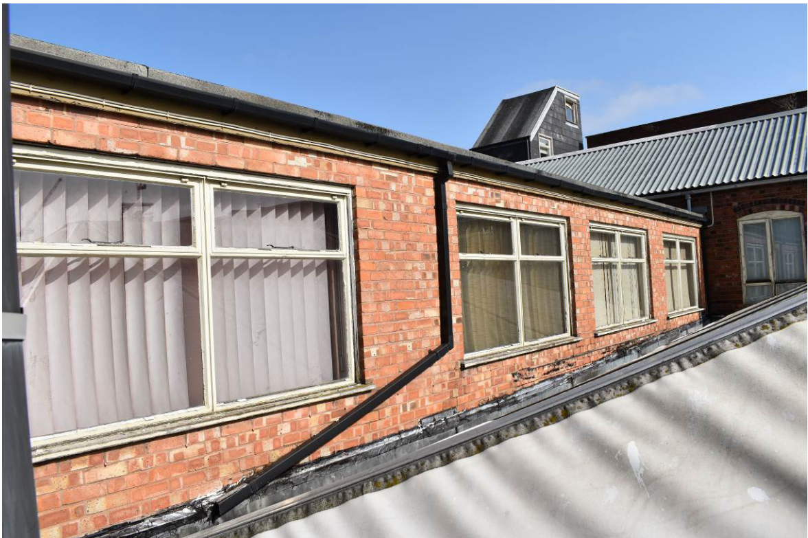
Plate 287: Building 13b; 1970s first floor extension (extending over cart entry [G5] to left)
