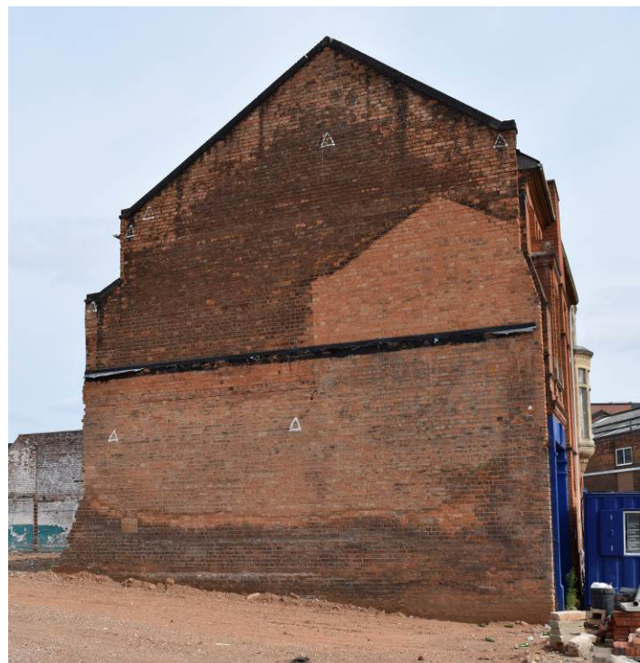
Plate 11: 'Ghost' of early street frontage range of No. 113, evident on west gable end of Bldg. 1 following demolition of Bldg. 4 (21.09.21)
