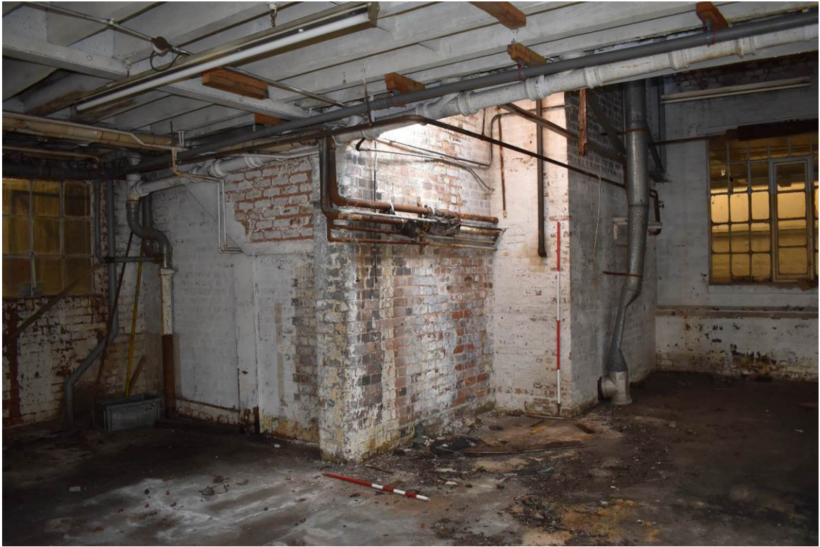
Plate 321: Boiler room 13h (right) and adjacent stairwell F (centre) as seen from [G12] looking north-east.
