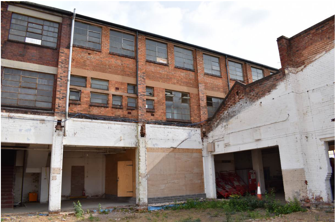
Plate 62: West elevation of eastern return of frontage range 7a , as observed after removal of covered yard 8 (21.09.21)
