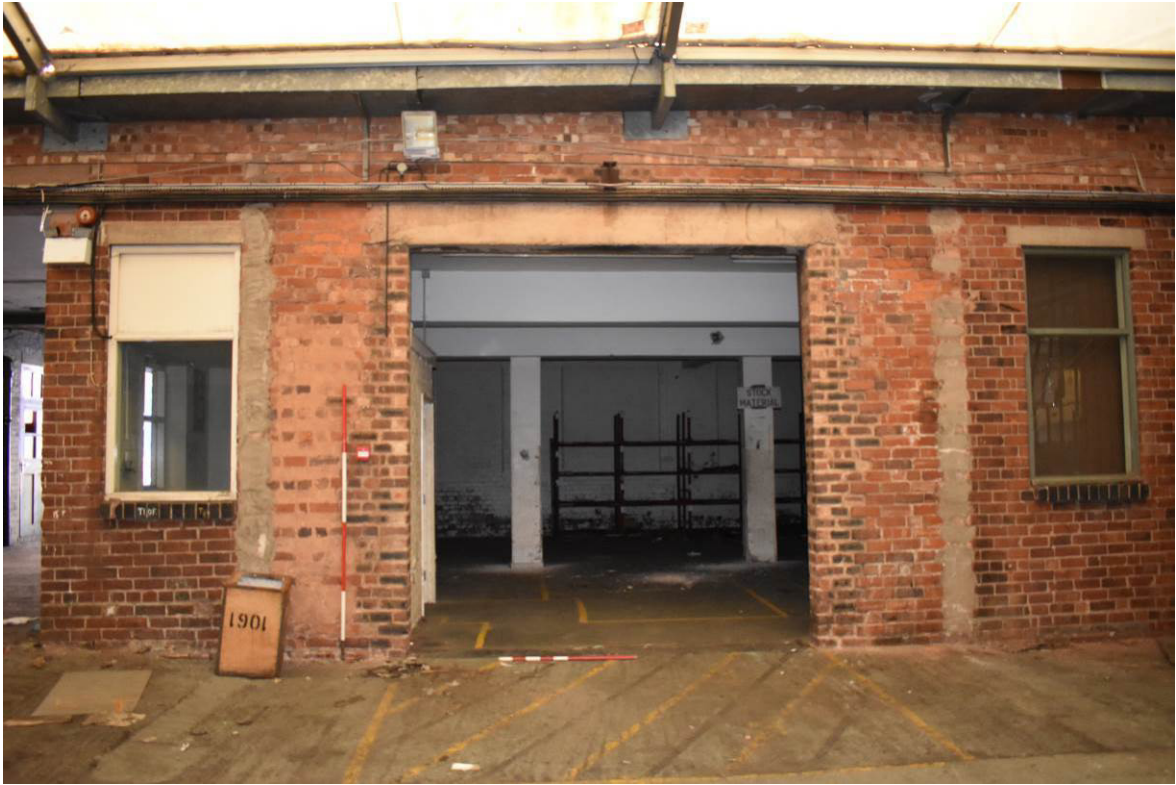
Plate 286: Rear (south) elevation of building 13b; GF as seen from covered yard 13j with cart entry [G5] to left.
