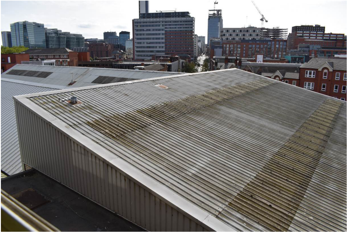
Plate 248: Building 12b; view over mono-pitch roof from 2F (room S6) of Building 12a.
