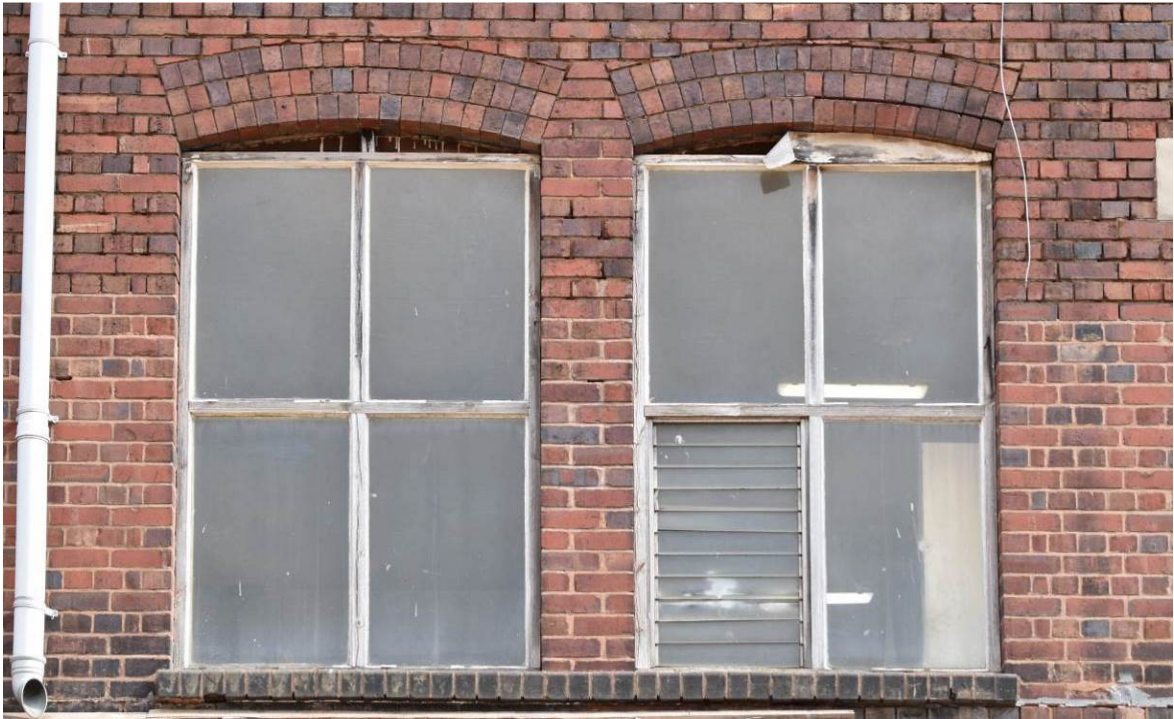
Plate 93: Building 7b: Segmental-headed windows with triple-header arches and secondary timber casements (Bay 7, 1F).
