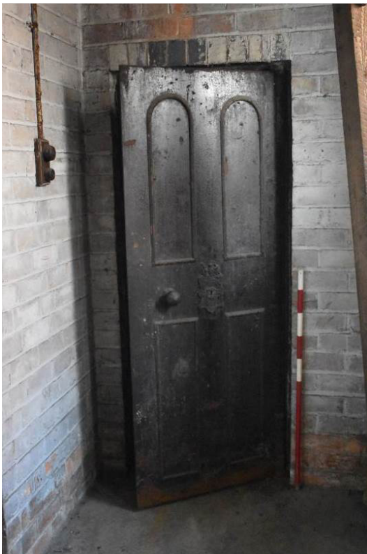
Plate 141: Strong room [B2] door.
