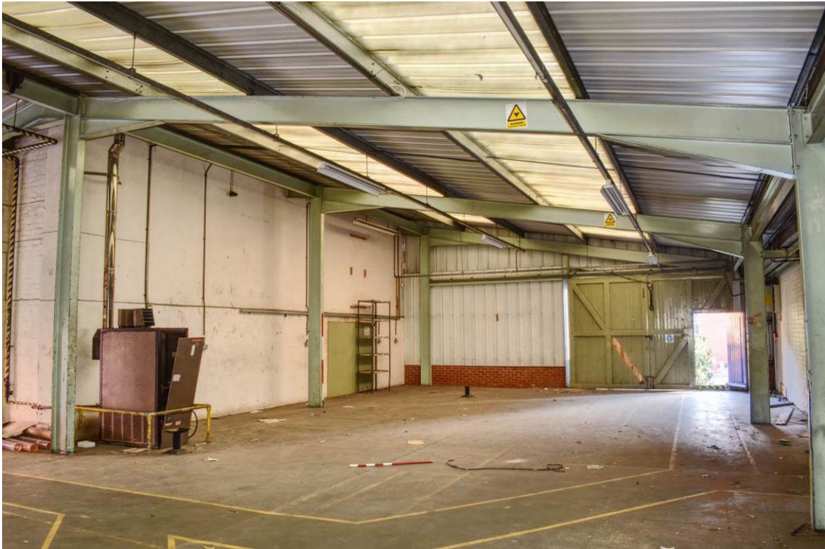
Plate 219: Building 11d; interior looking east, mono-pitch roof to eastern bays (south elevation of Bldg. 11a to left).
