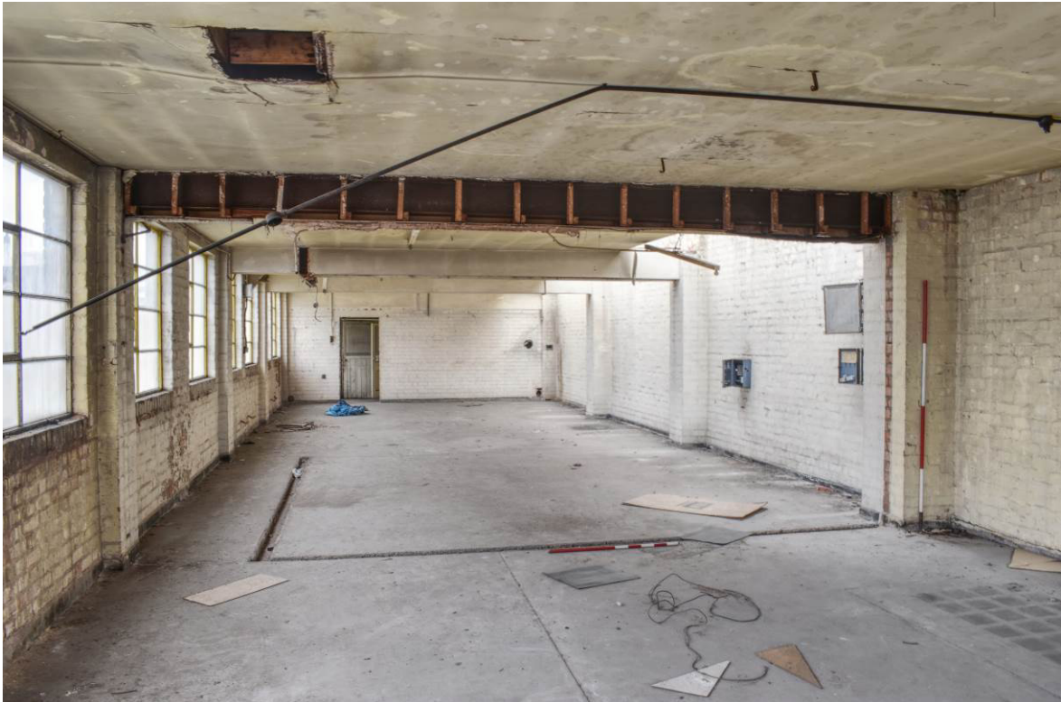
Plate 86: Second floor room [S2] looking north; note scarring to floor indicating former subdivision of space.
