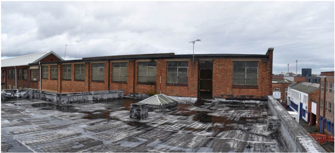
Plate 61: Secondary upper floor level over eastern return of 1945 street frontage block 7a .
