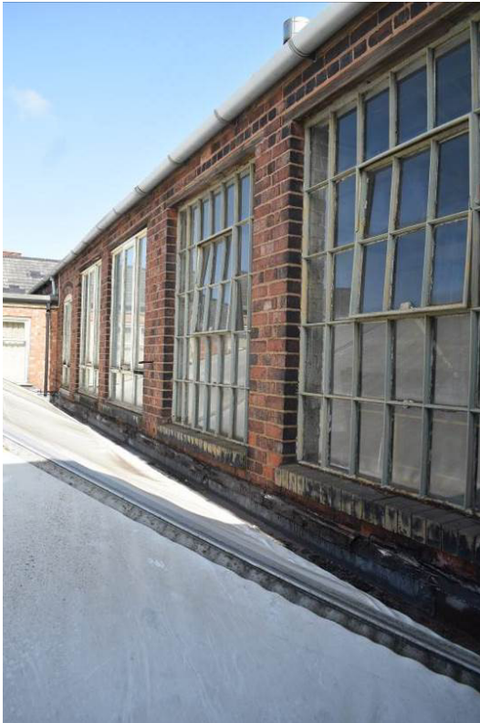
Plate 263: Bldg. 13a, west elevation (1F) as seen from raised link passage 13I.
