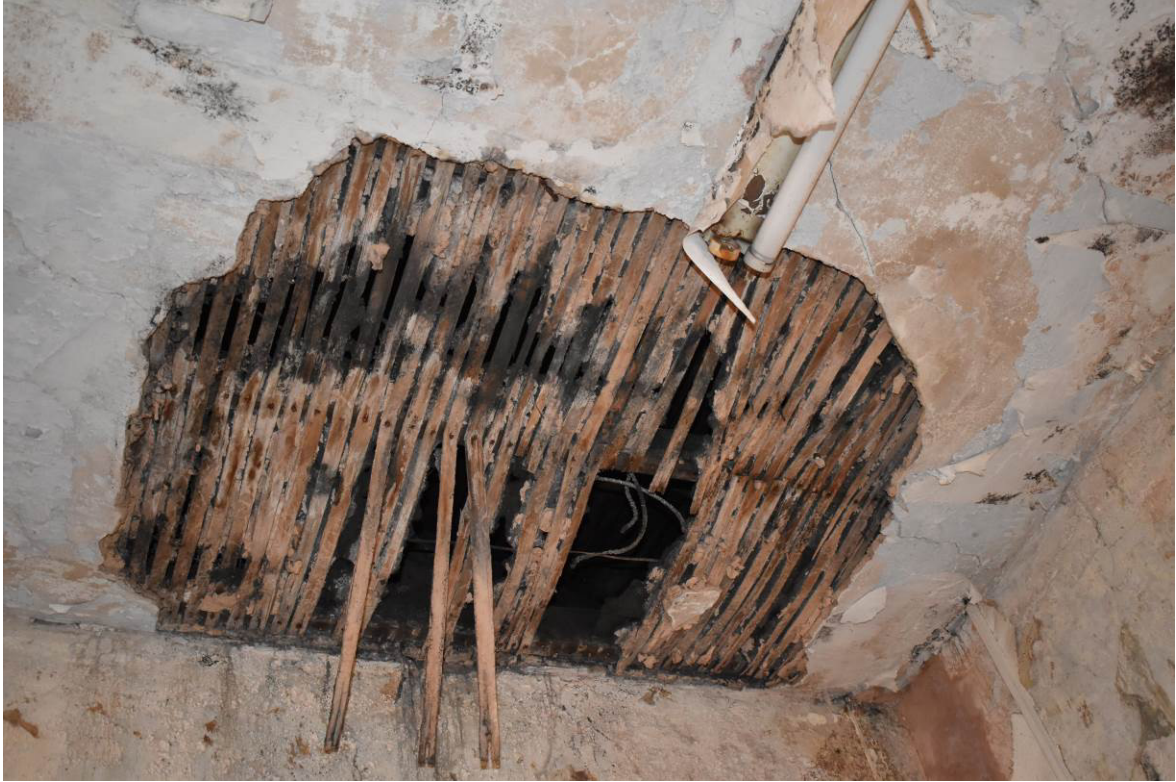
Plate 175: Section of lath and plaster ceiling exposed to ceiling of [LF3]
