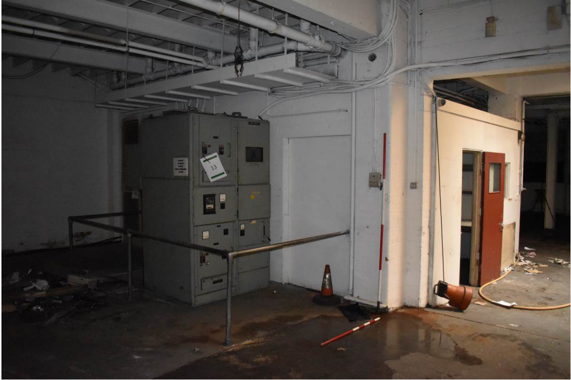
Plate 72: Sub-station / 'power house' [G3] to north-east corner of GF.
