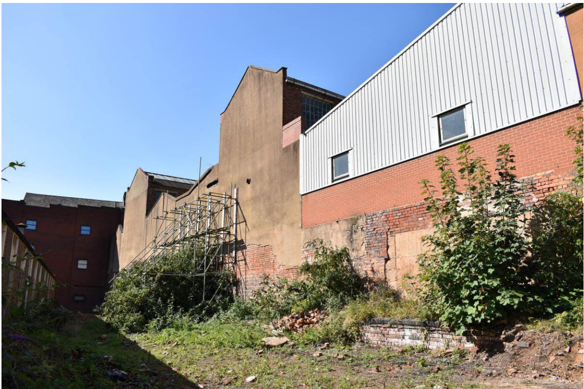
Plate 335: Building 14; rear yard, looking west, backing onto tall 'retaining wall' forming back of Bldgs. 12/13.
