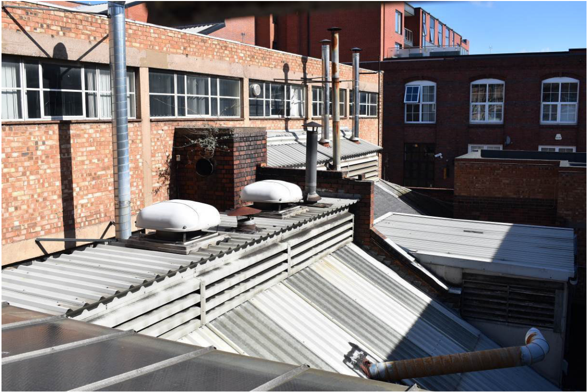
Plate 350: South elevation of Building 15a abutted at lower levels by pre-existing component ranges of Building 2c.
