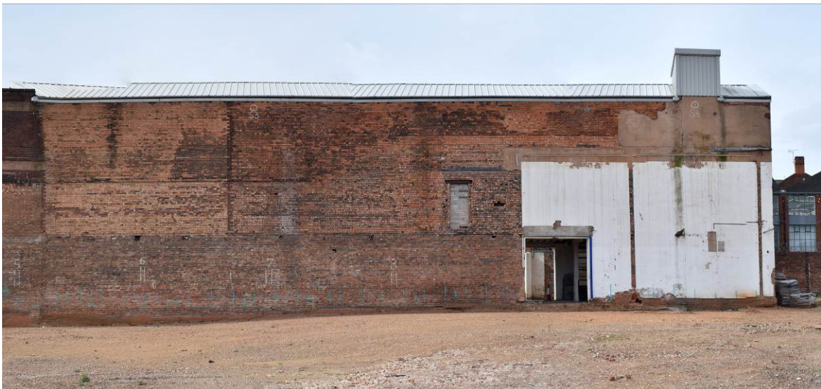
Plate 96: Building 7b; east elevation (after removal of Bldg. 6). NB. clear change in brickwork at 1F level.
