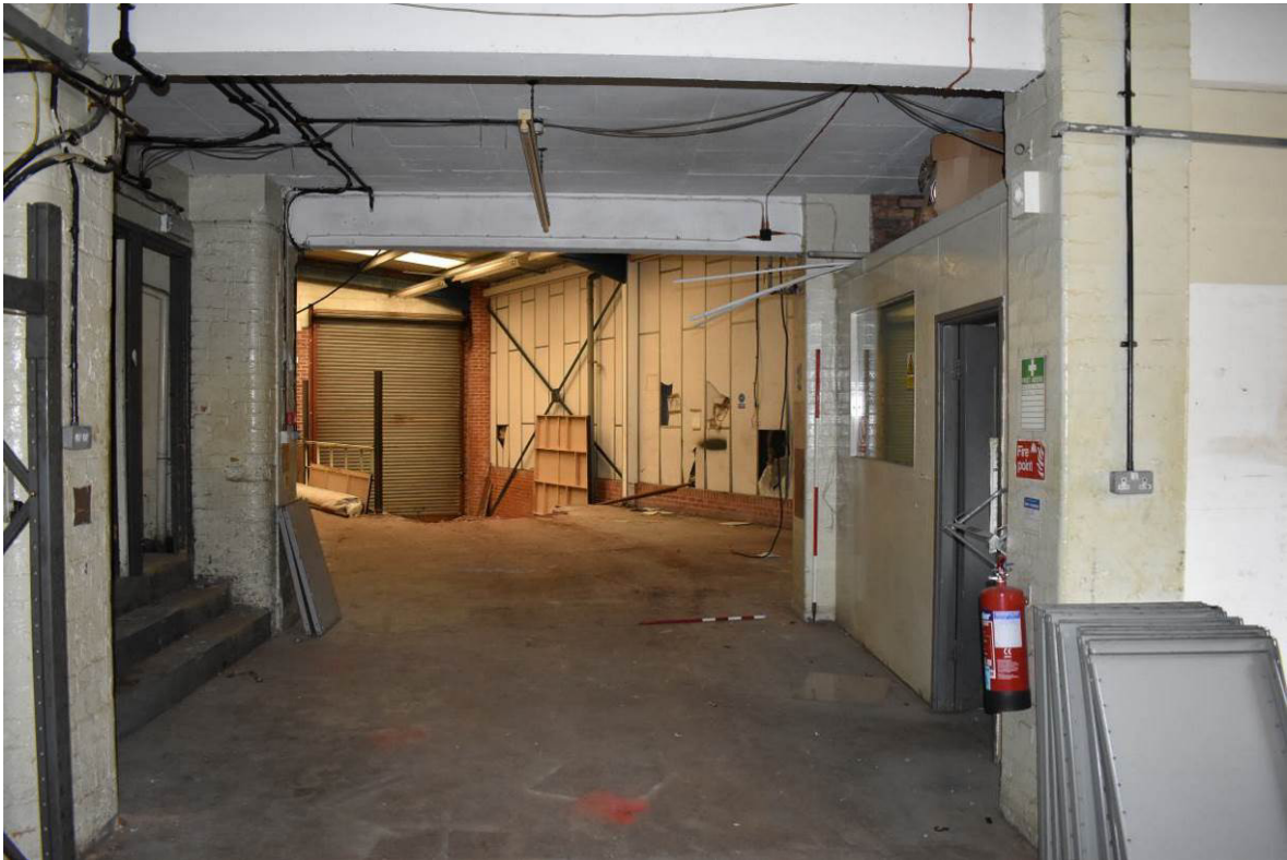
Plate 209: Basement open to Bldg. 10d (former carpenter's shop') at east end of range 11b.
