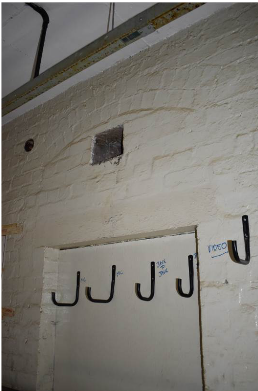
Plate 205: Building 11b; double-header brick arch of original window opening to north wall.
