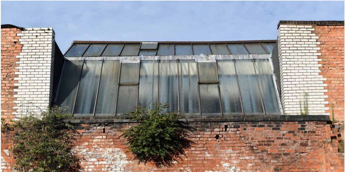
Plate 27: Building 5: detail of patent-glazed roof light with associated areas of white-glazed brickwork.
