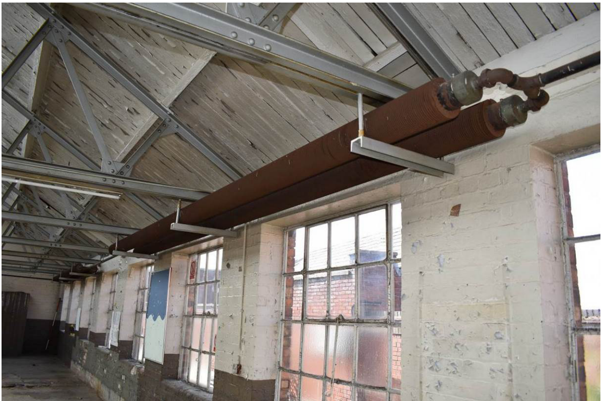
Plate 309: Shopping range 13d; first-floor, eaves-level, finned heating pipes.
