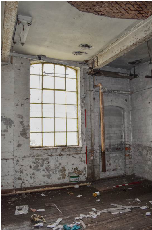
Plate 112: Building 7b, 1F; blocked door at Bay 10 (N). originally serving raised link-bridge.
