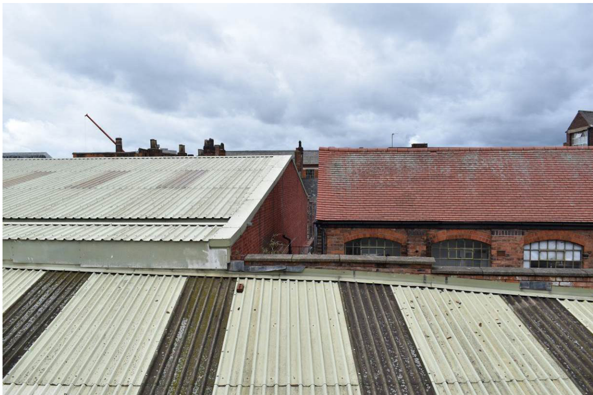
Plate 125: Building 9; blind north gable end, backing onto workshop range of Deakin and Francis of Regent Place, looking west over mono-pitch roof of covered yard 8 from 2F level of Bldg. 7.
