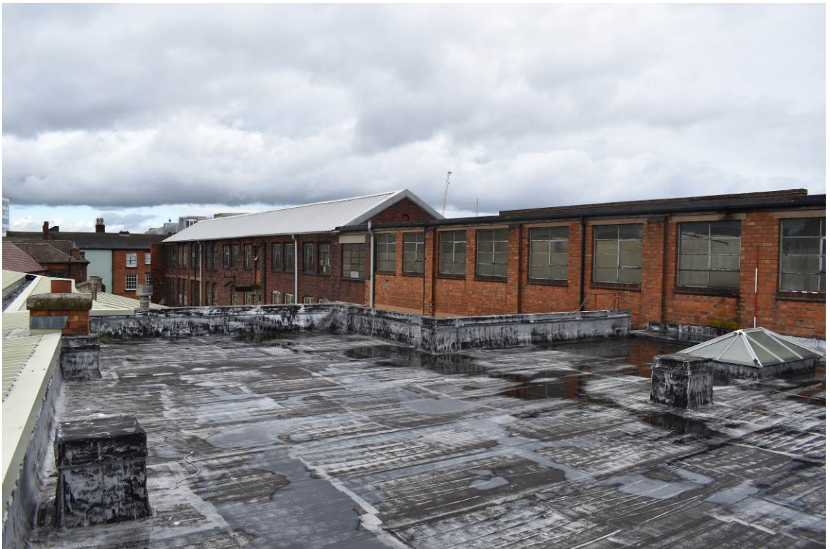
Plate 89: Looking north-east over flat roof of Bldg. 7a; pitched, patent -glazed rooflight to right lights former passage [F2].
