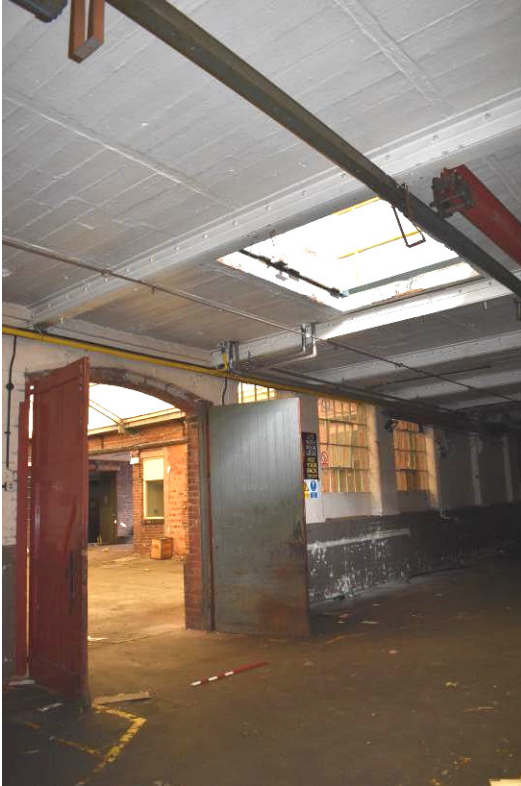
Plate 275: [G2], Bay 4 with access door and ceiling void over. NB. concrete beam ceiling.
