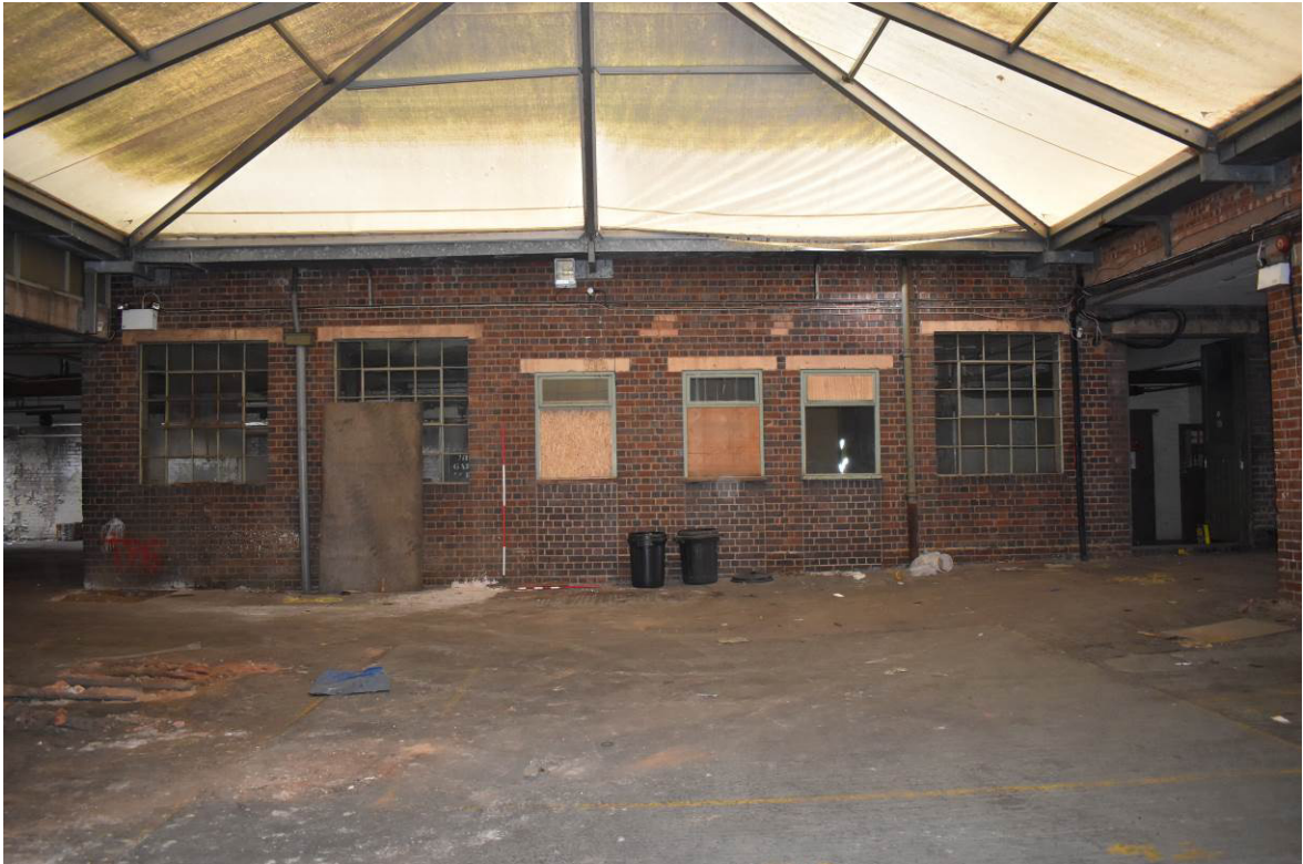
Plate 293: East elevation (Bays 2-4) of shopping range 13d ; GF as seen from covered yard 13j with cart entry to right. NB. three blocked doors to centre originally served coal, coke and petrol stores (later combined as [8a/b] ).
