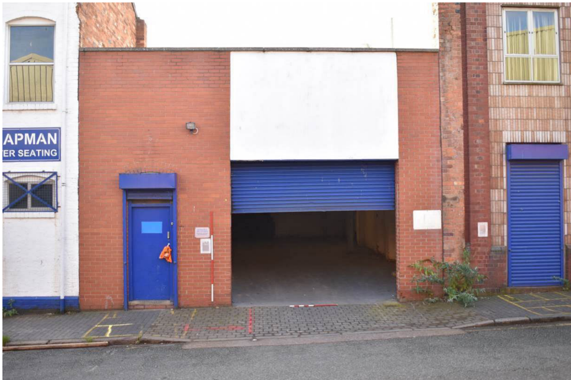
Plate 218: Building 11d; late 20 th -century entrance bay to Northwood Street at west end of truncated range 11a (replacing five original window bays of latter structure).
