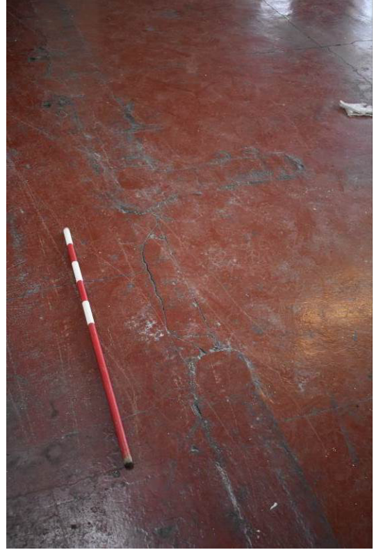
Plate 78: Scar of former partitions to floor.
