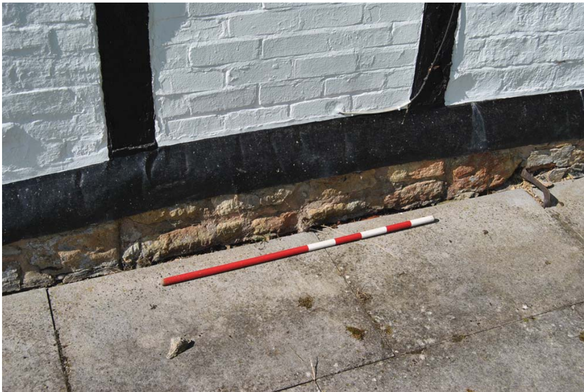
Plate 5: Paired straight joints in rubble stone plinth denoting blocked doorway of former cottage.
