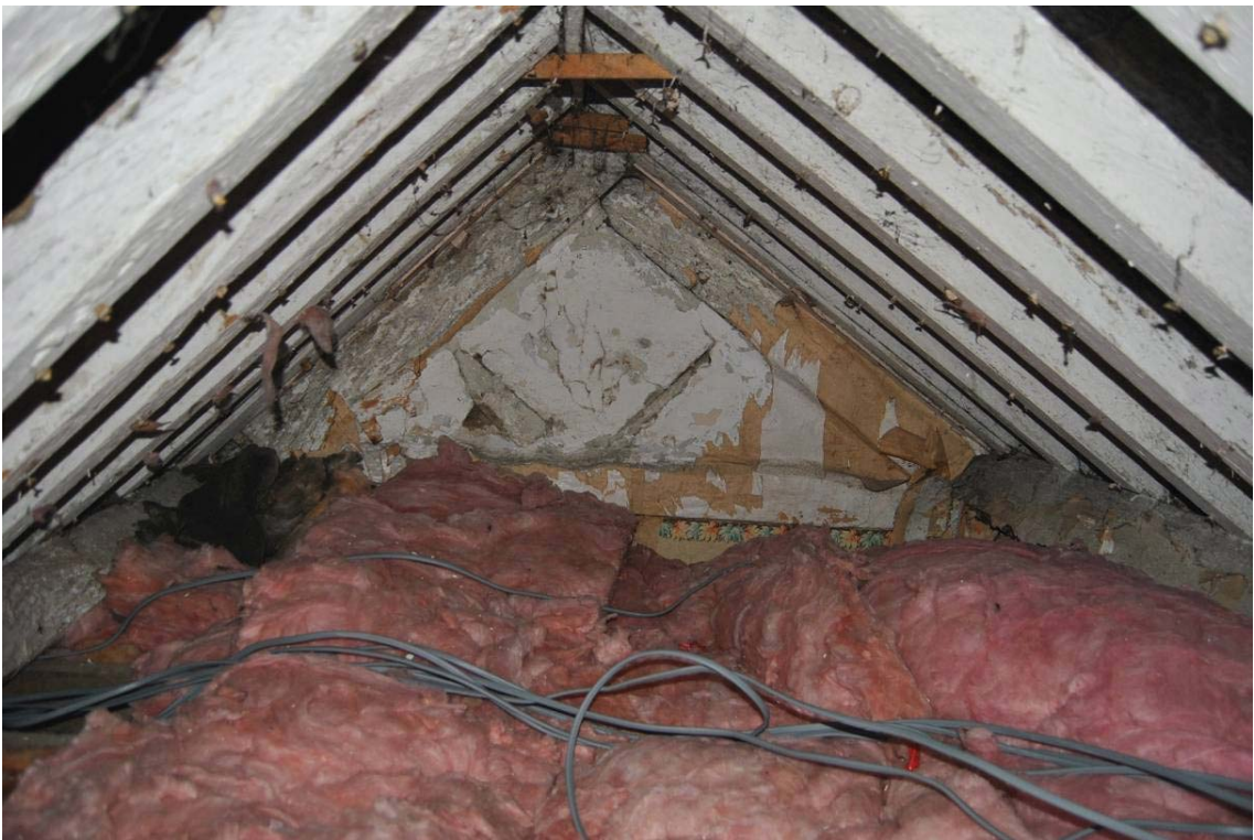
Plate 47: Easternmost truss with v-strutting above collar (photographed from ceiling hatch within [F.09]).
