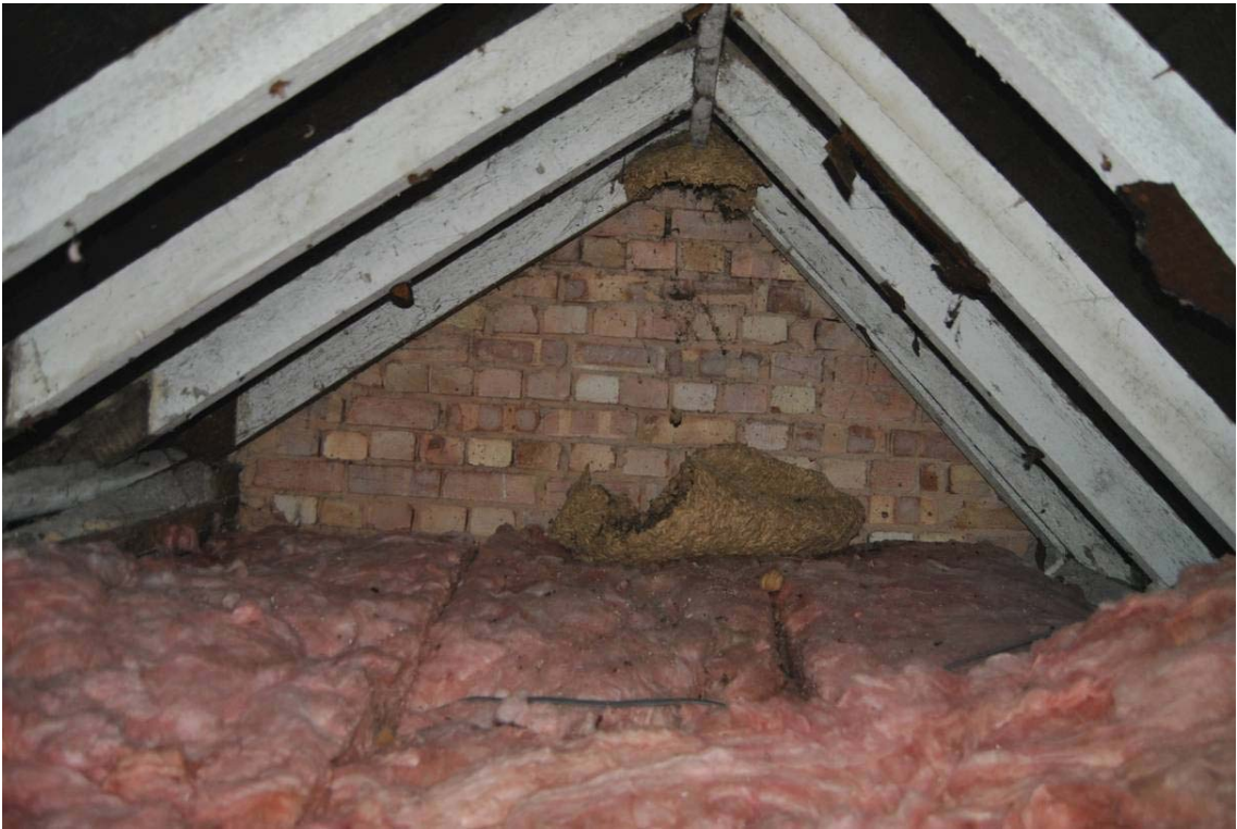
Plate 46: Western gable rebuilt in stretcher bond brick (photographed from ceiling hatch within [F.02]).
