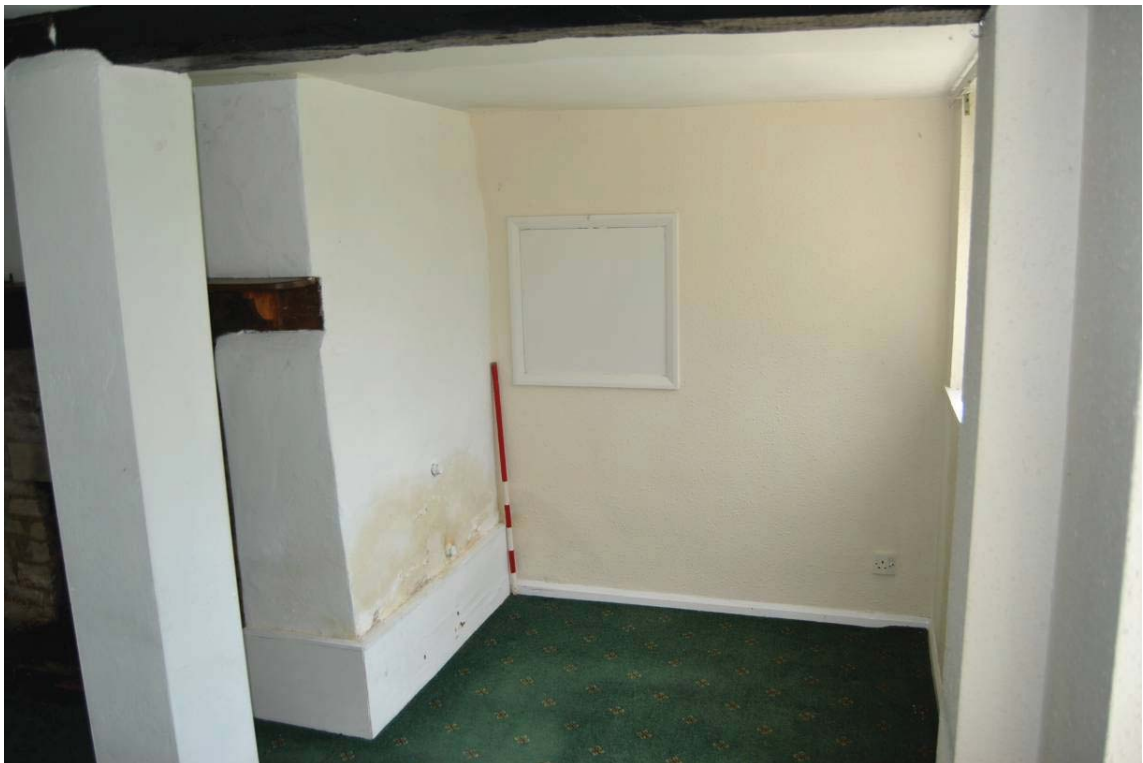
Plate 34: [G.06] looking east to south of stack; NB: transverse beam supported by brick pier (left).
