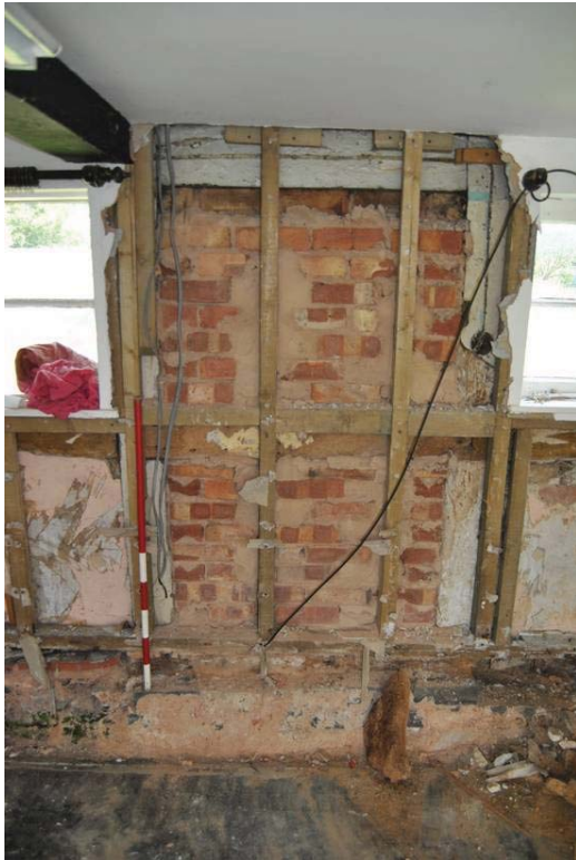
Plate 14: Blocked doorway to front elevation.
