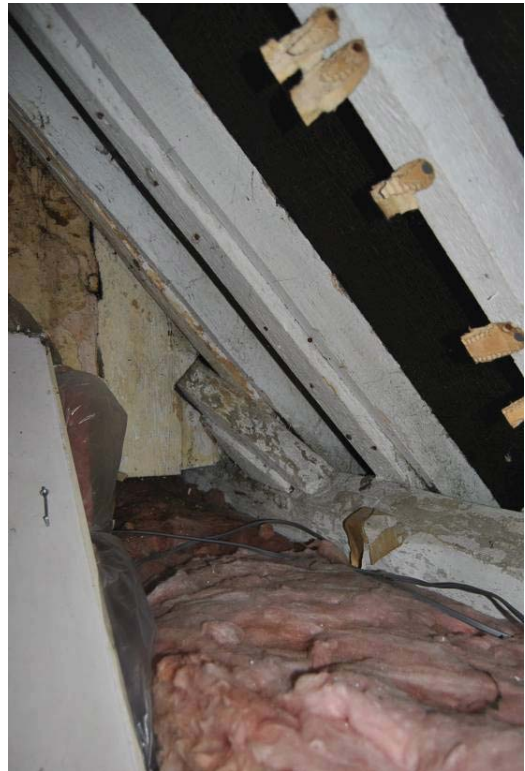
Plate 49: Detail of diagonal brace passing over back of purlin (see also Plate 25).
