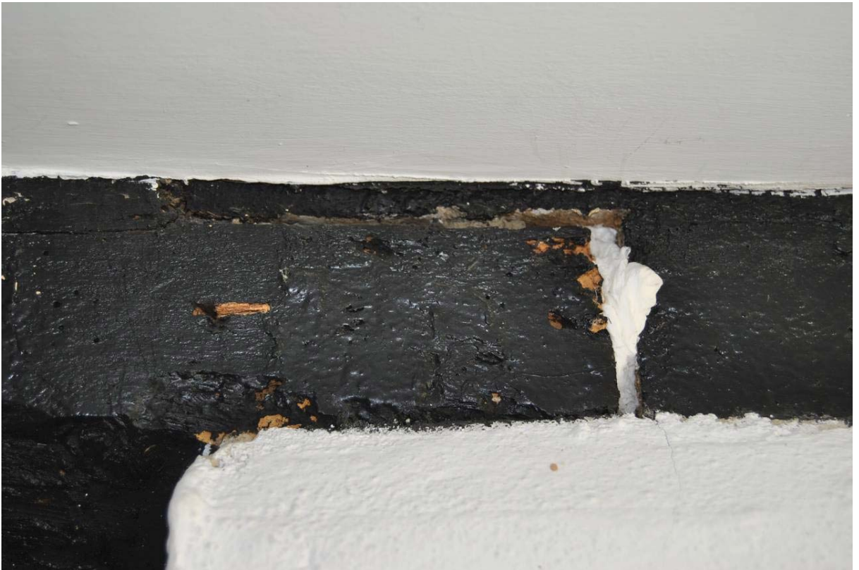
Plate 36: Transverse beam; detail of simple scarf at support pier.
