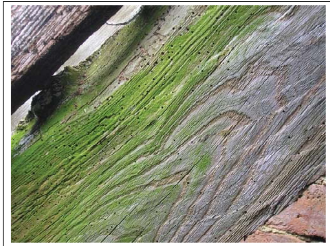
Figure 2: A further characteristic of elm is the presence of worm holes, not only on the sapwood (upper LH part of timber), where it is also found on oak, but also across the face of the timber. This photo also shows the 'swirled' and 'flecked' grain on the surface of the wood.
