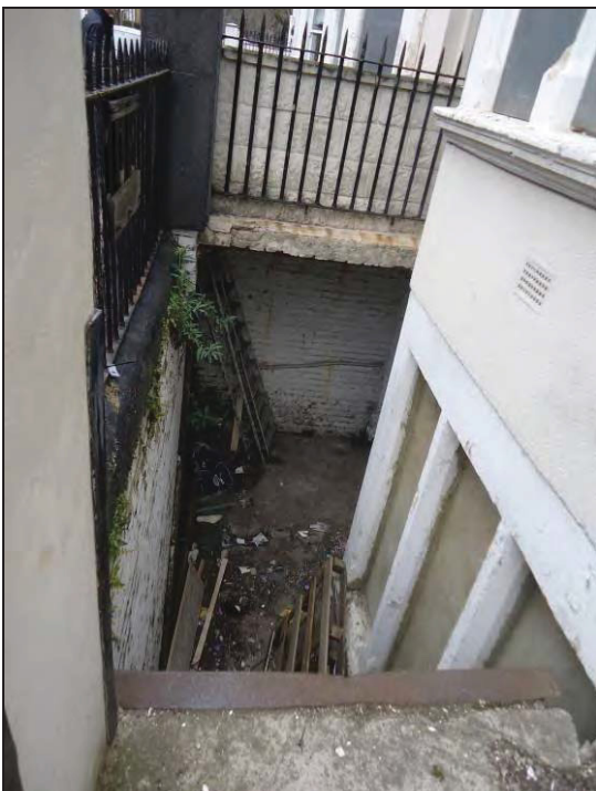
Photograph 4: Showing light well to basement at the front of the building (C. Mitchell, April 2013).
