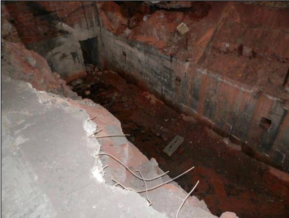
Photograph 9: Example of a large pit in the former press shop.
