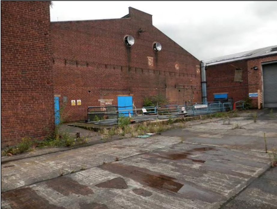
Photograph 3: Elevation of brick built workshop in centre of the site with blocked openings.
