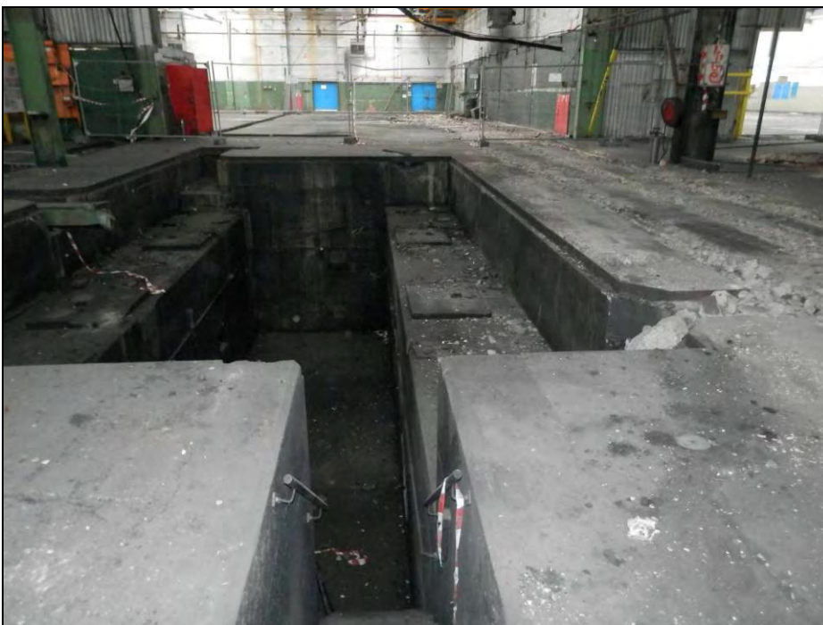
Photograph 8: Example of a large pit in the press shop.
