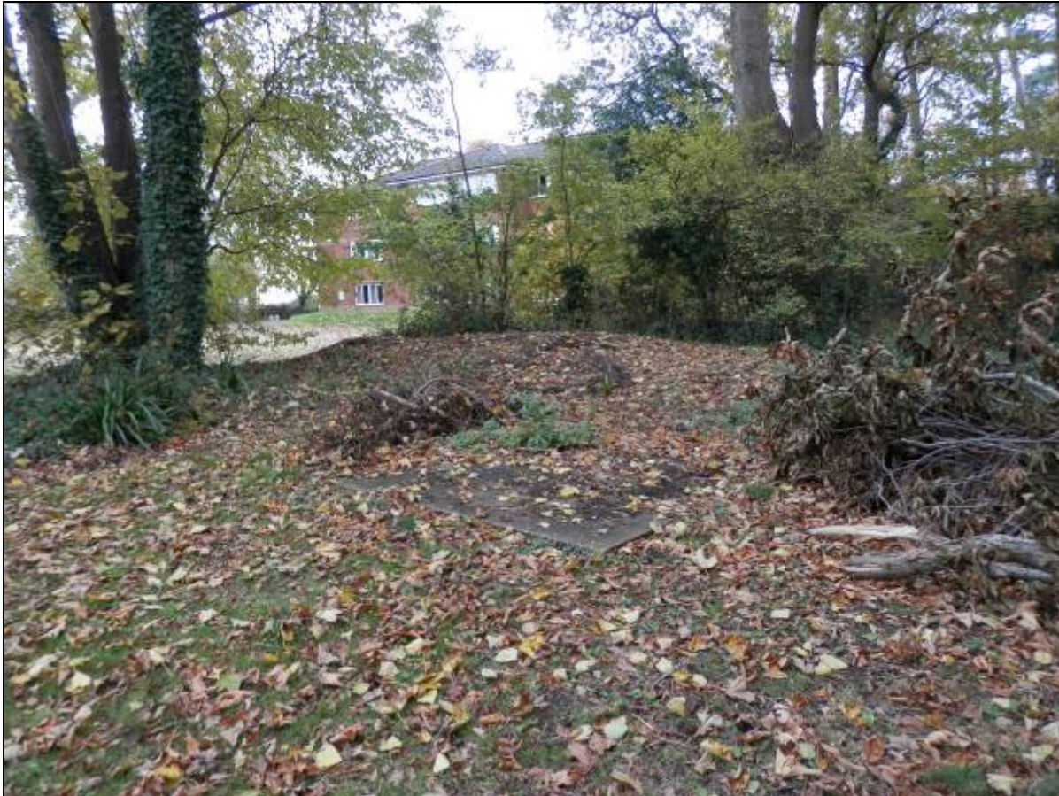
Photograph 6: Inspection cover and semi-buried, probable septic tank at the west end of the pond and immediately north of the wooded path.
