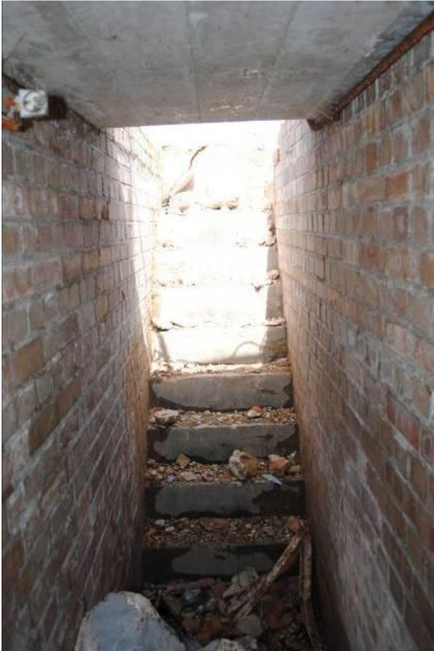
Photograph 19: Rubble strewn entrance to Shelter 3.
