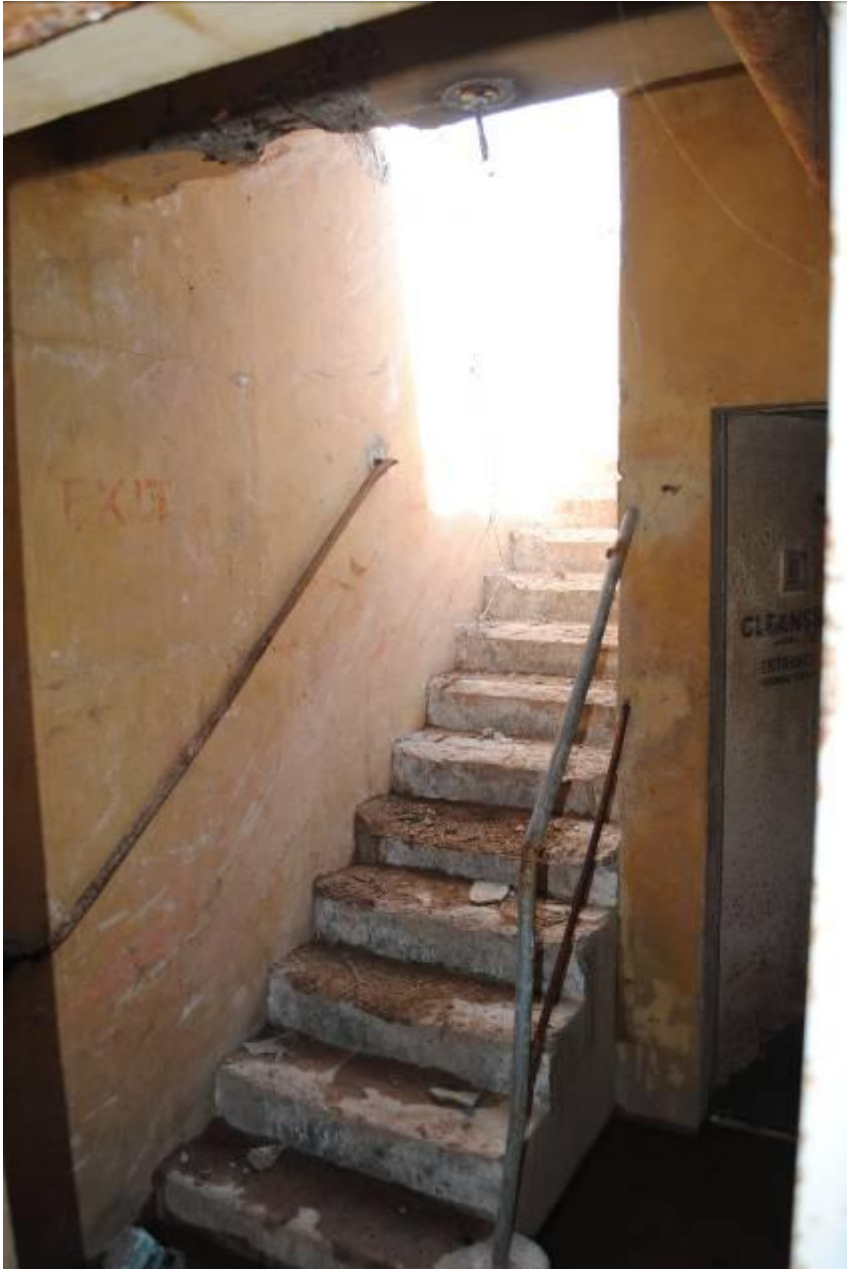
Photograph 11: North access to surface showing stencilled signage. The indicative cartoon hand remains visible to the right of the EXIT sign.
