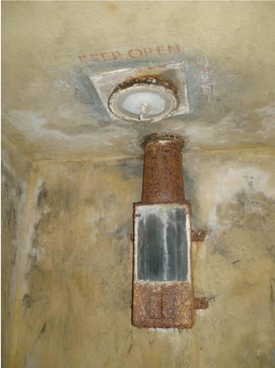
Photograph 12: Corroded stink pipe and air filter in chemical closet, Shelter 1.
