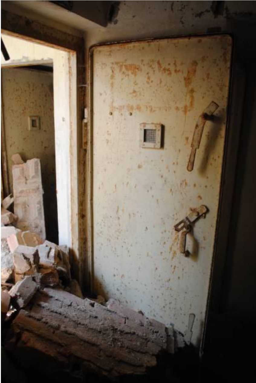
Picture 3: Southern entrance to Shelter 1, showing rubble from demolition of surface buildings and surface access to the shelter.
