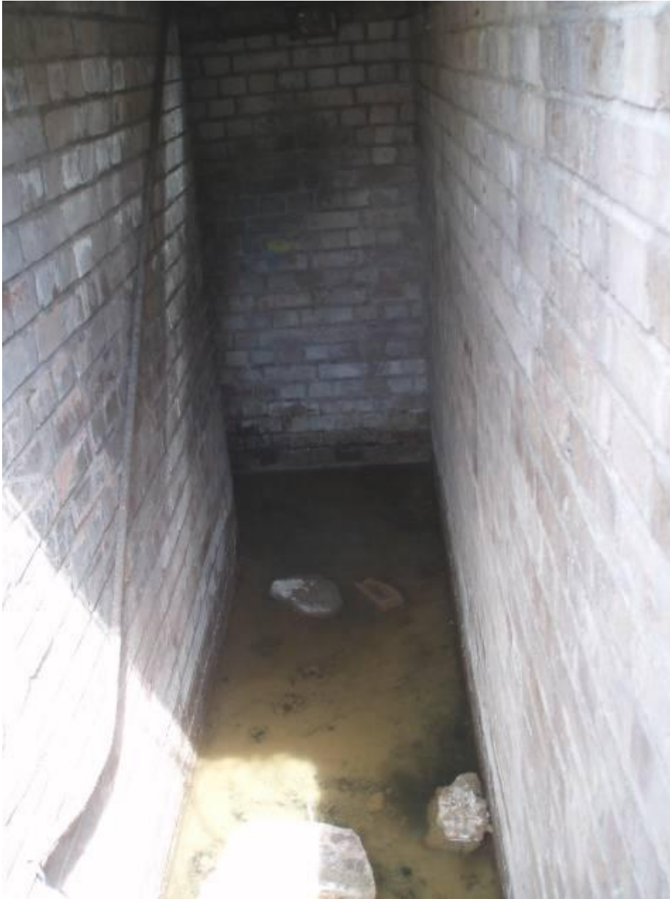
Photograph 15: Standing water in the eastern entrance to Shelter 2.
