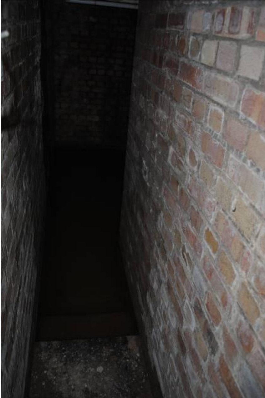
Photograph 16: Standing water in the cross passage between east and west galleries of Shelter 2.
