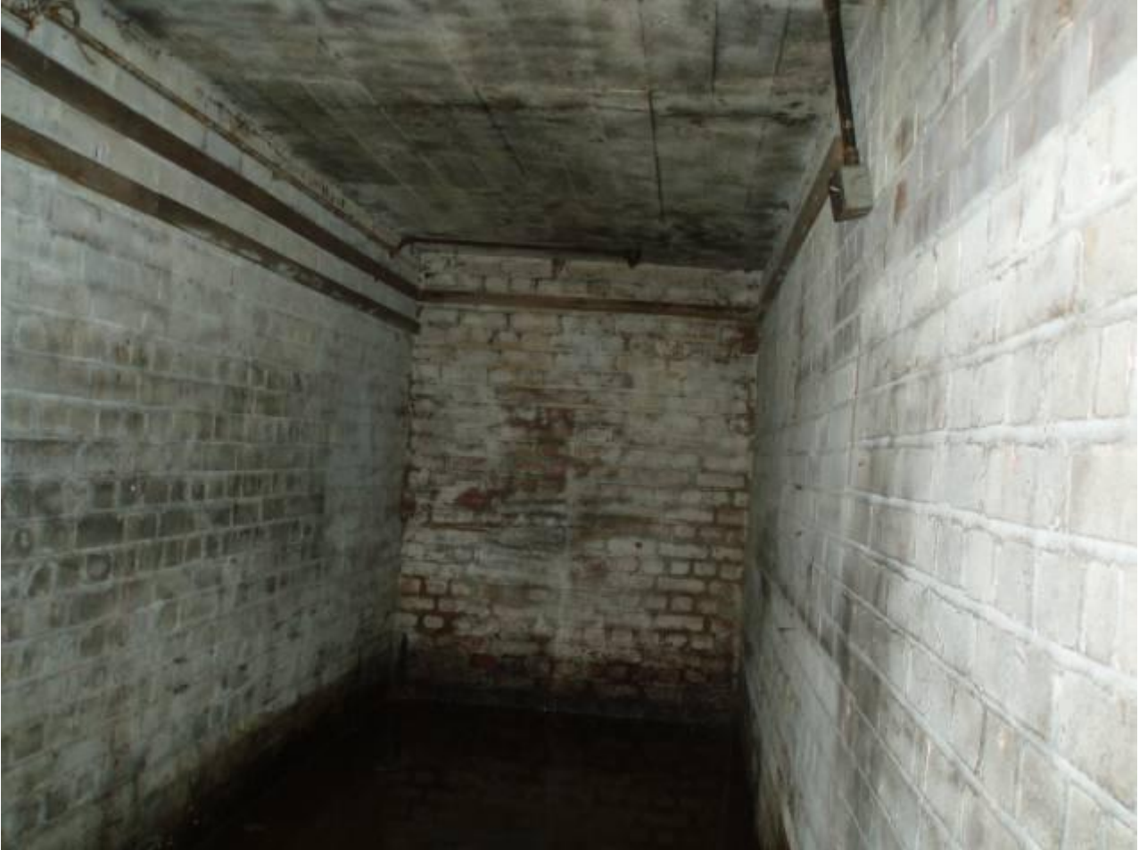
Photograph 17: East Gallery of Shelter 3 showing standing water and the wall blocking the passage.
