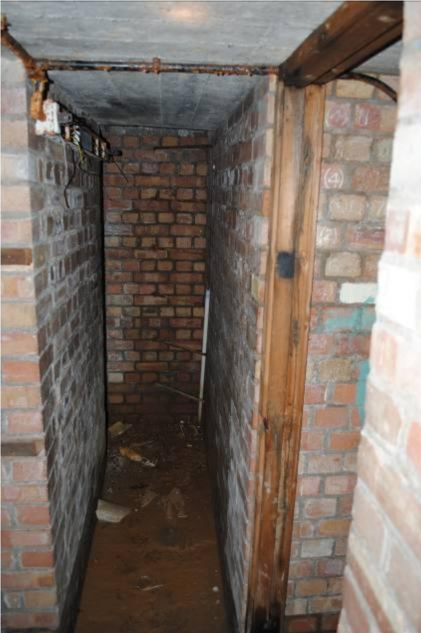
Photograph 18: Entrance to Shelter 3 eastern gallery and door to the chemical closet (right).
