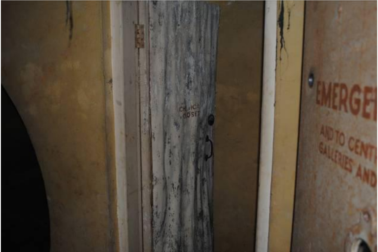
Photograph 7: In situ blast door and door to the Chemical Closet showing the adverse effects of damp on the door.
