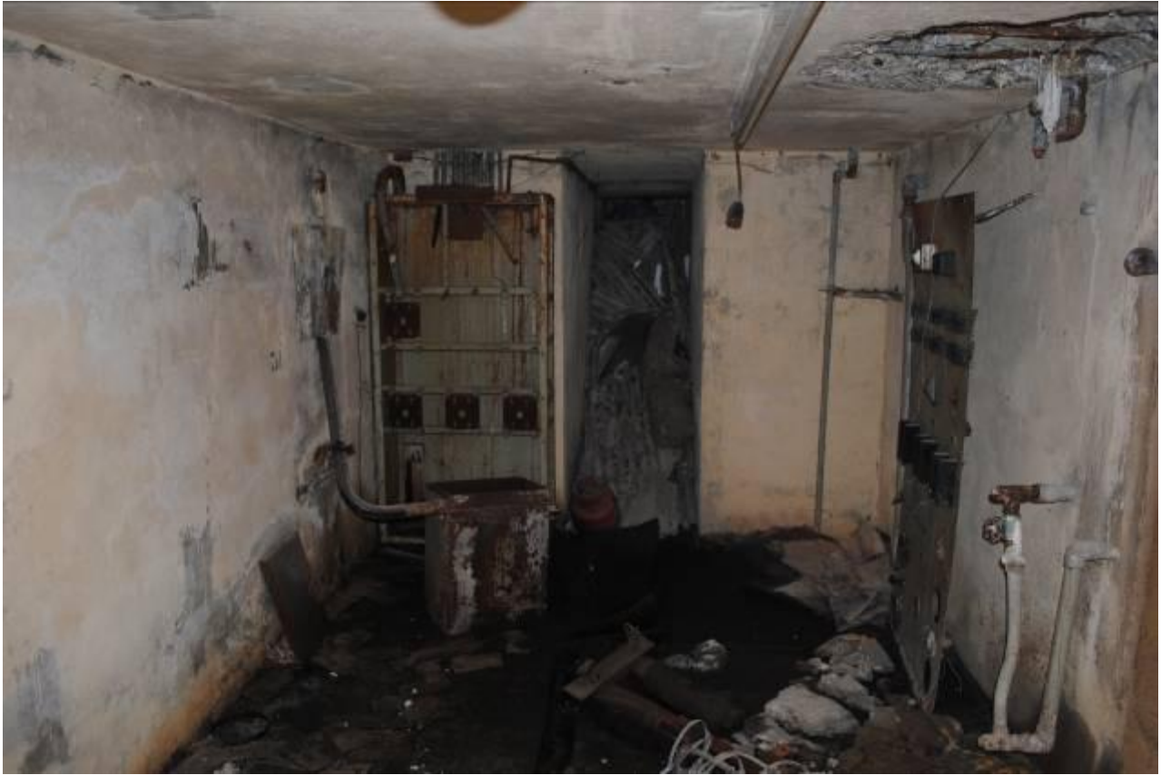
Photograph 5: Interior of the Plant Room, showing damage to the Control Panel and rubble blocking the escape passage.
