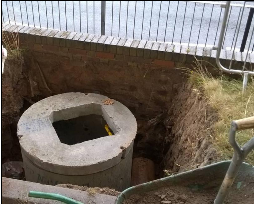
Picture 7: View south into the excavation showing the installed inspection chamber (prior to the installation of the hatch).
