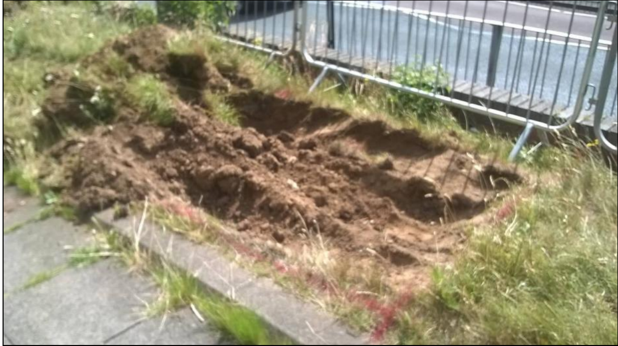
Picture 1: General view of the excavation area seen from the north-west showing ground conditions at the commencement of works.
