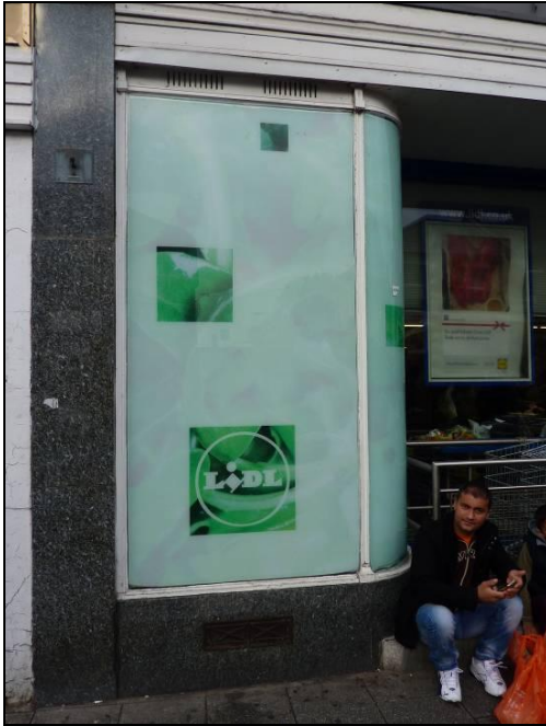
Photograph 11: 43-49 High Street, Walthamstow: close up of the western curved steel and glass shop display window.
