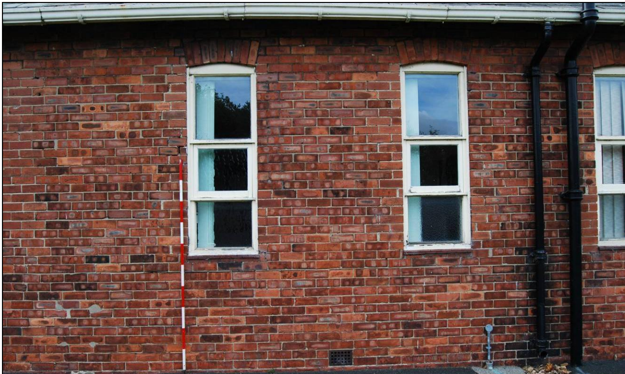
Plate 2: facing southwest showing detail of windows along the northeast elevation, with original openings, tile sills and arched brick lintels. The guttering and downpipes are modern.
