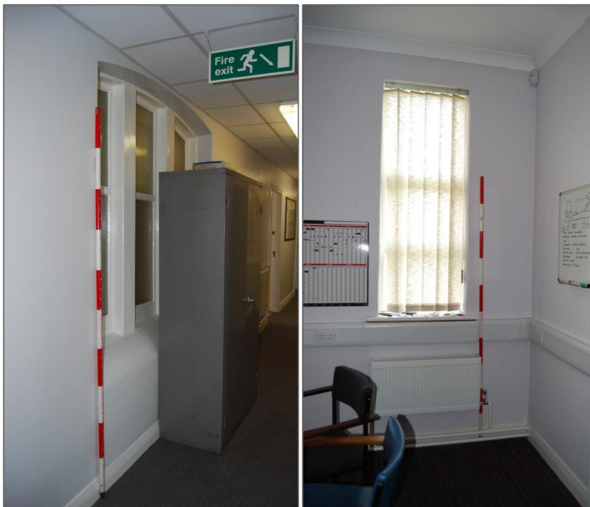
Plate 5: Left: view from 12 - the corridor (originally the veranda) with original exterior window visible between the corridor and office 4; the opening is blocked in office 4. Right: view within office 5 showing retained features: original height ceiling, cornicing and original exterior window opening.
