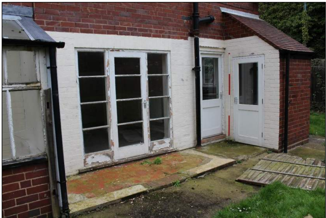
Photograph 50 – Detail shot of current and former outhouses of the south-east elevation of No. 20 Frog Lane.
