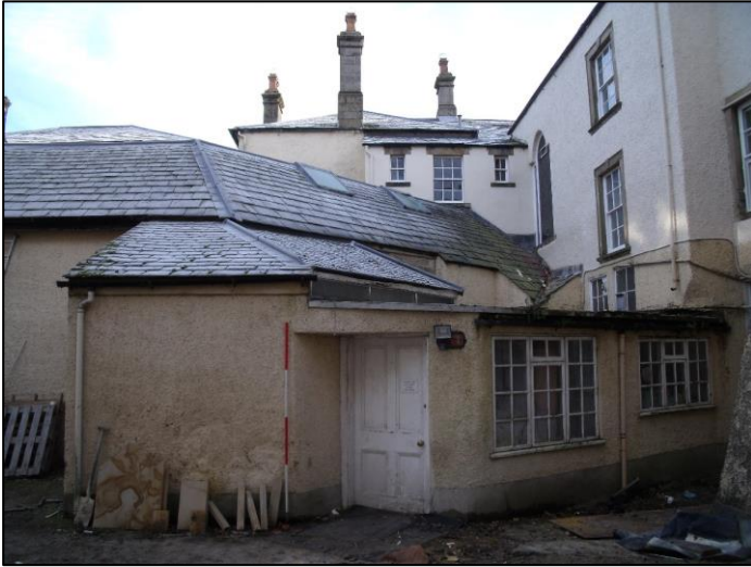
Plate 6 (left). Single storey structures in the south-east corner of the courtyard on the site of the 18 th century kitchen block. These were a mixture of mid-19 th century and later construction and alteration. These demolished as part of the consented works to allow for logistically better arrangements for access and utility.
