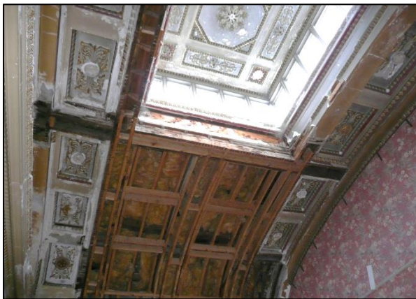
Plate 13. Room G3, (left above) Northern Atrium ceiling and clerestory under repair in 2012; (below left) West wall and fireplace under repair, not replacement column sections waiting for insertion 2012; (below right) looking north-east, room under repair, note the white plaster repair sections to the column capitals previously damaged by insertion of a 20 th century recording studio.
