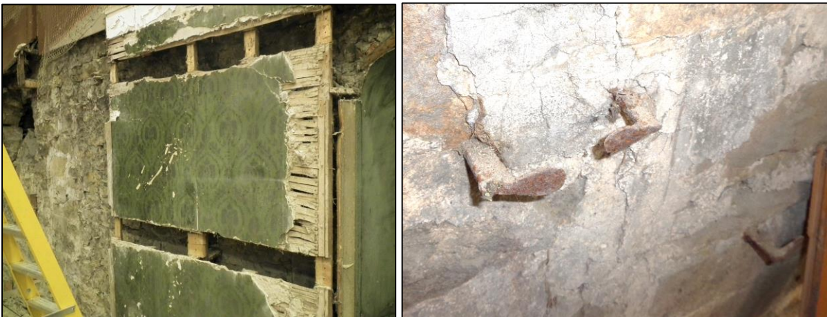
Plate 24. (above left) 19 th C lathe and plaster with decorative painted stencil work on battens attached to the former west outside wall of the 17 th century Hall. (above right) iron brackets behind the 19 th c decoration and possibly to retain some form of panelling for an earlier chapel decorative scheme.
