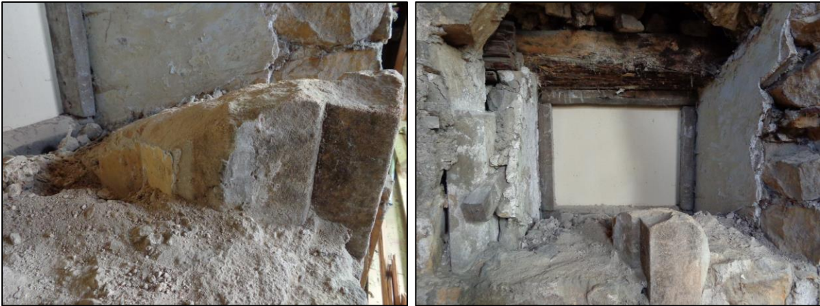
Plate 23. (above left) South side of the blocked and damaged 17 th century mullion window in the chapel's east wall showing a small fragment of early plaster with yellow ochre decoration. (above right), later rectangular insertion through the wall with wooden frame and plain white plasterwork and seemingly creating a link from the chapel to the sacristy. The creation of this opening resulted in the damage to the 17 th century mullion window which had by that point been blocked.
