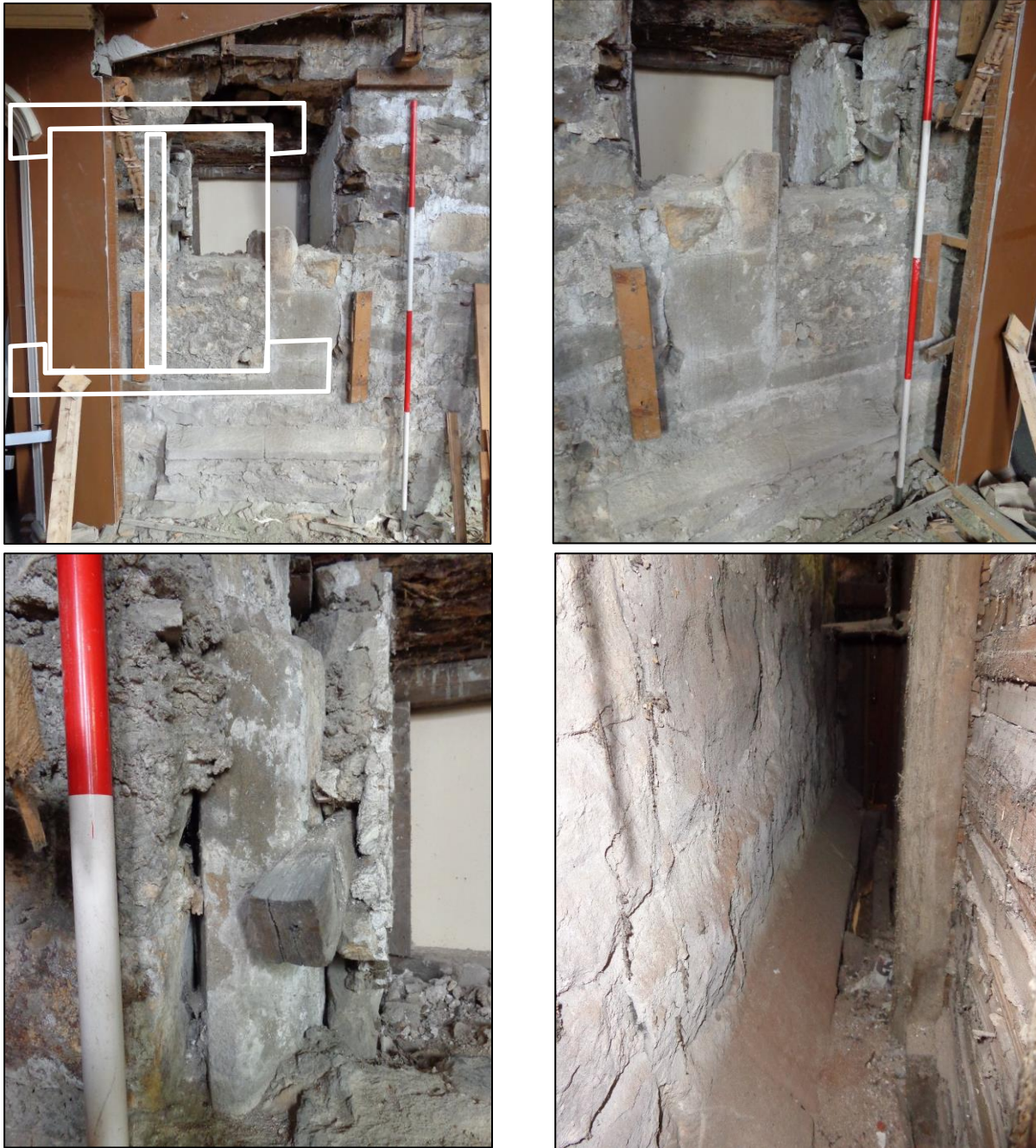
Plate 22. (Clockwise from top left) exposed but damaged two light mullion and transom window in the former west outside wall of the Hall prior to the construction of the chapel in the late 18 th century. The window and plinth course below it appear identical to those on the projecting entrance tower on the Hall's south front which is dated 1623. The outline of the window is shown in white. (top right) the same window showing the later rectangular, wood framed and plastered window opening driven through the wall. (bottom right) looking south behind the lathe and plaster 19 th century wall of the chapel and showing the 17 th century west wall of the hall and its distinctive plinth course. (bottom left) the central mullion of the blocked window with later white plaster work.
