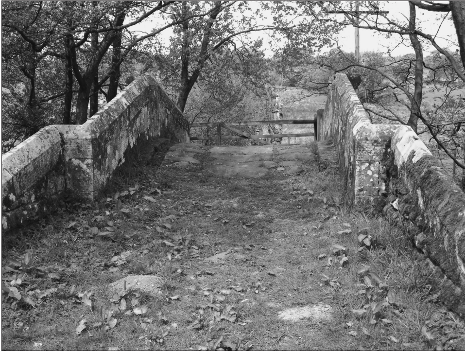
Figure 13 Looking north, paved trods over Huntersty bridge. This linked the village of Westerdale with the hamlet of Gowthorpe Green. Trods line the east side of the green. The path continues north-west and west to Baysdale, Kildale, Stokesley and Guisborough.
