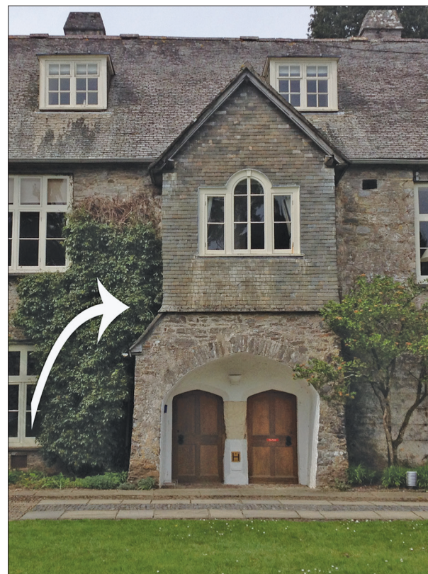
Figure 4b This image is an example of the other staircases on the west range. The stairs inclined from south to north, the opposite of the example beside the lord's chambers.
