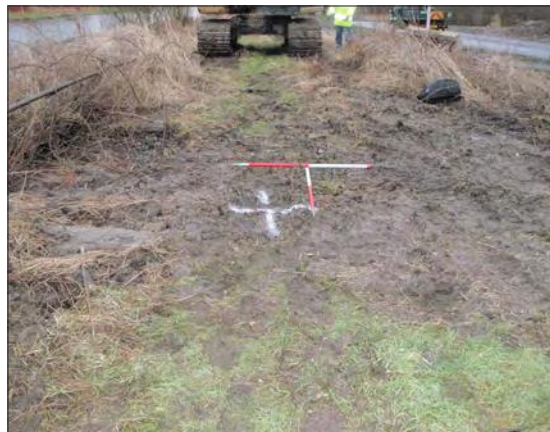
Plate 1: Pre-excitation shot of the manhole trench showing the embankment to the right and the canal edge to the left. The new access road can be seen in the top right corner.
