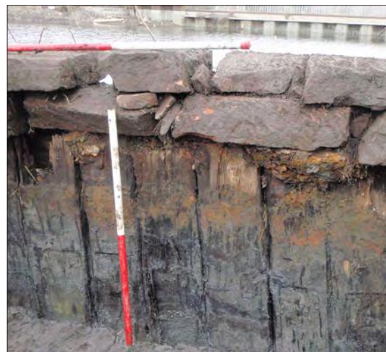
Plate 4: Grey packing clay excavated to partially expose tarred timber piles and cap stones. Shown in context, looking north over the canal.
