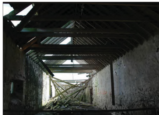
Plate 20: West end of Building 2 showing collapsed roofing.
