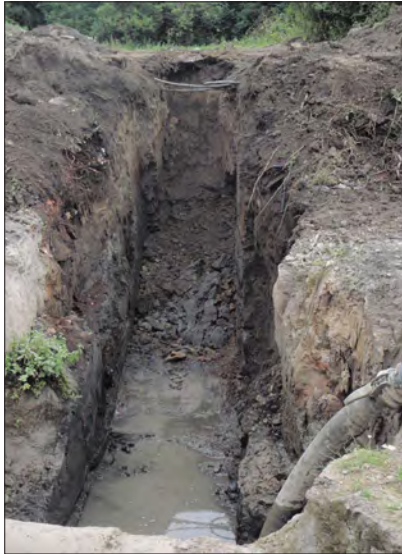
Plate 1: Working shot of pipe trench showing telecom cables and a metal service pipe (foreground).
