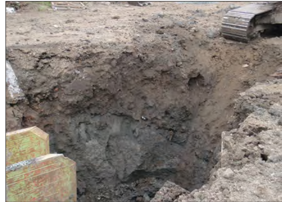
Plate 2. West facing section of pipe trench showing in-fill deposit and modern disturbance to the north canal wall.
