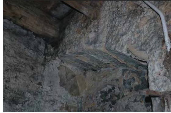
Plate 16: Detail of blocked cart arch above Room 3 interior doorway.
