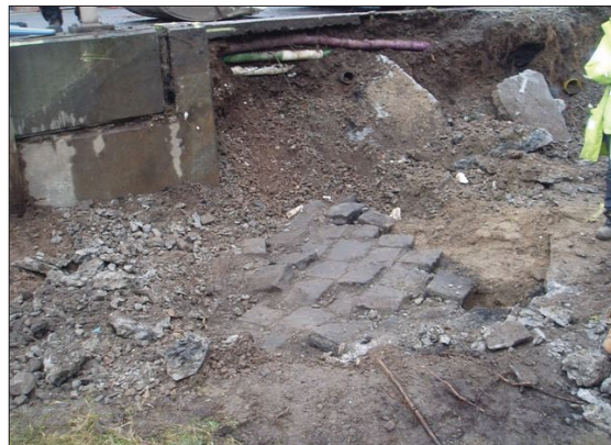
Plate 4: Cobbled surface at Victoria Swing Bridge
