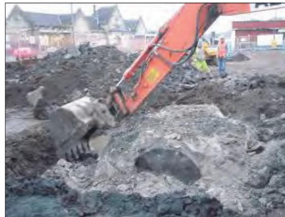
Plate 23: Concrete encased diesel tank on the site of foundation trench pad 4, probably responsible for the petro-chemical contamination across this part of the site.
