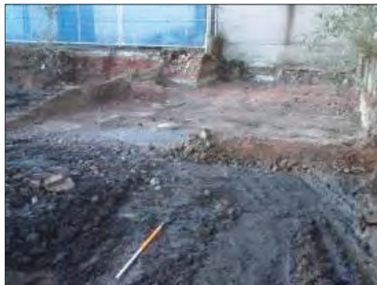
Plate 16: Concrete slab and miscellaneous truncated brick walls 1000 associated with the former Post Office Sorting Office, located along the western part of the watching brief area, from the east.
