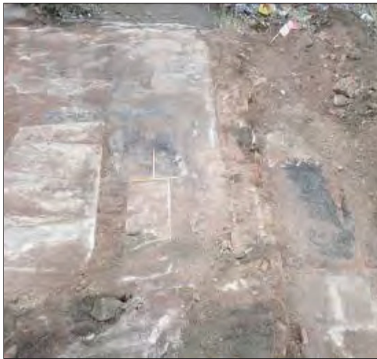
Plate 14: Demolished building remnants 1000 at the north end of the watching brief area, from the west.
