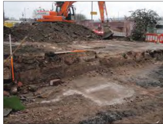
Plate 15: Wall 1007 and concrete floors 1000 at the north end of watching brief area, from the south-west.
