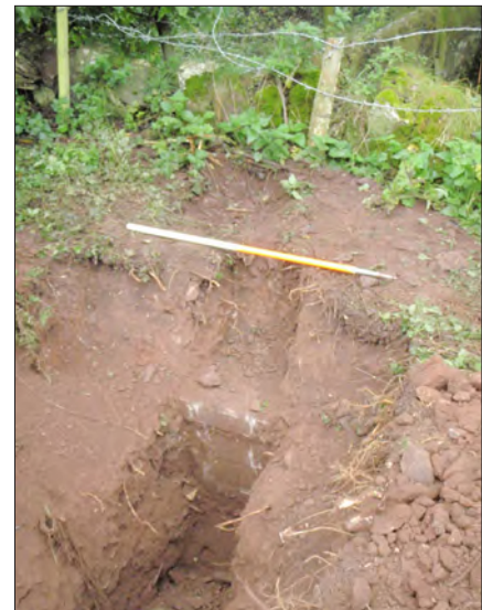
Plate 2: View of concrete beam in TH03 bracing field boundary wall, from the east-north-east.
