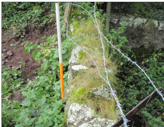
Plate 1: View immediately west of TH03 showing build up of road make-up layer 003 on the west side of field boundary wall, from the north.
