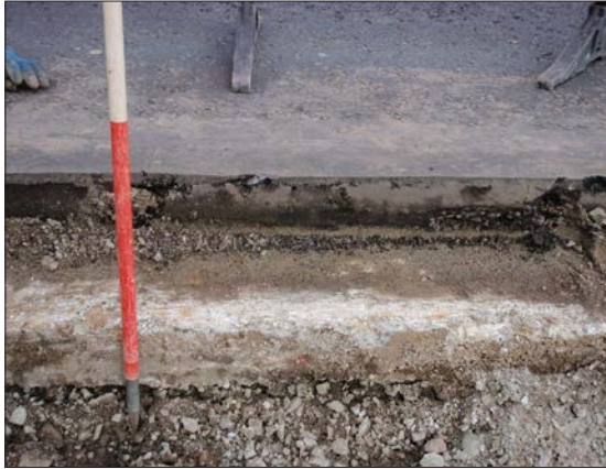
Plate 1: South facing section of cut alongside Glasgow Road, showing tarmac, hard standing, concrete and type 1.
