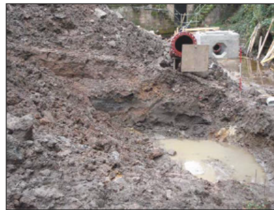
Plate 18: North-north-west facing section of the turbine base trench, water supply pipe and flood release valve top right of frame.
