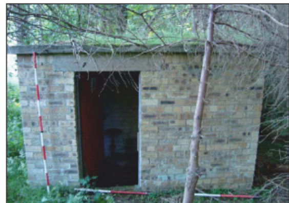
Plate 2: Building 1, from the north-east, cast-iron valve is visible on the rear wall of the building.
