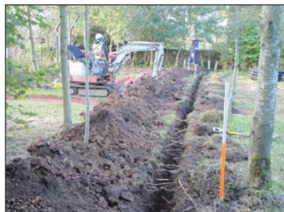
Plate 16: General view of the north-east to south-west electric cable trench in the visitor centre garden, from the north-east.
