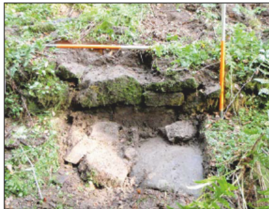
Plate 19: Bank revetting wall 1001 at the base of the bank along the eastern edge of the outfall, from the west-south-west.
