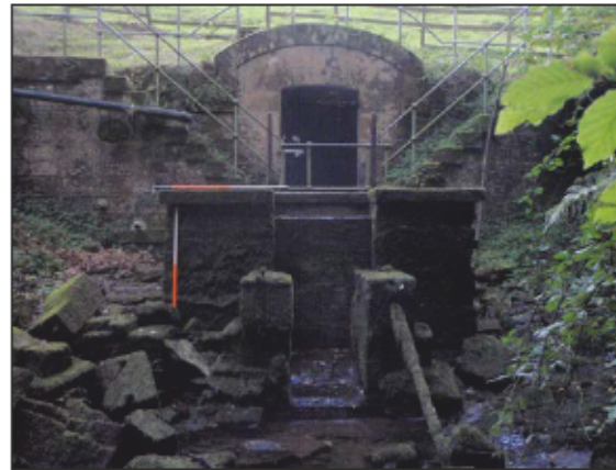
Plate 7: General view of Building 5, rubble spread left of frame may represent the site of the earlier electricity turbine. Rear of frame the sandstone wall revetting the base of the bank of the dam with a valve chamber compartment, from the north-west.
