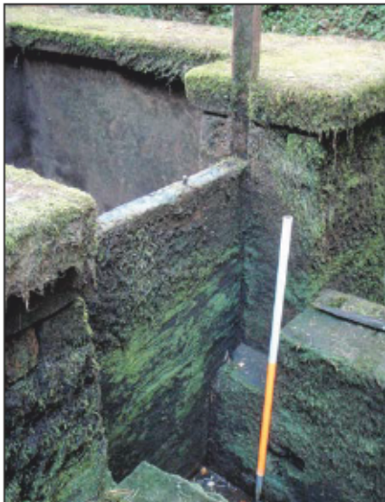
Plate 8: Detail of wooden sluice gate controlling flow of water to waterwheel mounted on projecting sandstone walls on the north side of Building 5. Part of a semi-circular scar made by the water wheel is visible to right of and below the base of the ranging rod, from the north-west.
