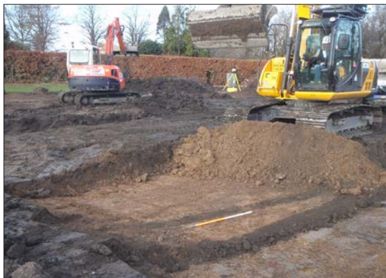
Plate 5: General view of stripping towards the south-west corner of the site, tile drain visible cutting natural sandy, gravely clay 007, from the south-east.
