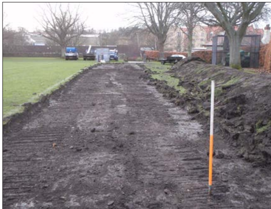
Plate 1: General view of the temporary access road after topsoil stripping, from the NNW. A fibre optic cable traverses the road from the ranging rod to the stockpile of Heras fencing in front of the parked vehicles.
