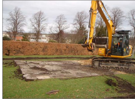
Plate 4: Concrete base of the cricket practise nets prior to removal, from the south.
