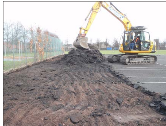
Plate 2: General view during removal of tarmac surface 003 from existing tennis courts, slag rich bedding/levelling layer 004 visible below.
