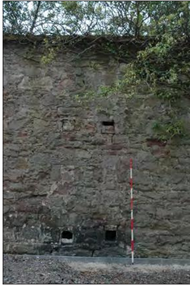
Plate 1: Square iron vents for internal heating system.
