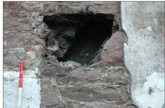
Plate 4: Detail of internal vent system.
