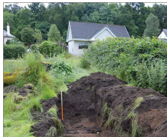
Plate 6: General view of the south-east end of Trench 2 showing the depth of infill layer 002 at this part of site.
