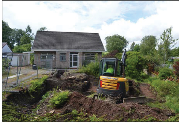
Plate 13: General view of trenches 11 and 12 on the east side of the bungalow. A service trench to disconnect the mains electric from the property excavated prior to arrival on-site is visible aligned along the right hand side of the drive and curved round to the north along the eastern property boundary.
